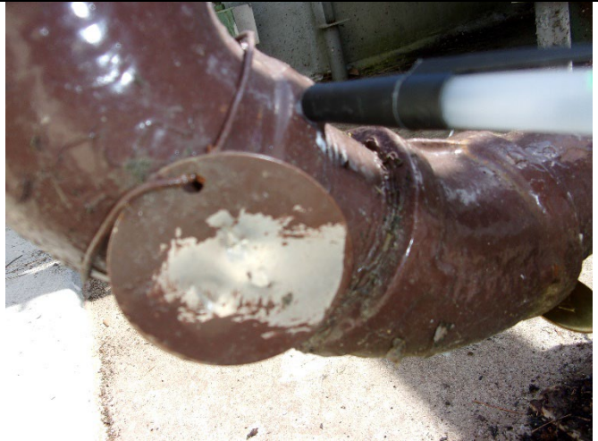
Figure 14: 10:04 AM Tank Farm Tag #4 partially illegible.
