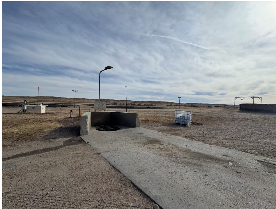
Figure 7 – Dry Creek POTW Septic Disposal Station
