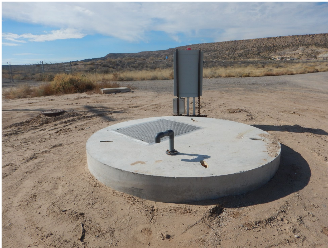
View of Lift Station (LS) WWTP#2 located approximately North and outside of WWTP fenced perimeter (DSCN1658). September 13, 2022. Photographed by D. Esparza
