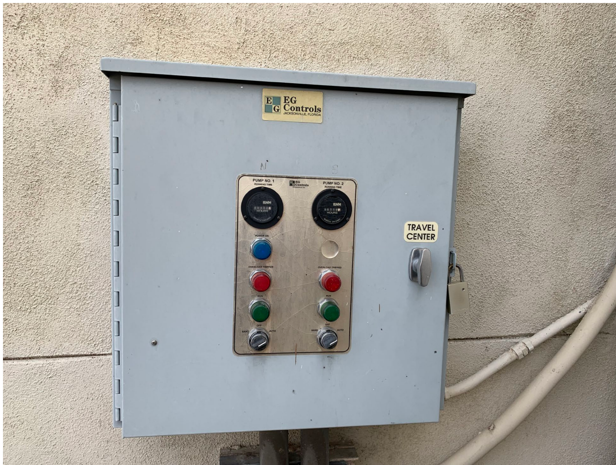
View of control panel of the Burger King Lift Station located along the West side of drive-thru next to the building. (IMG0140). September 13, 2022. Photographed by D. Esparza
