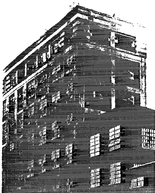
After an explosion of flour dust. Damage was confined largely to the upper floors on account of the window glass area which provided effective venting.
