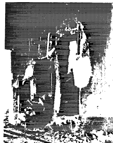
Damage to reinforced concrete bin from an explosion of grain dust. Two men were injured and property damage amounted to about $60,000.
