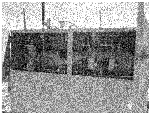
Figure 17-1 Picture of Equipment Building
