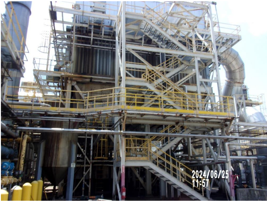
Photograph 3: Baghouses where the dust will be utilized for fuel.
