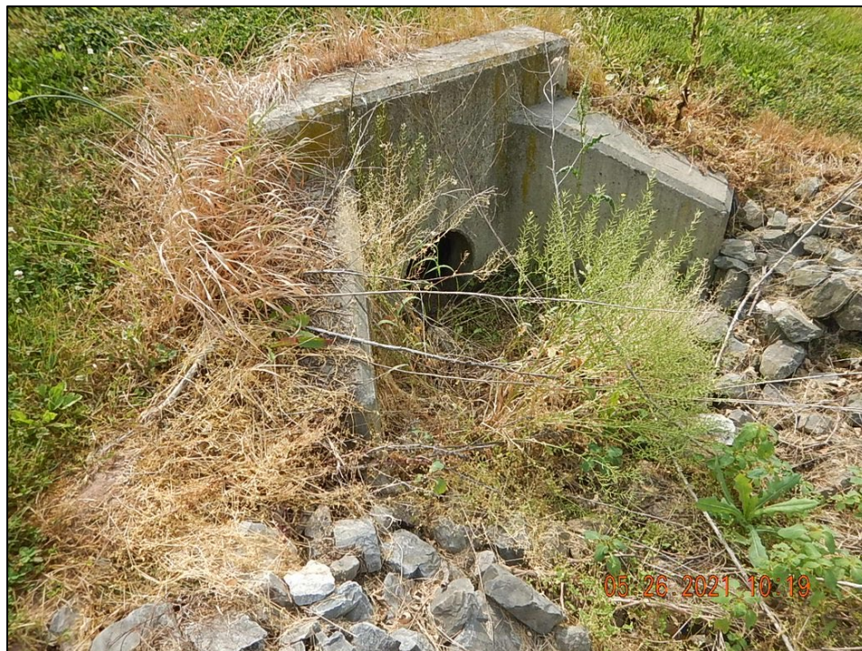
Photograph 18. Randall Drive Detention Basin: (DSCN5111) Closer view of Photograph 17, of the outlet structure for the detention basin. Note the excess vegetation in and around the structure.
