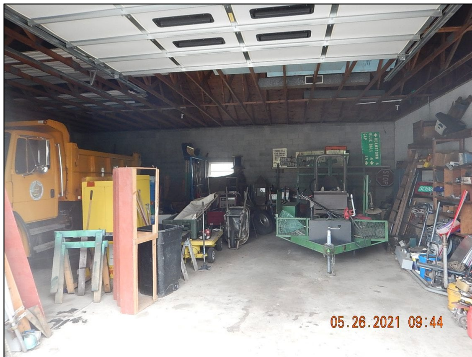
Photograph 4. Municipal Garage: (DSCN5088) View inside one of the main enclosed garages that stores vehicles and tools. No floor drains were installed in this building.
