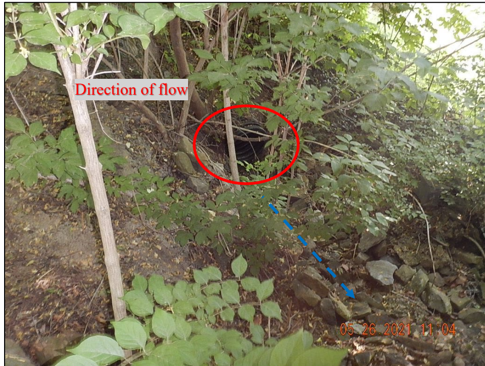
Photograph 33. Memorial Park Rain Garden #3: (DSCN5148) View of the overflow outlet pipe from Rain Garden #3 and the stormwater tank. The channel leads to Outfall 025.
