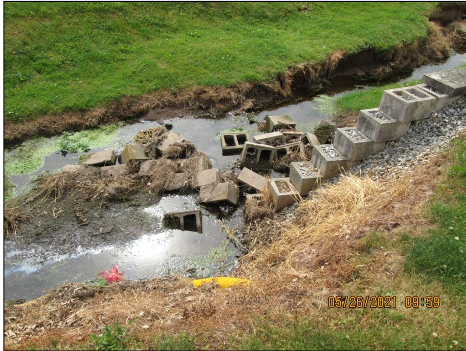
Photograph 13. Outfall #12: (IMG_1797) View, facing east, of cinder blocks in the channel upstream of the outfall. These materials originated from the adjacent private property's retaining wall.
