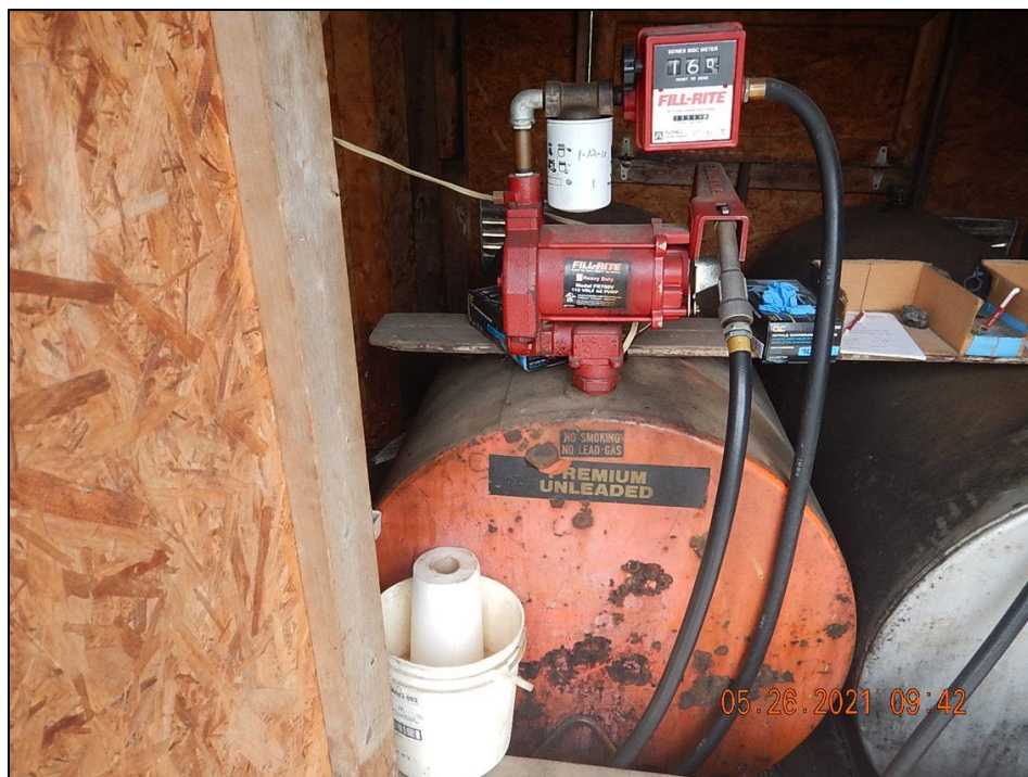
Photograph 2. Municipal Garage: (DSCN5084) Closer view of the aboveground unleaded fuel storage tank from Photograph 1. Note the bucket of absorbent material next to the tank.
