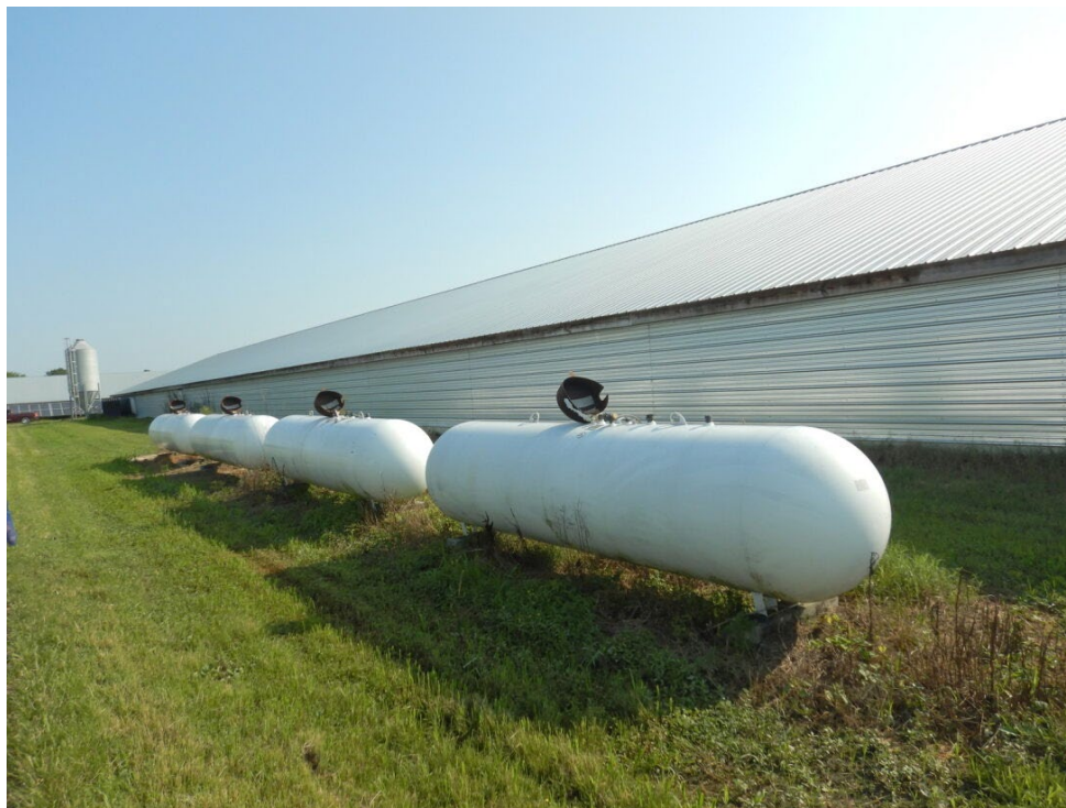
Photograph 31. View of fuel tanks between Poultry Houses 3 and 4.
