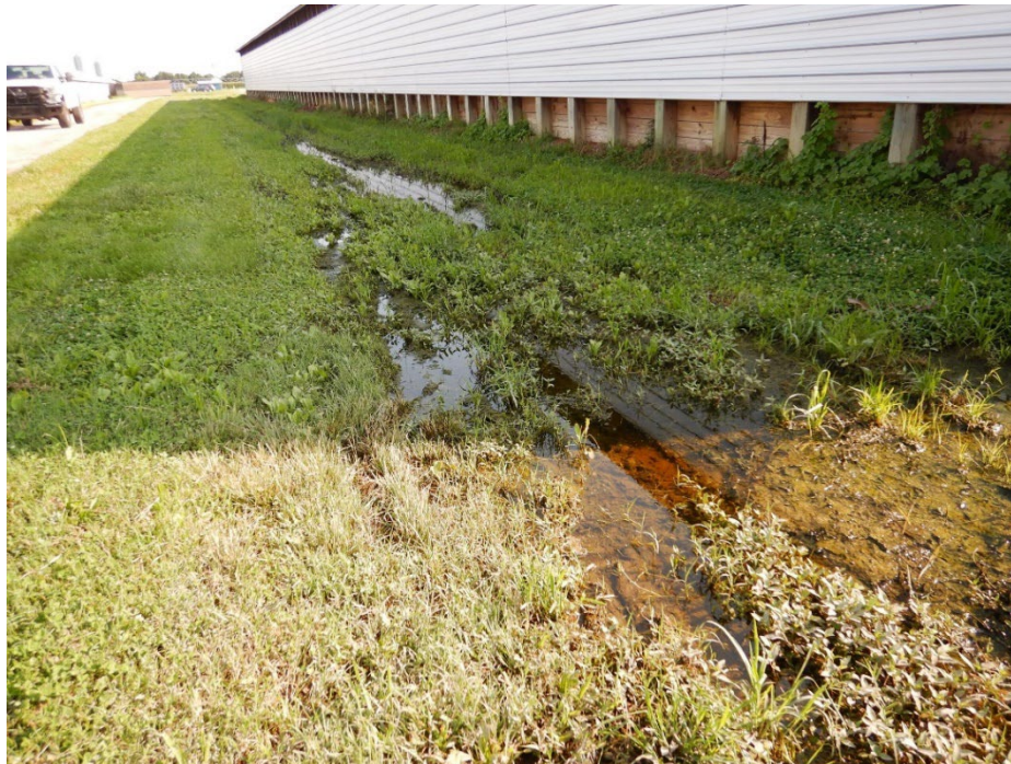
Photograph 16. Alternative view of the stormwater drainage and standing water shown in Photograph 15. The inspection team observed discoloration in the standing water.
