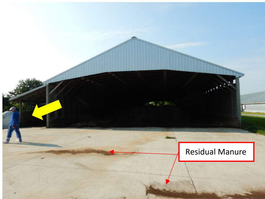
Photograph 10. View of the southern manure storage building and the concrete pad at the northern end of the building. Residual manure was observed on the concrete pad (red arrows). Mortality composting is performed in the composter located on the eastern edge of the building (yellow arrow).
