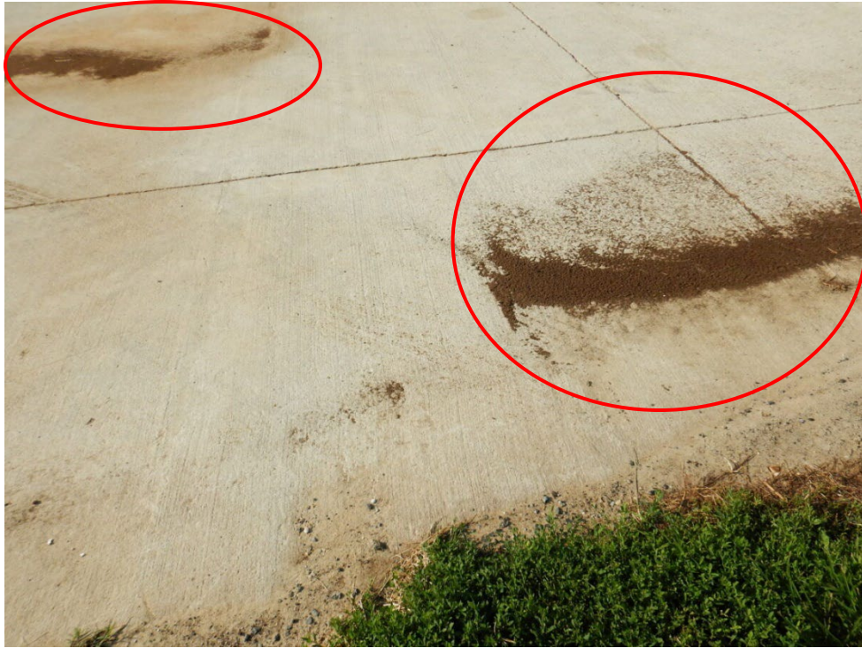
Photograph 11. Close-up view of the residual manure (red circles) on concrete pad on north end of the southern manure storage building.
