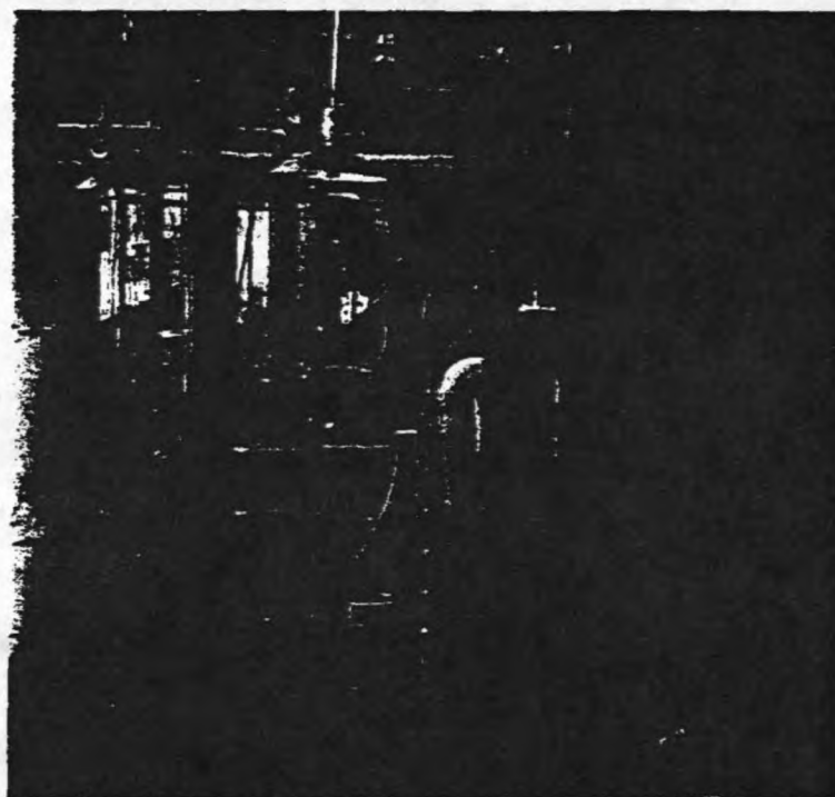
This photograph shows the line of Elliott turbine-driven single-stage blowers serving continuous filters in the Carlsbad plant. There were nine Elliott turbine-driven blowers at the time this picture was taken, with two more on order. The blowers are each rated 12,640 cfm, with an inlet pressure of about 3.5 in. absolute, discharging to atmosphere (barometer 26.5 in.) and are driven at 3670 rpm by Elliott steam turbines of about 160 hp.
