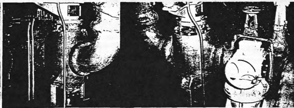
These Elliott 12-in. self-cleaning strainers are located in the take-off lines from No. 1 and No. 2 main penstocks to raw water header. They each handle 1300 gpm. One strainer is located on either side of a rotary control valve which separates the two main penstocks.
