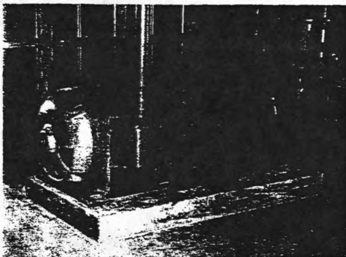
This Elliott Crocker-Wheeler 75-hp, 1800-rpm motor drives a 1000-gpm relay pump, used to relay water from a large storage basin to the main plant reservoir.
