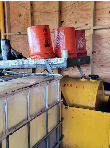
Photo #7 – Maintenance Area – used oil transfer containers and filter.
