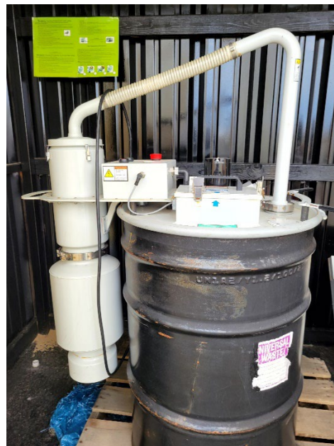
Photo #4 – 55-gallon container of bulb crusher in the outdoor environmental area.
