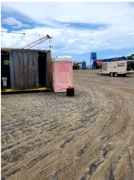
Photo #3 – Spent blast media release On the ground.
