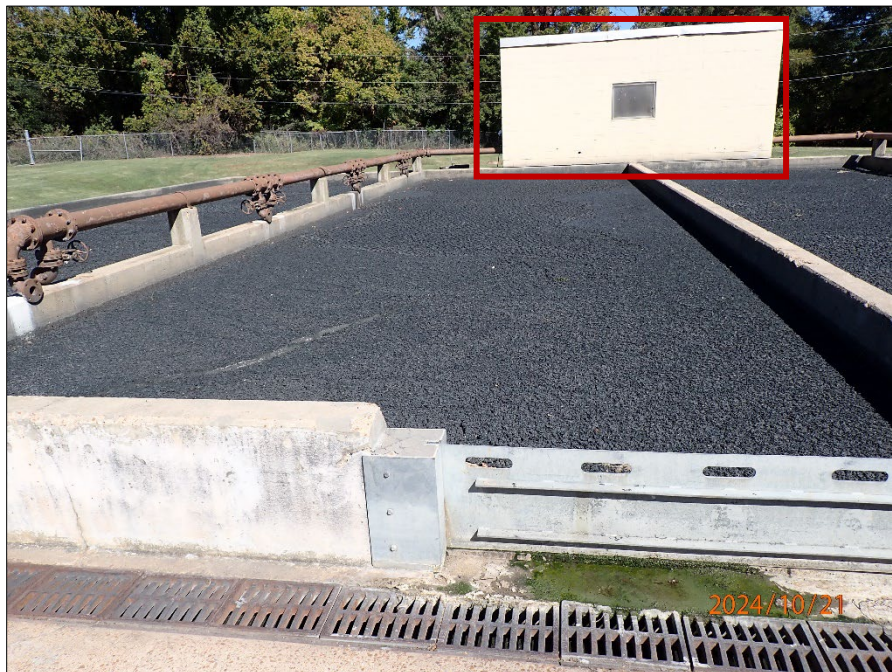
Photograph 48. Sludge drying beds with the water and polymer storage shed, outlined in red by the inspectors.
