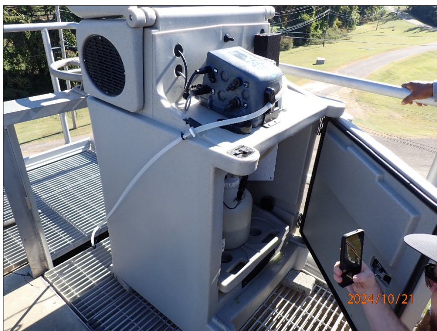
Photograph 10. Influent auto sampler located immediately after the fine screen process.
