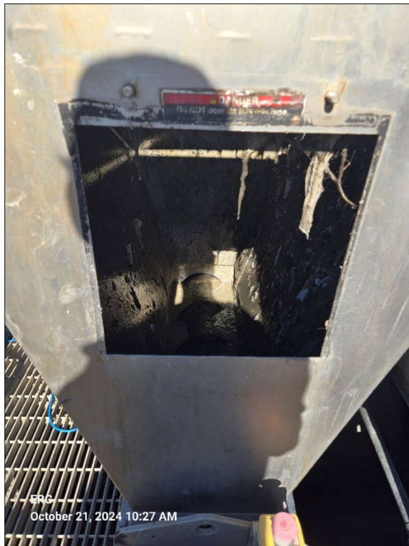
Photograph 8. Solids disposal chute for the fine screen.
