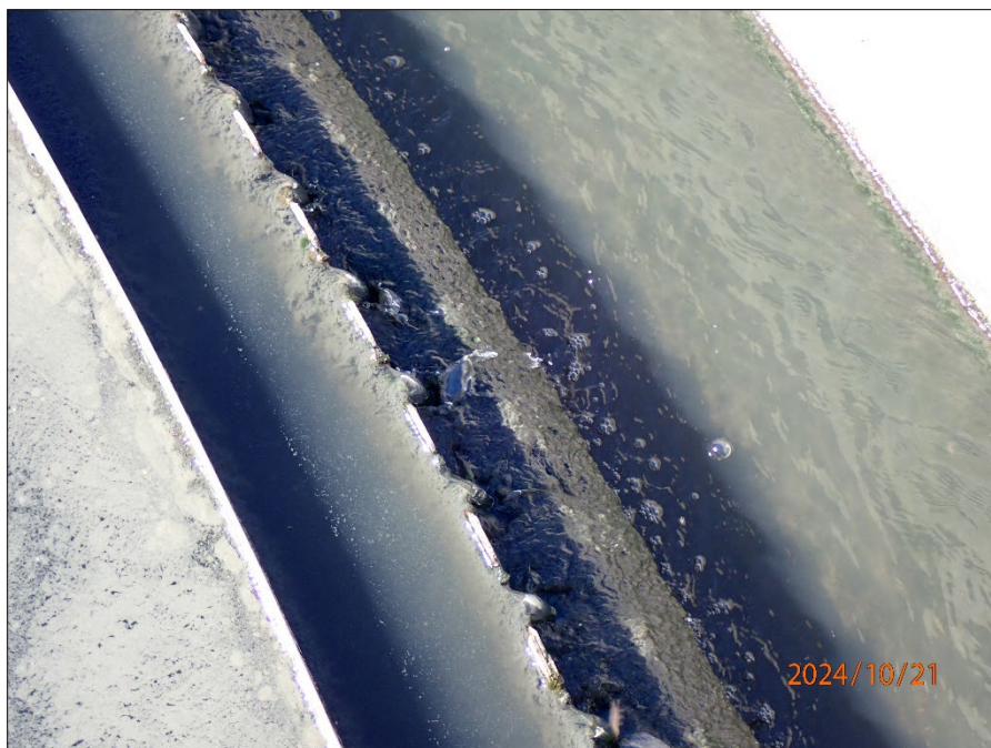
Photograph 25. East secondary clarifier weir. Note the suspended solids in the effluent from the secondary clarifier.
