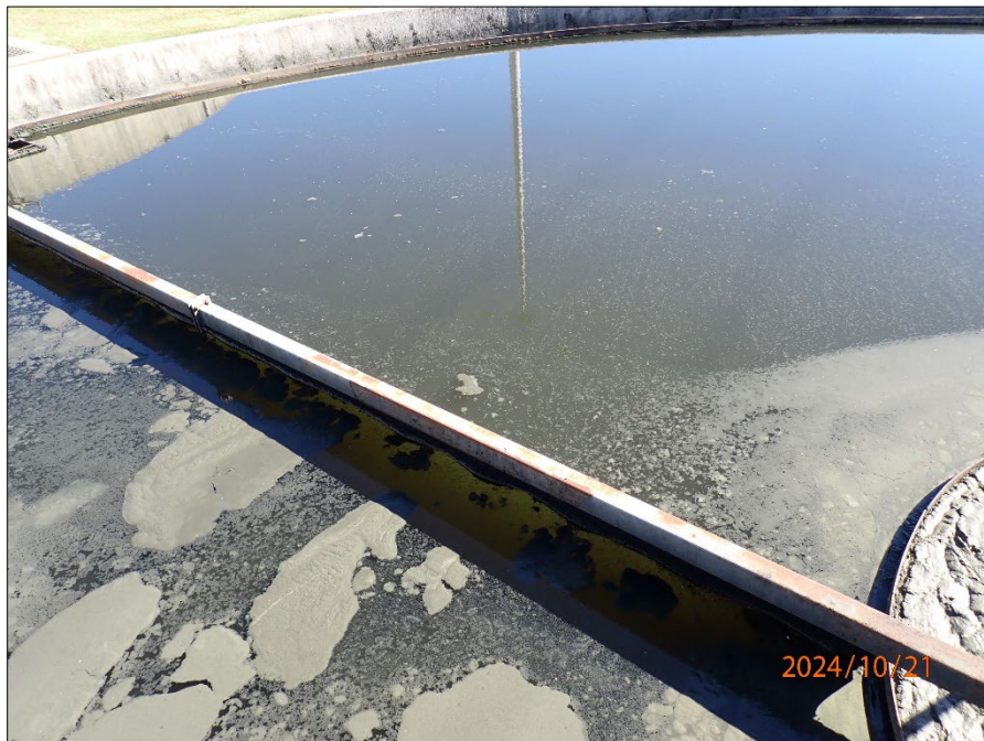
Photograph 28. East secondary clarifier surface and skimmer arm. Note the excessive solids accumulation on the surface of the secondary clarifier.
