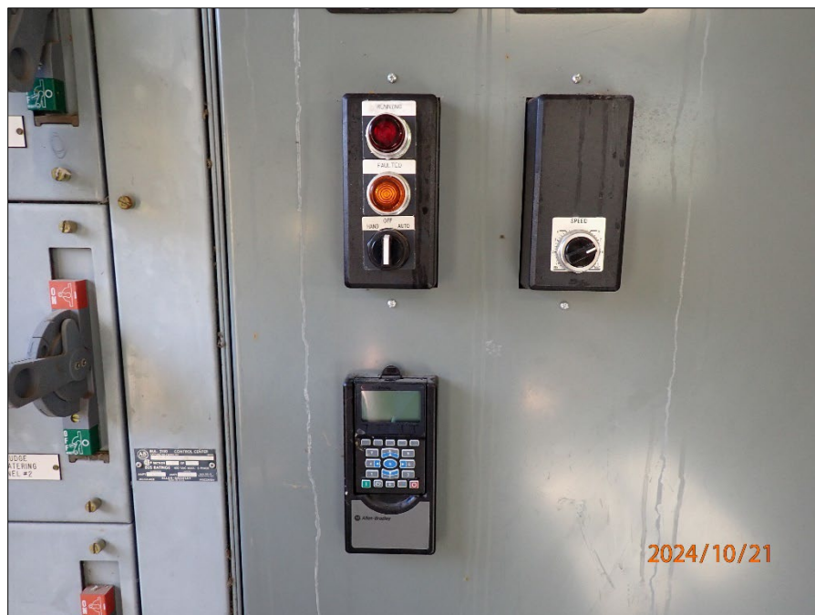
Photograph 2. Control panel for one of the three influent grinder pumps.
