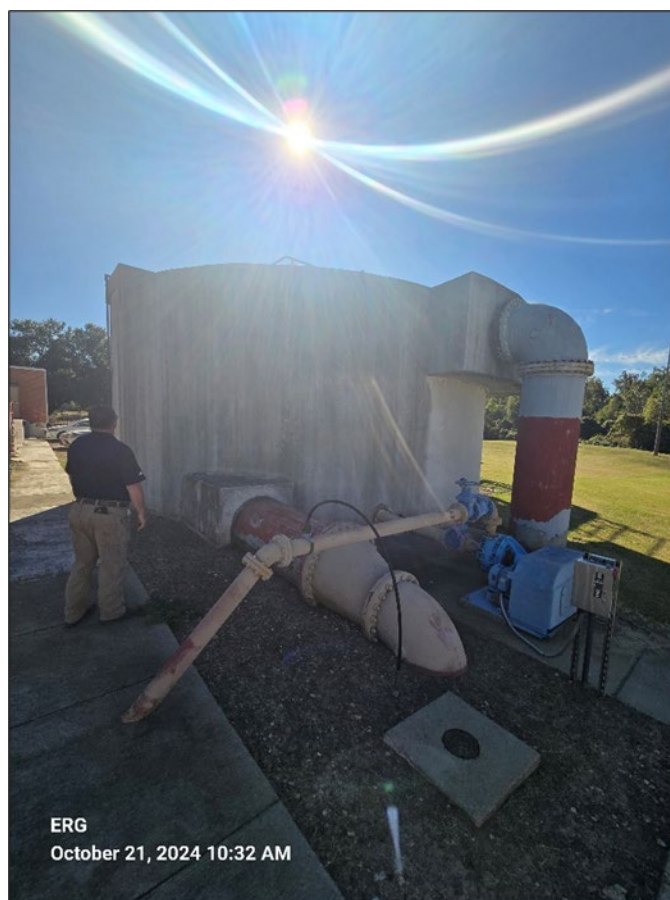
Photograph 12. Grit removal system.
