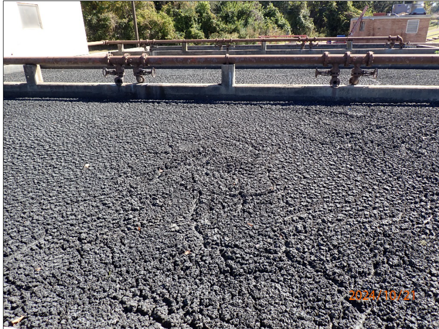
Photograph 49. Sludge drying beds. Note the drying beds are nearly at capacity.
