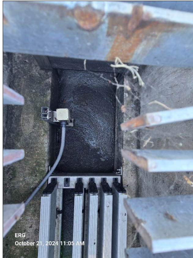
Photograph 35. UV disinfection system contact chamber. Note the floating solids in the wastewater.
