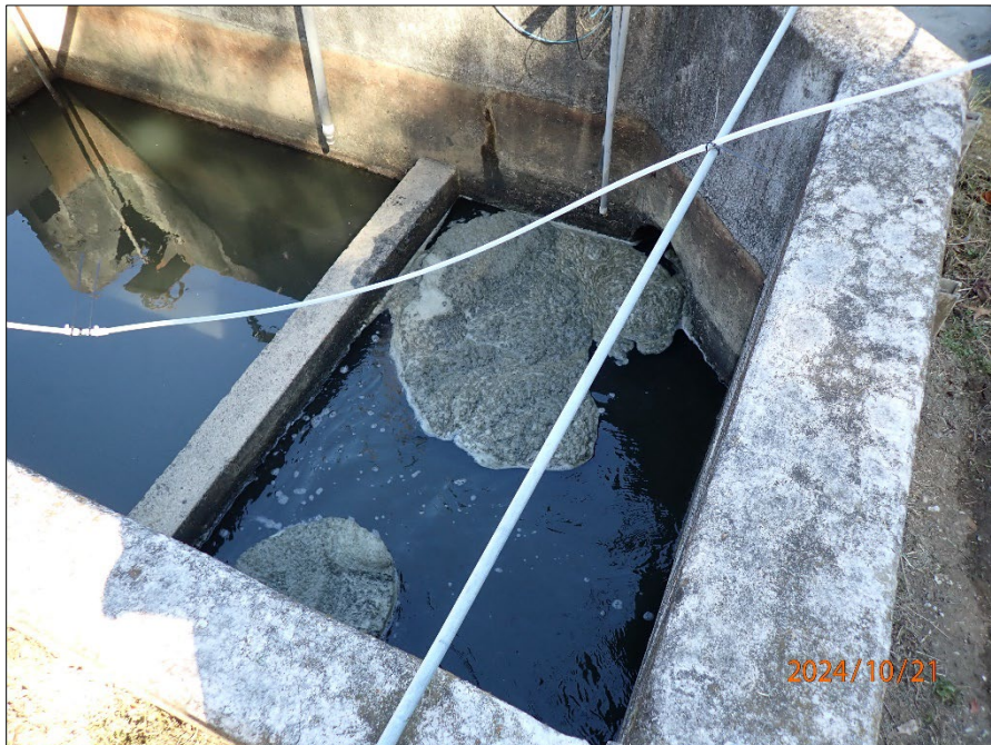
Photograph 36. Baffle located at Outfall 001, prior to flowing over the effluent weir. Note the foam on
