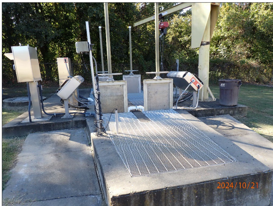
Photograph 30. UV disinfection system.
