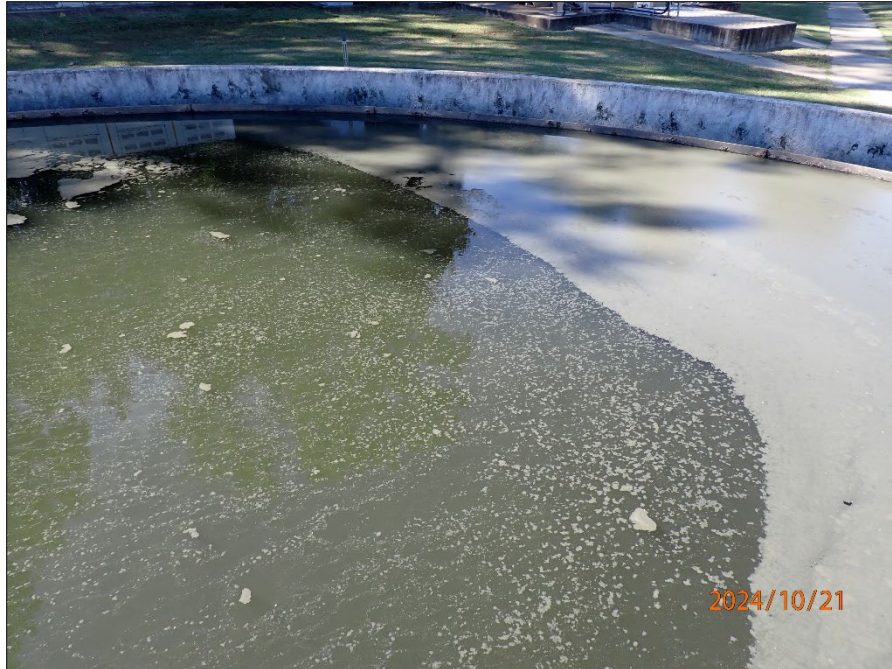
Photograph 27. East secondary clarifier. Note the excessive bulking solids accumulation on the surface of the secondary clarifier.
