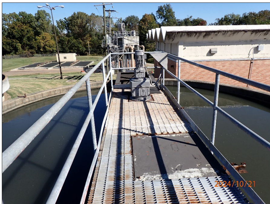
Photograph 15. East primary clarifier.
