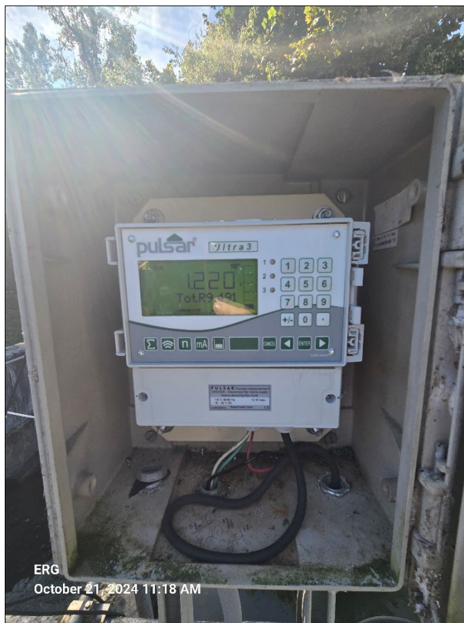
Photograph 40. Outfall 001 effluent flowmeter.
