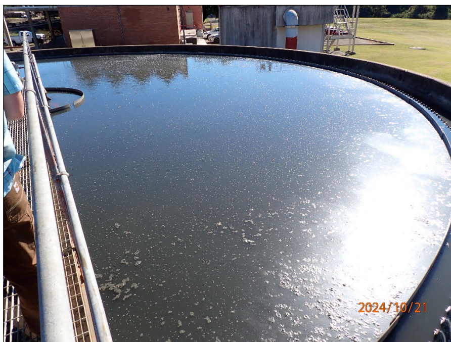
Photograph 16. Surface of the east primary clarifier. Note the air bubbles on the surface of the primary clarifier.
