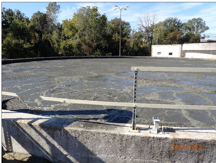
Photograph 19. East aeration basin.
