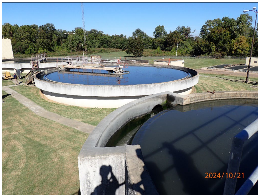
Photograph 14. East and west primary clarifiers.
