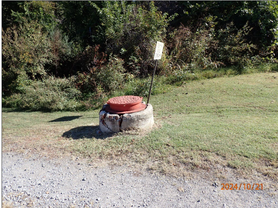
Photograph 5. Septic hauling discharge manhole with cracked concrete around the perimeter.
