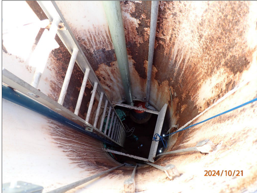
Photograph 23. Aeration basin pumps wet well access ladder. The inspectors did not observe any confined space warning signs in or around the access ladder.
