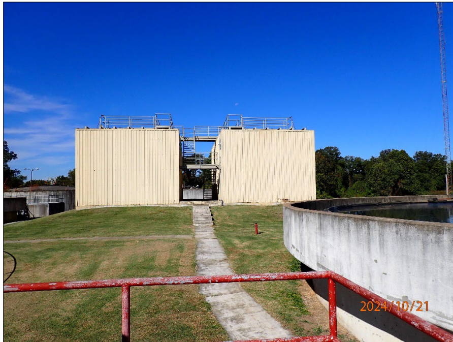
Photograph 42. Two out of service bio-cells.
