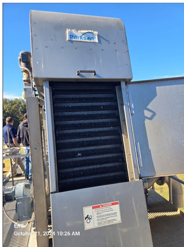
Photograph 7. Fine screen at the headworks.
