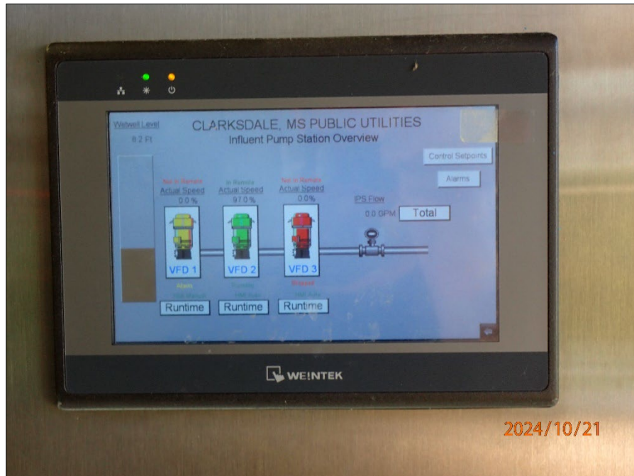
Photograph 3. Influent grinder pumps control system display.
