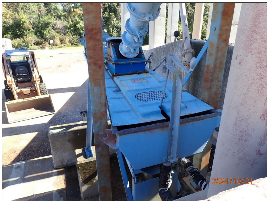
Photograph 13. Grit removal system solids disposal line. The solids are transferred to a dumpster for disposal.
