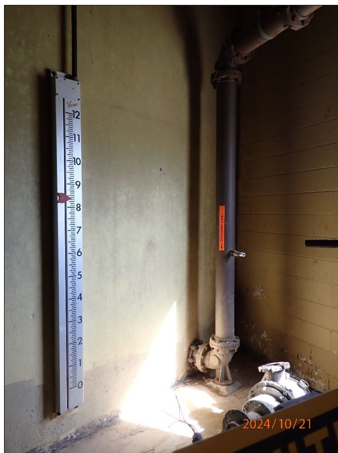
Photograph 46. North anaerobic digester sludge level measurement.
