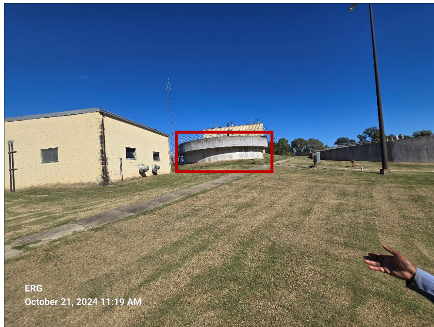
Photograph 41. Out of service trickling filter, outlined in red by the inspectors.
