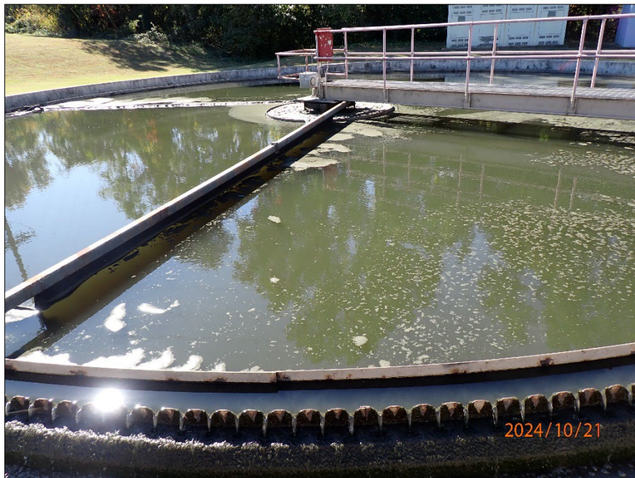
Photograph 24. East secondary clarifier and skimmer arm.
