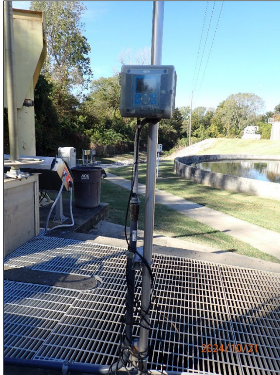
Photograph 33. UV transmittance meter. Note that the transmittance meter was out of service at the time of the inspection.
