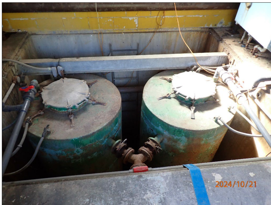
Photograph 50. Water tanks are in a shed near the sludge drying beds. The water is added to the sludge prior to being piped to the drying beds.
