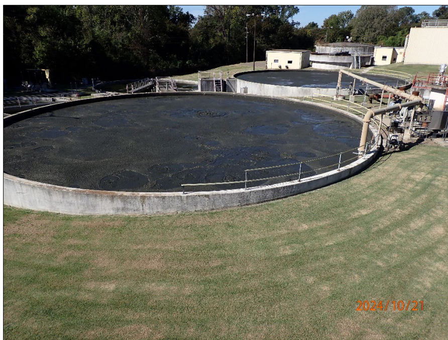
Photograph 18. Two aeration basins.
