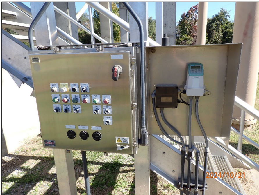
Photograph 6. Fine screen control panel.
