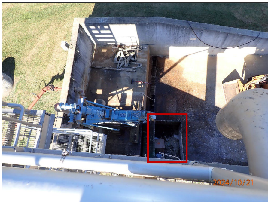
Photograph 9. Fine screen and grit removal solids disposal location. The red outline is added to identify the solids disposal dumpster.
