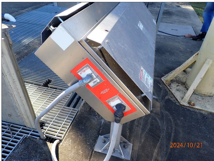
Photograph 31. UV disinfection system.
