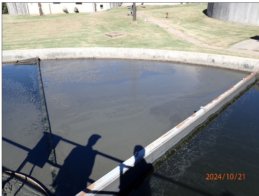
Photograph 29. East secondary clarifier surface and skimmer arm. Note the excessive solids accumulation on the surface of the secondary clarifier.
