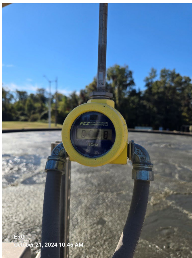
Photograph 20. East aeration basin air flowmeter.
