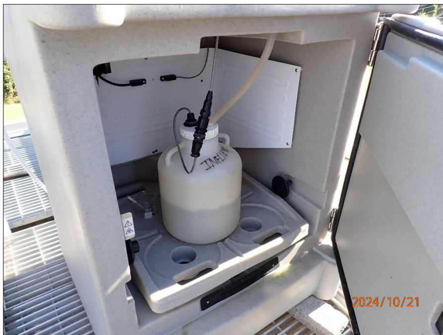
Photograph 11. Inside of the influent auto sampler.
