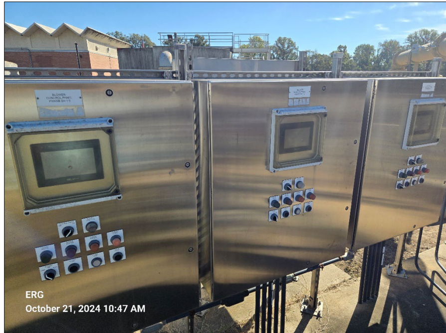
Photograph 21. Aeration basin blower control panels. Note that there are three control panels but that the facility only had two blowers at the time of the inspection.
