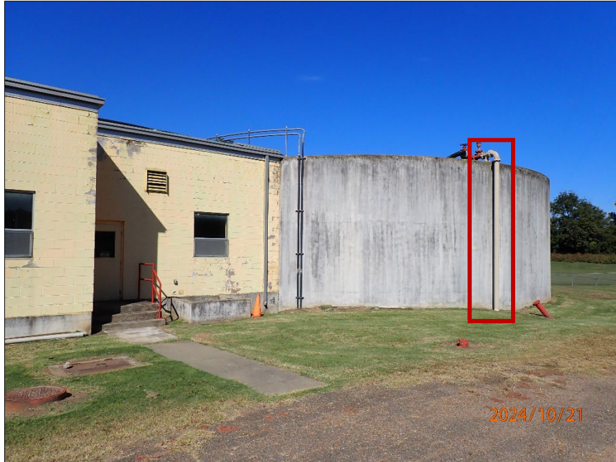
Photograph 43. North anaerobic digester. Note the sludge line to the sludge drying beds, outlined in red by the inspectors.
