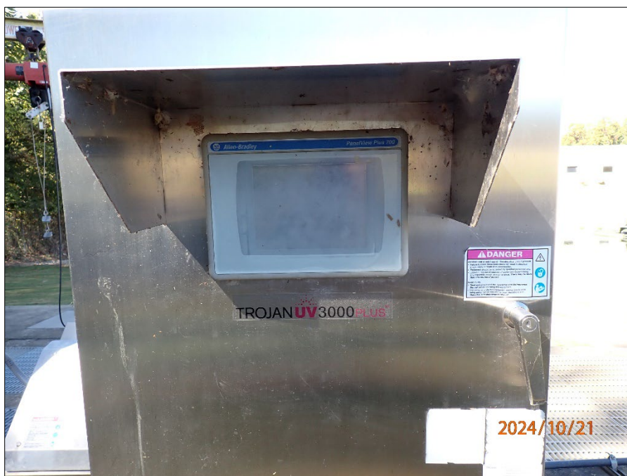
Photograph 32. UV disinfection system control panel. Note that the screen was inoperable at the time of the inspection.
