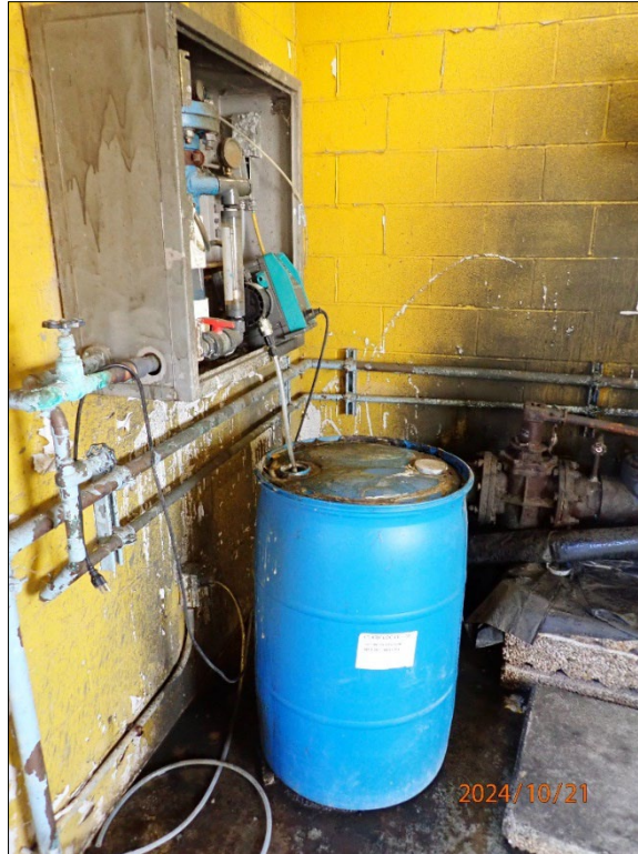
Photograph 51. Polymer drum located in a shed near the sludge drying beds. The polymer is added to the sludge prior to being piped to the drying beds.
