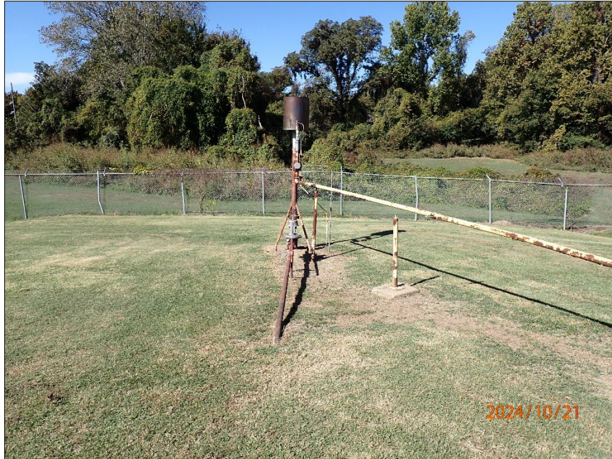
Photograph 47. Gas flare line for the anaerobic digesters. Note the flare was offline at the time of the inspection.
