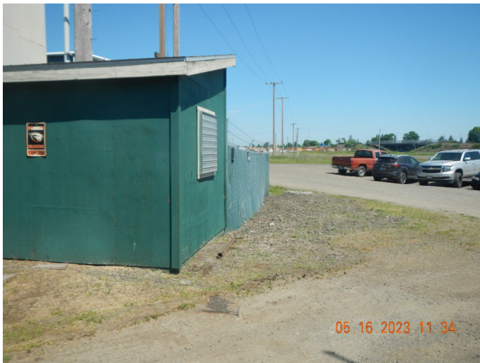
Photo #:11 (DSCN3266) Description: Facing north, photo of observed catch basin not on SWPCP Map.
