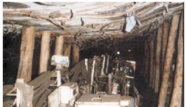
Mining conditions associated with adverse horizontal stress effects (Australia).
