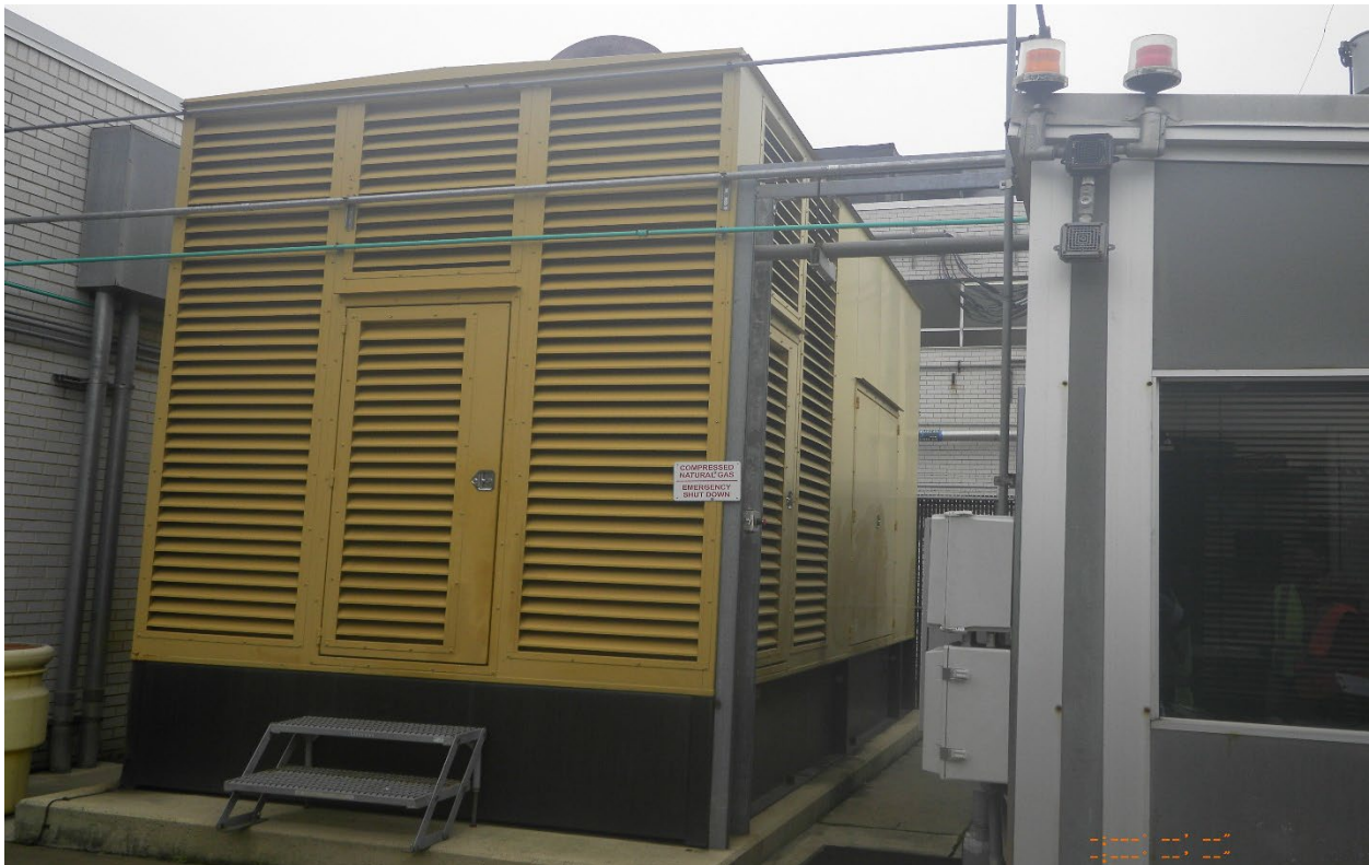
2. EG5: 1,500kW Caterpillar Generator – WMATA Bladensburg – 10/25/22
