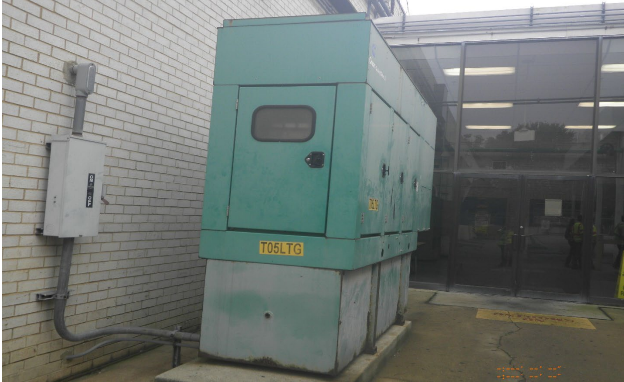
1. EG4: 200kW Cummins Generator – WMATA Bladensburg – 10/25/22
