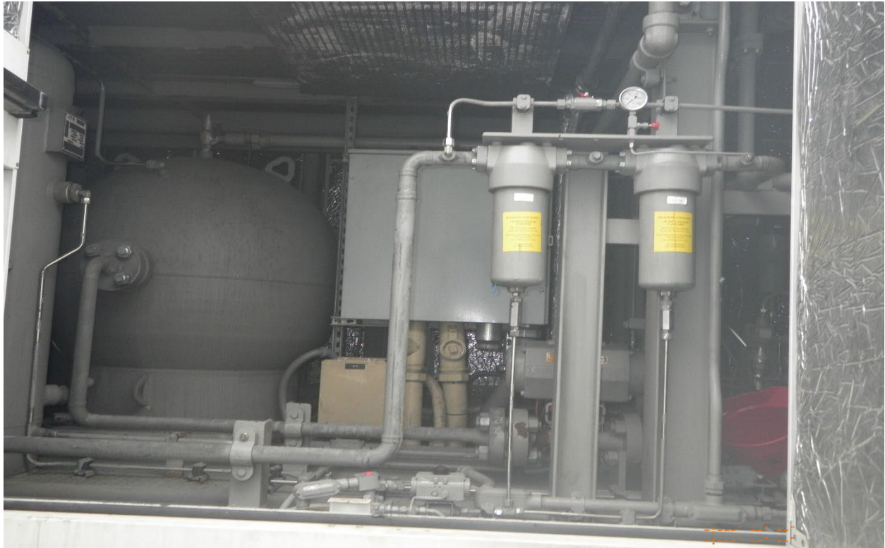
3. Natural Gas Compressor B – WMATA Bladensburg – 10/25/22
