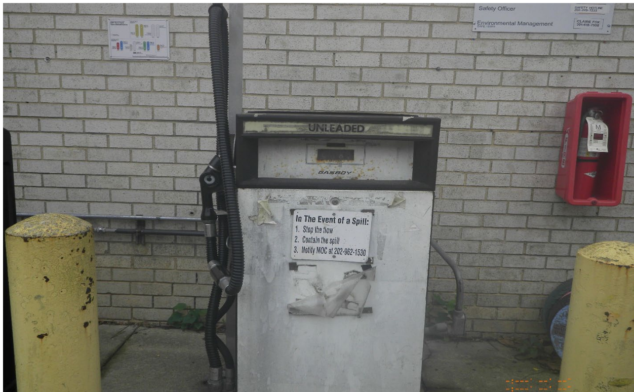
10. Gasoline Fueling Pump – WMATA Bladensburg – 10/25/22
