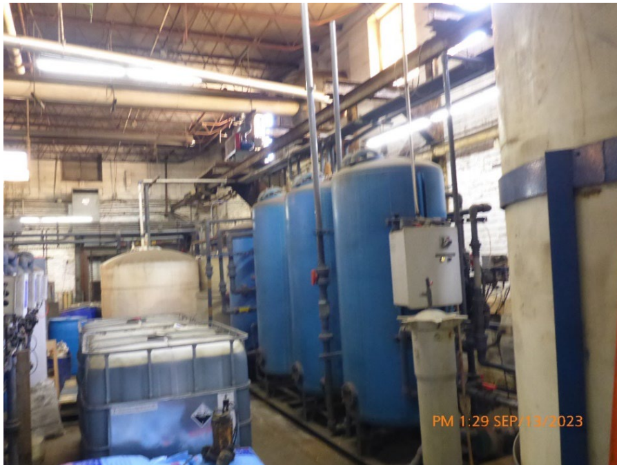
Photograph 8: Recirculation tanks (cation exchange) for chrome rinse water at American Tinning.
