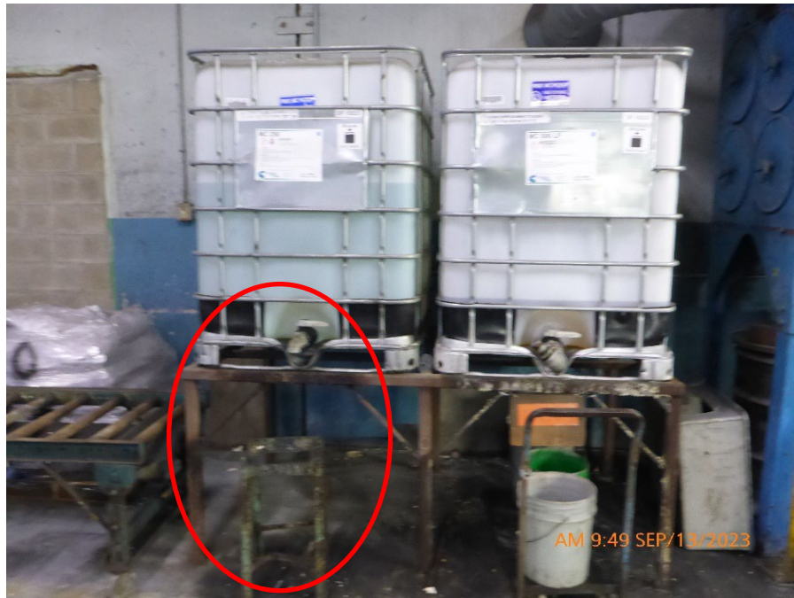
Photograph 5: Chemical storage concern at PHB: Left tote is missing catch bucket.
