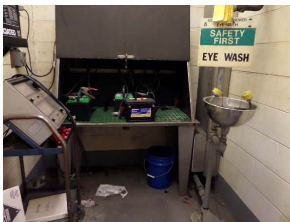
Picture 3: Battery Charging Room
