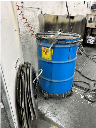
Photo-1 1–3-ton Paint Booth SAA
