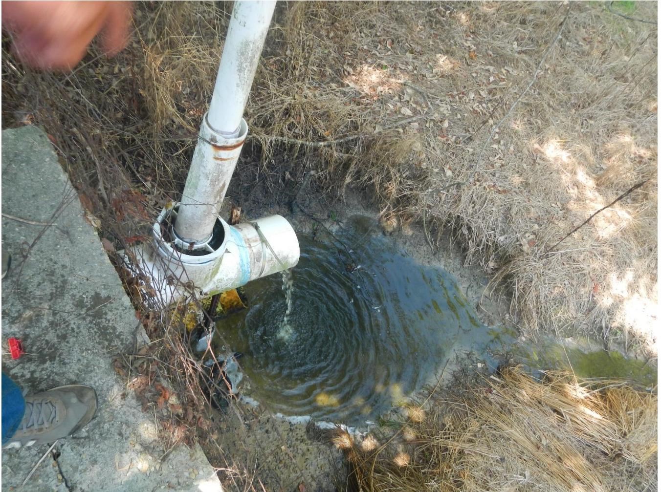
Figure 1. Effluent discharging directly from the chlorination chamber and not through pipe to permitted discharge point.
