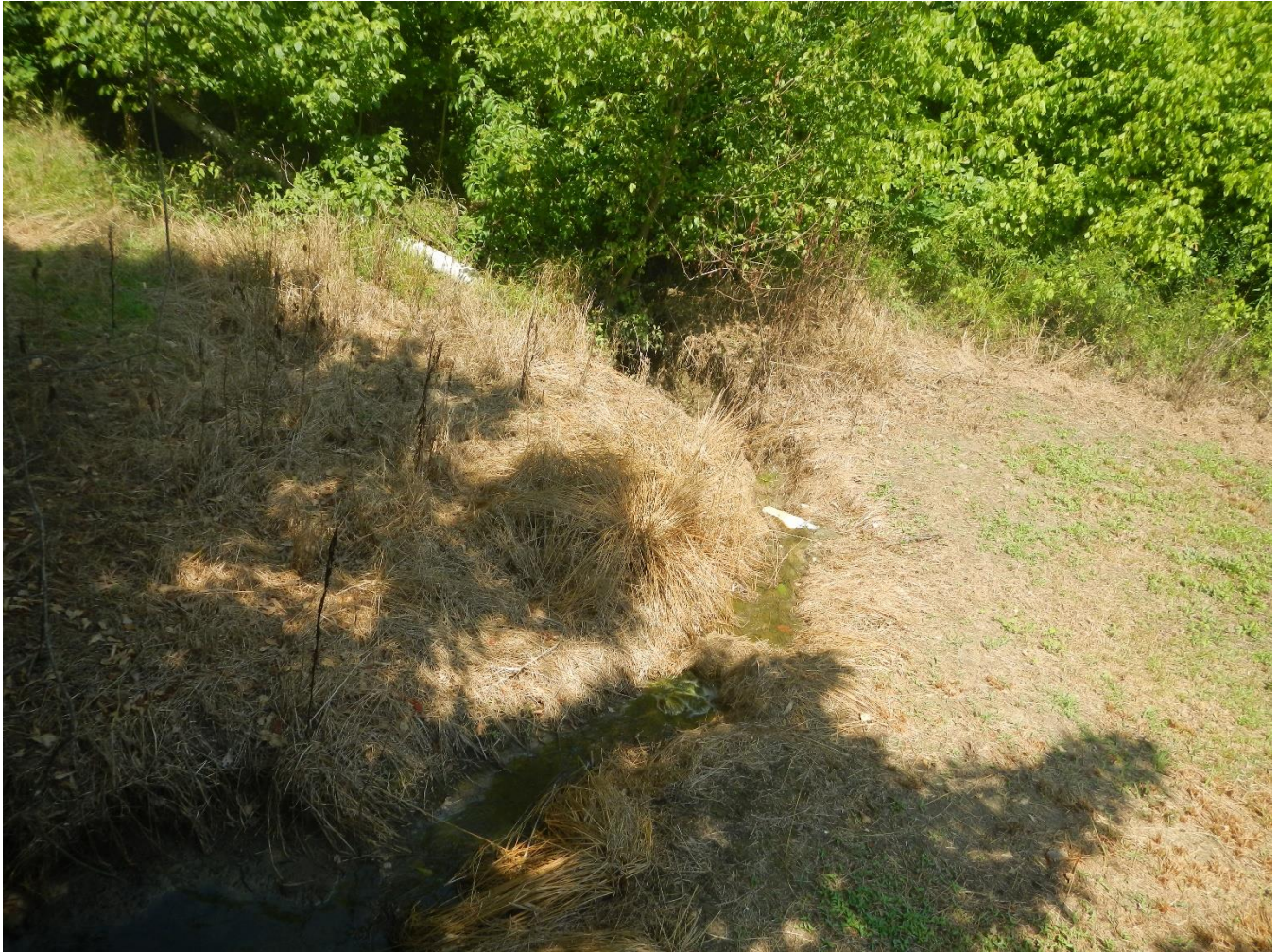
Figure 2. Disassembled effluent pipe shown below the trees. A ditch in the foreground was made by erosion as effluent discharges from a higher point.
