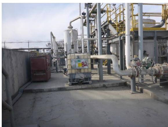
Photo 18: Tote containing approximately 100-gallons of hazardous waste carbon water in the Carbon Vent System Area at Area 5100.
