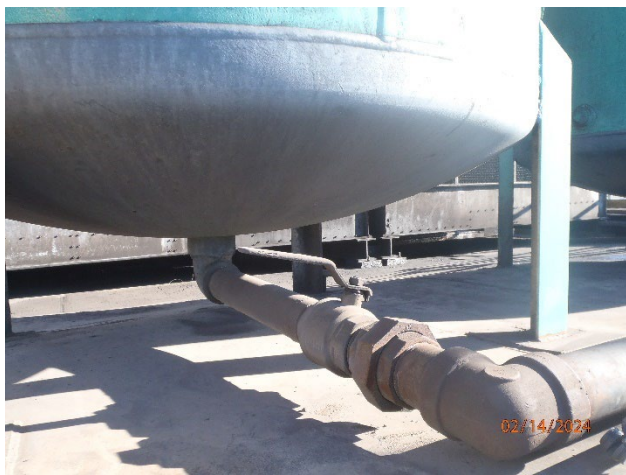
Picture 2 – Roll Mill Used Oil Tank drain structure to skimmer
