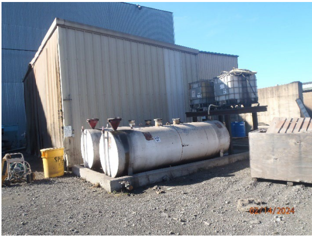
Picture 13 – Melt Shop Used Oil Storage
