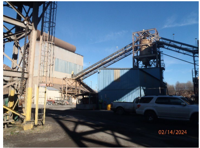
Picture 4 – Furnace Baghouse and Silo
