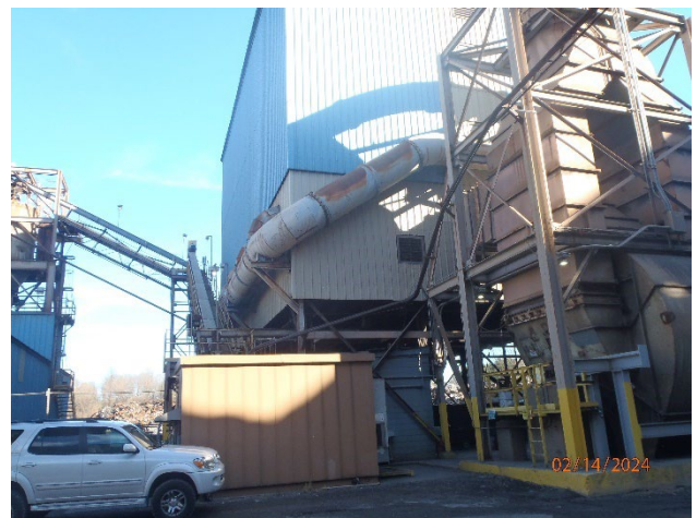
Picture 5 – Caster Baghouse
