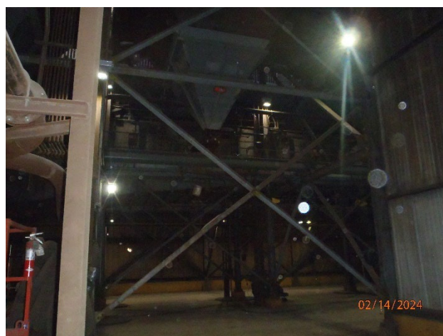
Picture 10 – Furnace Baghouse interior and hoppers
