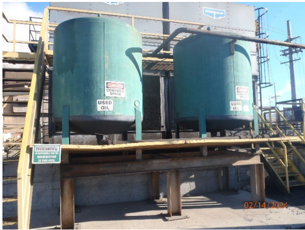
Picture 1 – Roll Mill Used Oil Tanks
