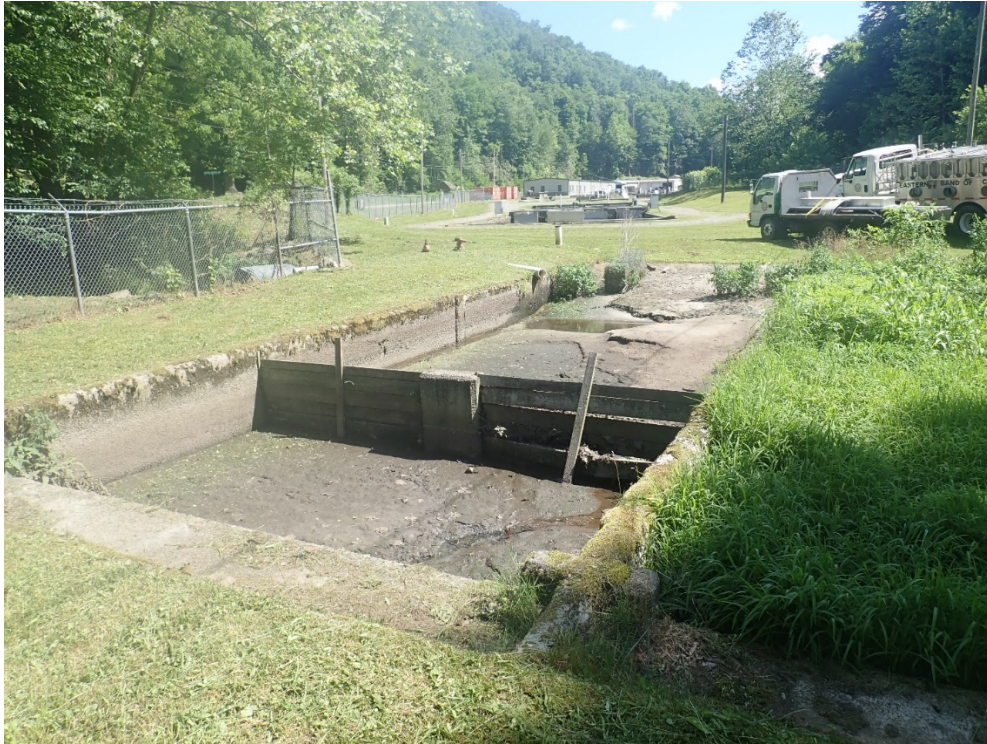
Photo 5. Settling pond with raceways in background. Pond is shown with high sediment buildup. Wooden wall is broken on the right.
