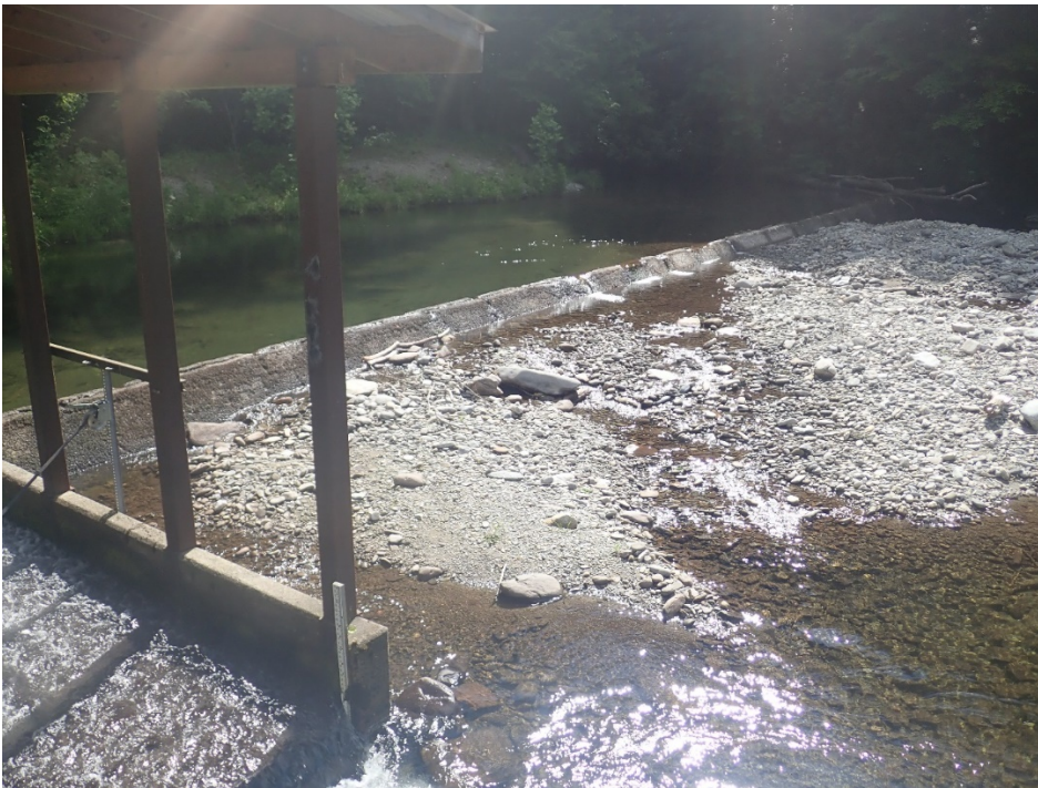
Photo 2. Retaining wall showing wear and damage. Clearer view of sedimentation.
