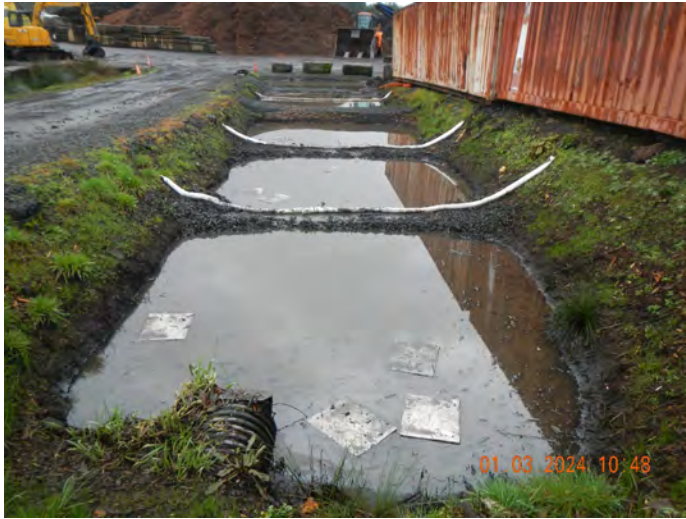
Photo #:11 (DSCN3462) Description: Facing south, photo of the Pond 1 cells/chambers.
