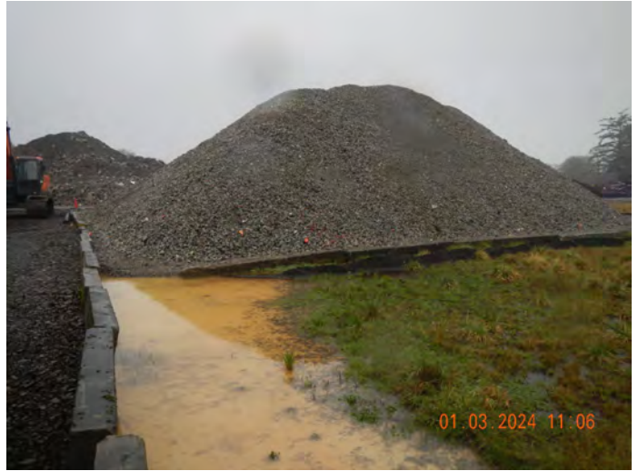
Photo #:26 (DSCN3475) Description: Facing north, ponded stormwater south of inerts storage area.
