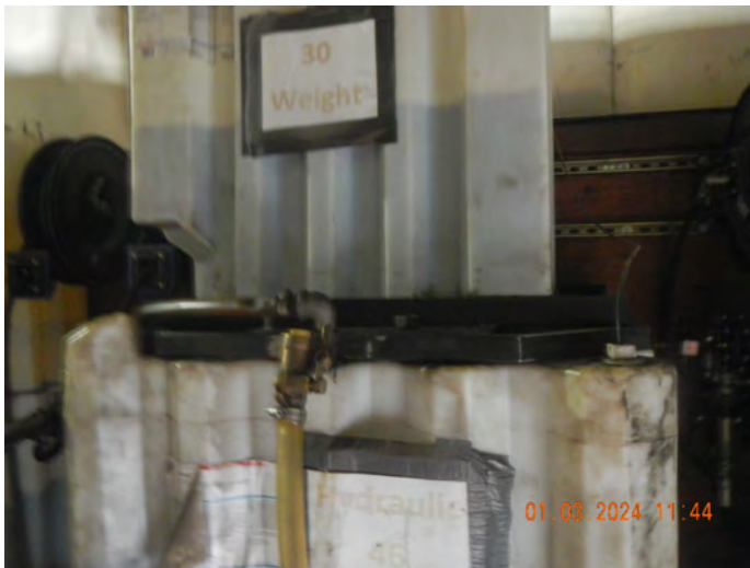
Photo #:55 (DSCN3504) Description: Photo from inside the maintenance shop, hydraulic fluid storage tote.
