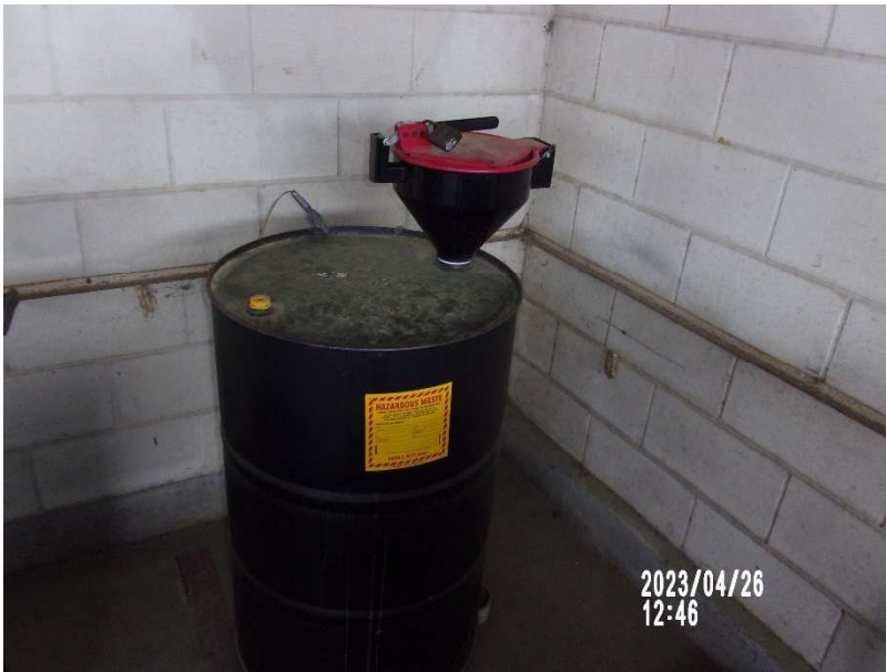
Photograph 29: Building 449, SAA B, Container Missing Hazard Indicator
