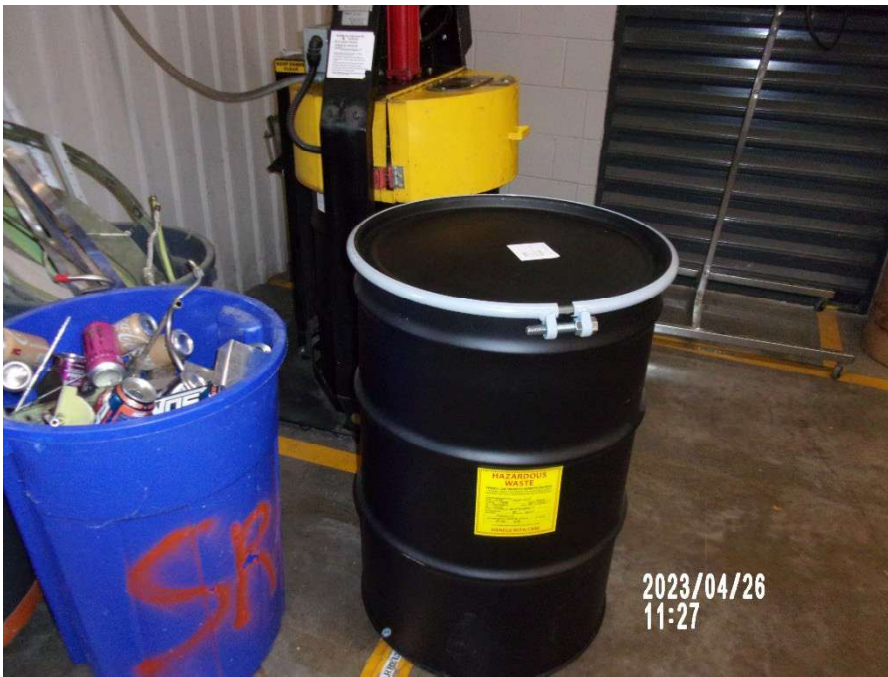
Photograph 5: 55-Gallon Container Missing the Hazard Indicator
