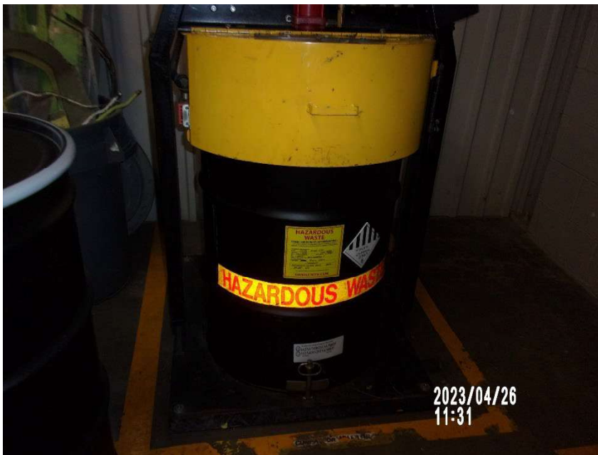
Photograph 7: Hazard indicator information added to container.
