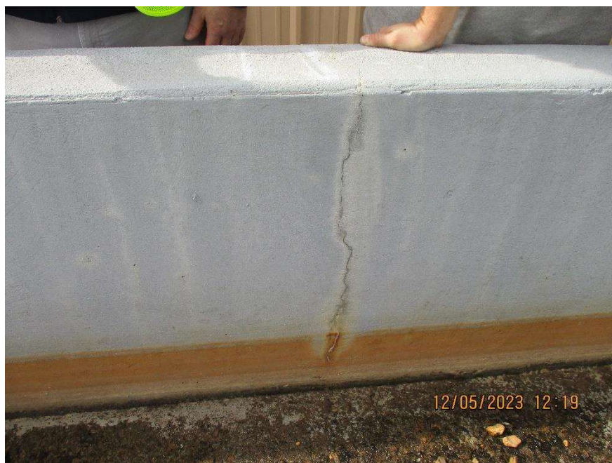
Photo # 8 Cracks inside secondary containment
