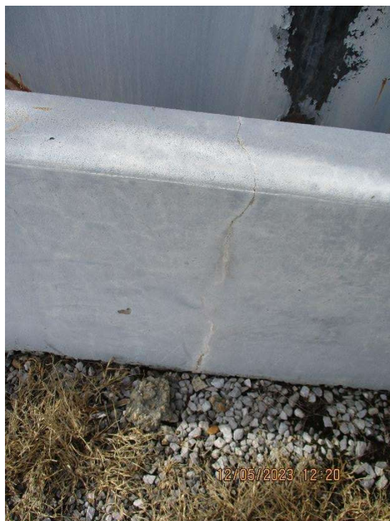
Photo # 9 Cracks outside the secondary containment
