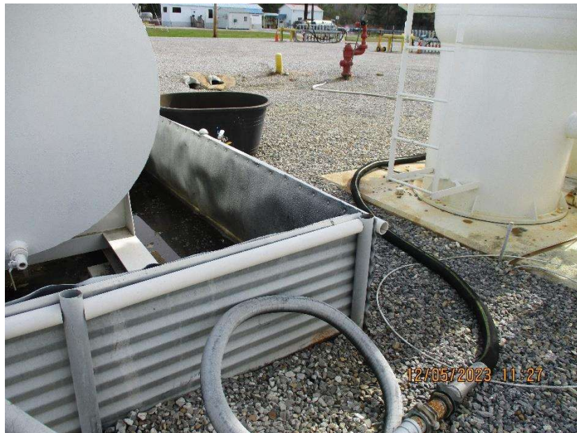
Photo #4 Hose attached to the tank
