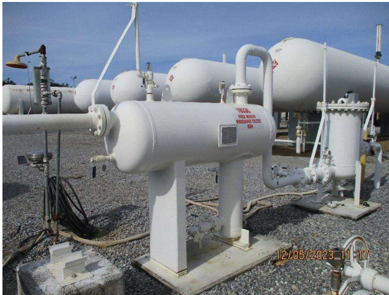
Photo #2 “Knockout Filter Tank”
