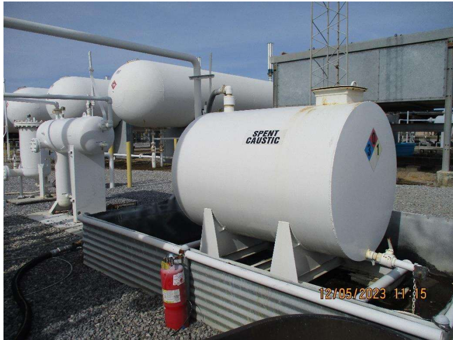
Photo #3 "Spent Caustic Tank"
