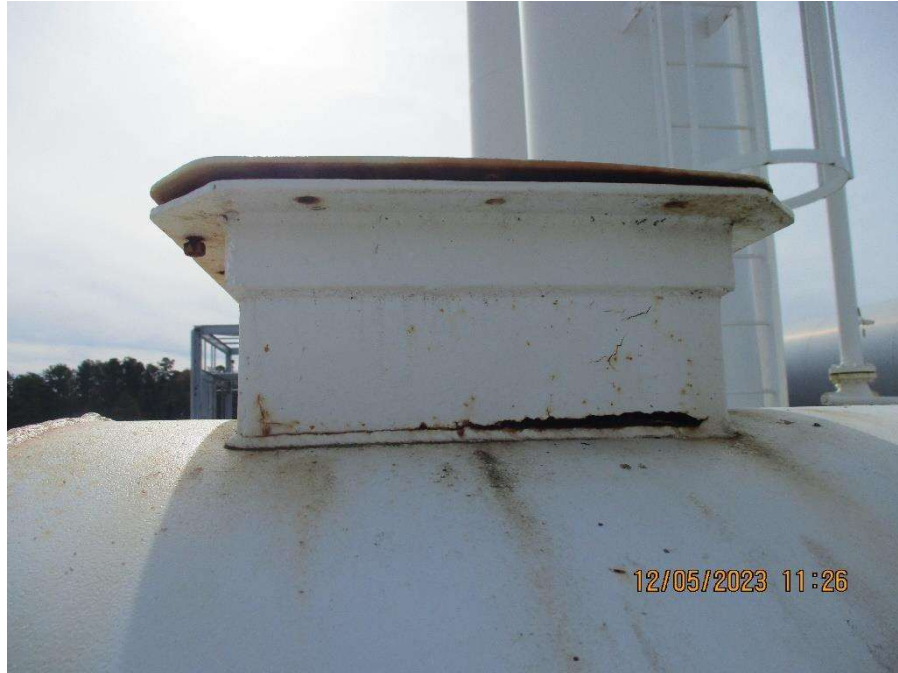
Photo # 5 Containment on top of the "spent caustic tank" with open lid
