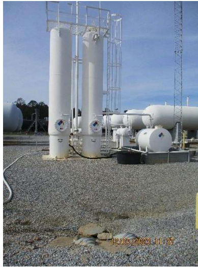
Photo #1 General view of the treater towers, “spent caustic tank” LPG and butane tanks
