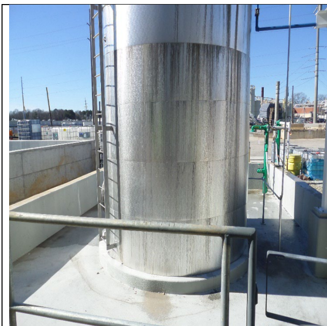
AEI. Tank T-3030. The inspectors observed the tank pumps, valves, and flanges and other pipe connections were not marked to identify each piece of equipment. The inspectors observed the tank was not labeled or marked with the words hazardous waste and not marked with a date. Photograph 9 taken at 12:19 p.m.
