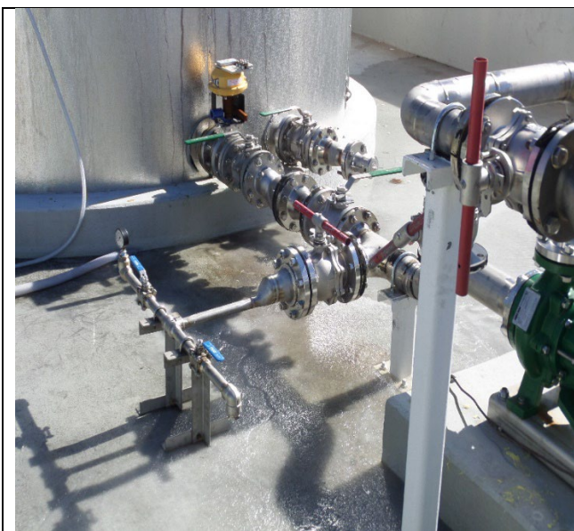
AEI. Tank T-3030. The inspectors observed the tank pumps, valves, and flanges and other pipe connections were not marked to identify each piece of equipment. The inspectors observed the tank was not labeled or marked with the words hazardous waste and not marked with a date. Photograph 11 taken at 12:19 p.m.
