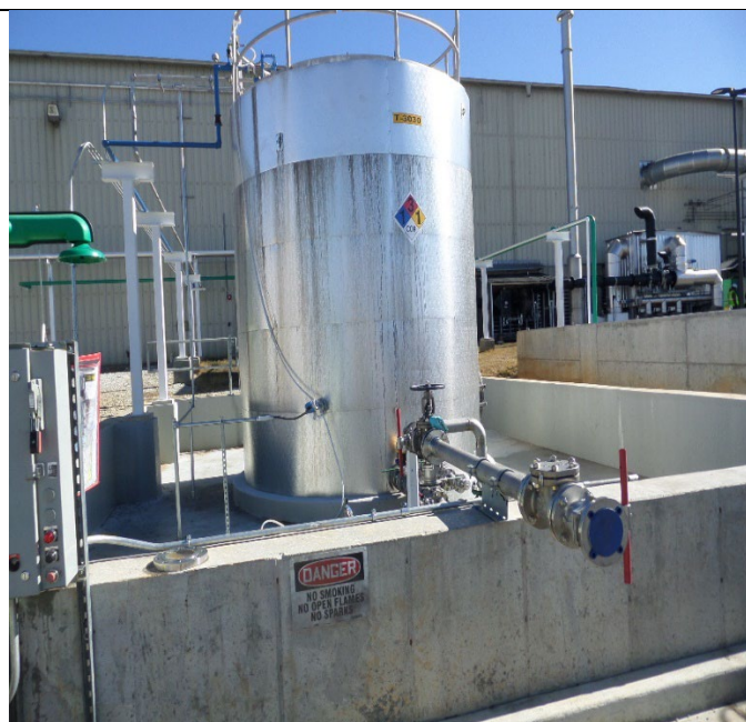
AEI. Tank T-3030. The inspectors observed the tank pumps, valves, and flanges and other pipe connections were not marked to identify each piece of equipment. The inspectors observed the tank was not labeled or marked with the words hazardous waste and not marked with a date. Photograph 10 taken at 12:19 p.m.
