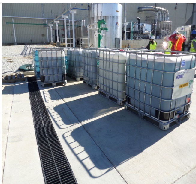
AEI. Tank T-3030. The inspectors observed five 250-gallon totes accumulating scrubber water. Tank T-3030 is in the background. Photograph 8 taken at 12:17 p.m.
