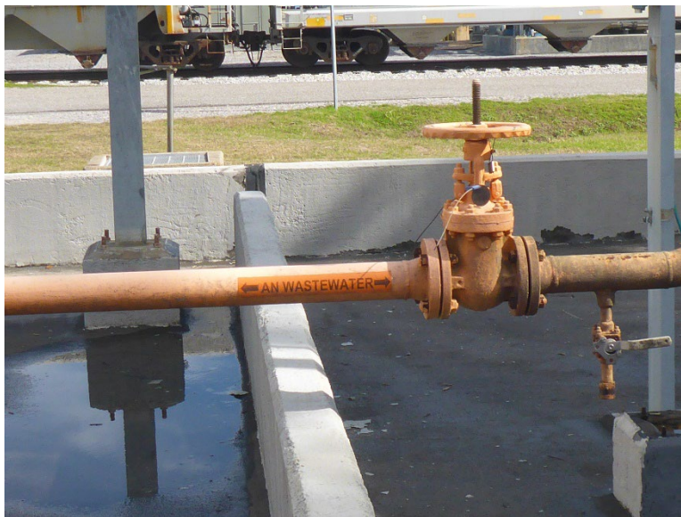
Photo 4: Piping to transfer combined influent line to the hazardous waste storage tanks.
