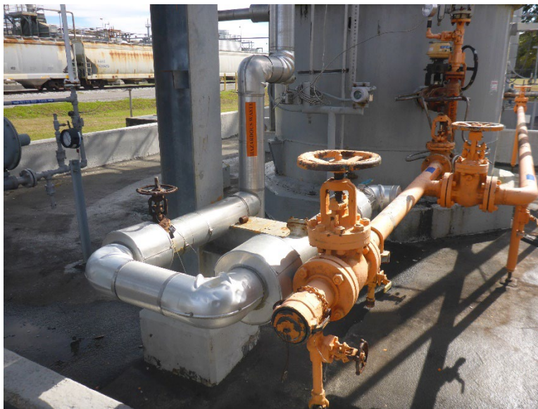
Photo 5: Piping to transfer combined influent line to the hazardous waste storage tanks.
