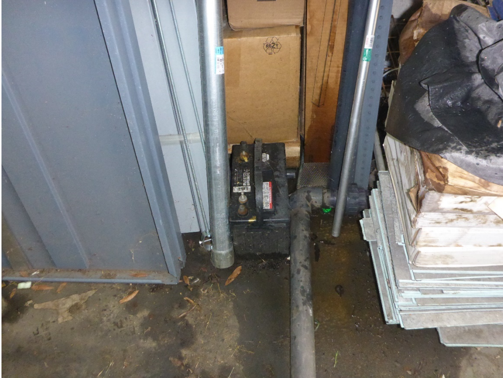
Photo 11: One used battery located on the floor next to the shelving unit in the Contractor Storage Room.
