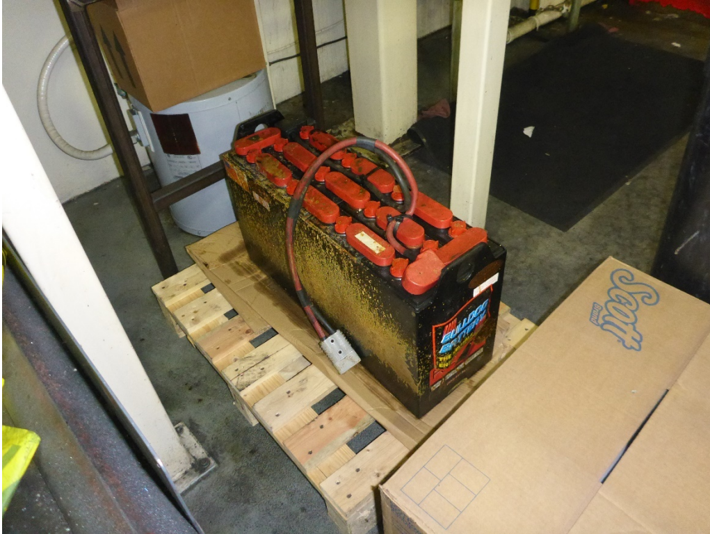
Photo 6: Large battery taken from a tool cart in the Press Department. Staged in the Maintenance Area. The battery appeared to be leaking, and it was not labeled as universal waste.
