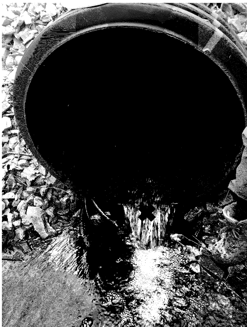
Market01 (photo taken 05/24/22 at 09:05 AM) Outfall located near the eastern side of the parking lot at 1 Essex Dr into an unnamed stream into the Shawsheen River. Sample point is indicated by a red x.
