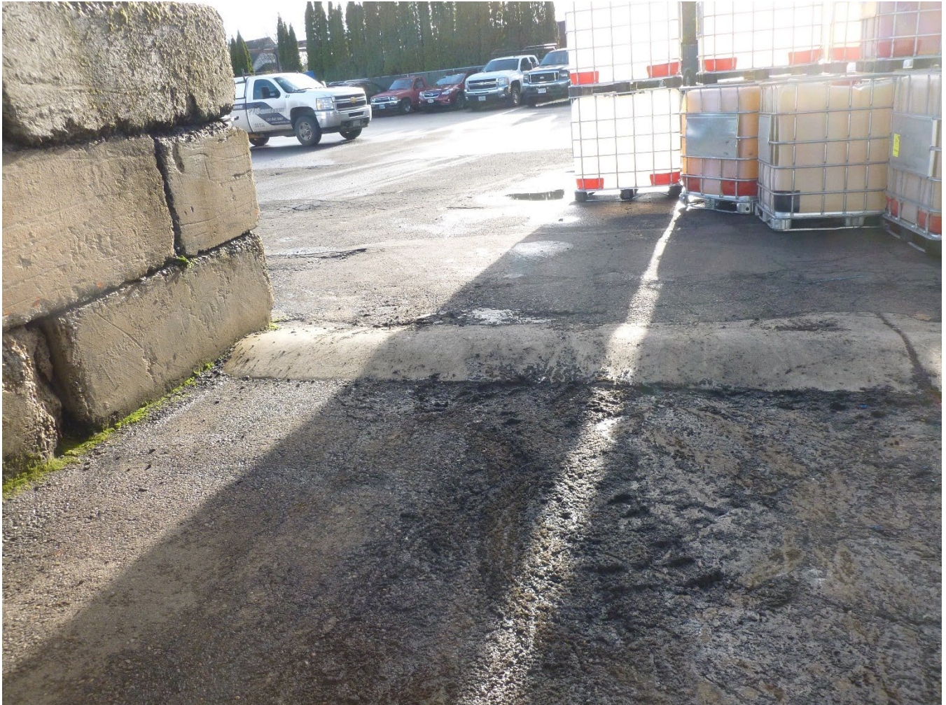
Photo 7 / P1010049 – Spill Containment Berm
