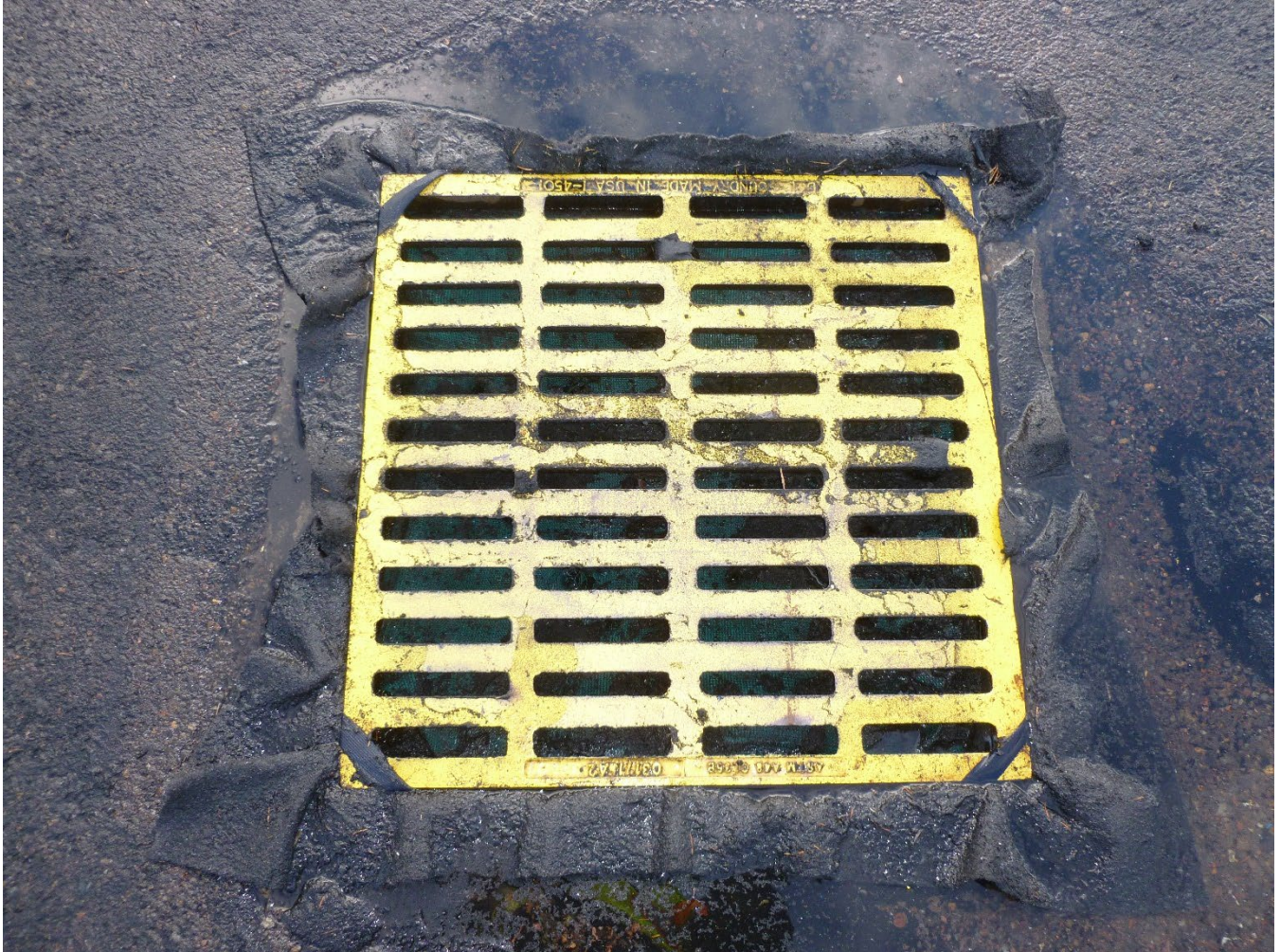
Photo 9 / P1010053 – Catch Basin with Sodium Ion Filter
