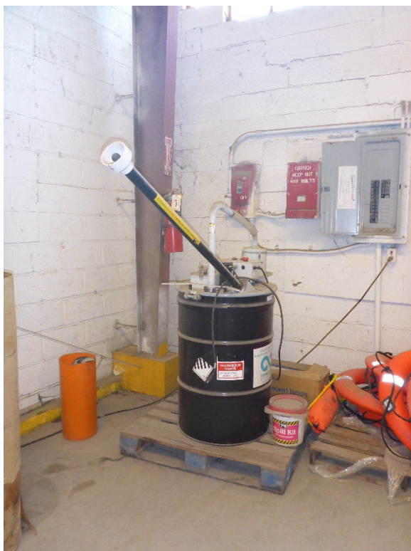
Photo 11: One 55-gallon drum equipped with a bulb-crusher unit in the SAA in the near left corner of the CAA warehouse. The drum was not identified with an indication that its contents are toxic.
