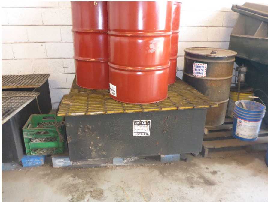
Photo 6: Secondary containment pallet accumulating used oil from 55-gallon drums in the CAA warehouse.
