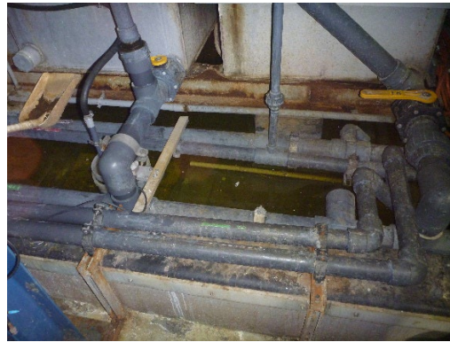
Photo #2 – Several inches of plating rinse water stored in the secondary containment.
