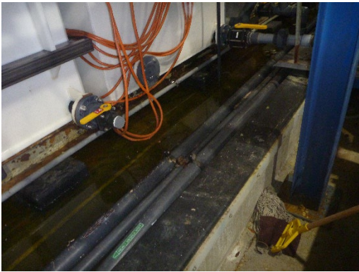
Photo #1 – Several inches of plating rinse water stored in the secondary containment.
