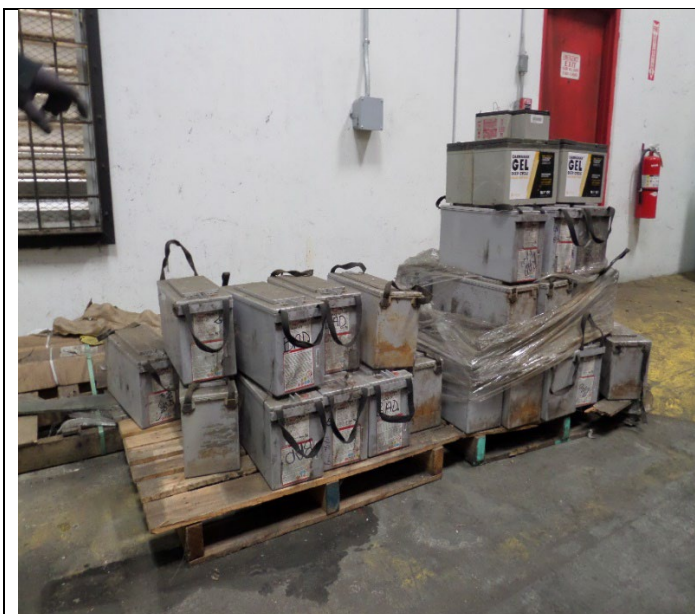
CAA. Observed universal waste batteries not marked or labeled universal waste and not dated. Facility labeled and dated the batteries. Photograph 9 taken at 12:11 p.m.
