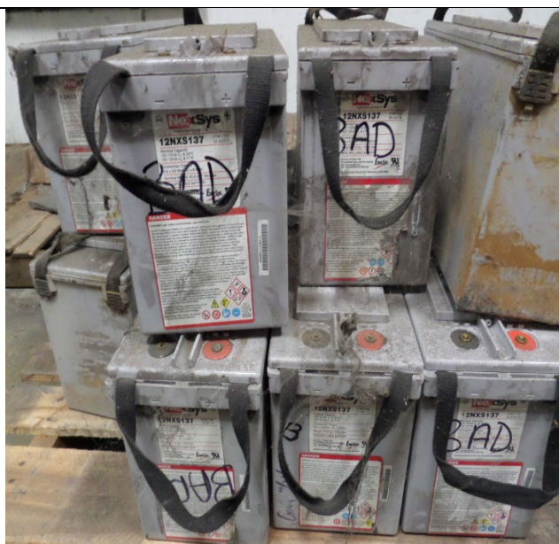
CAA. Observed universal waste batteries not marked or labeled universal waste and not dated. Facility labeled and dated the batteries. Photograph 10 taken at 12:11 p.m.
