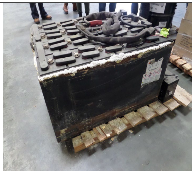
CAA. The inspectors observed one “sitdown equipment” battery leaking and not marked as universal waste and not dated. Facility managed the battery and shipped it off-site for disposal. Photograph 14 taken at 12:21 p.m.
