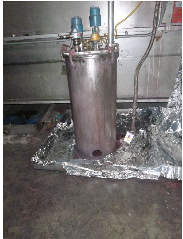
Photograph 73: Recirculation Tank for waste solvent.
