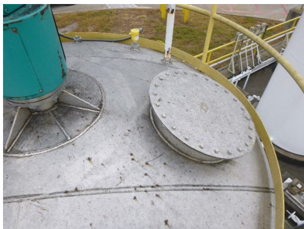
Photograph 33: Hazardous Waste Tank CAA.
