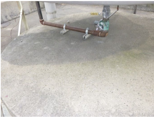
Photograph 36: Hazardous Waste Tank CAA.
