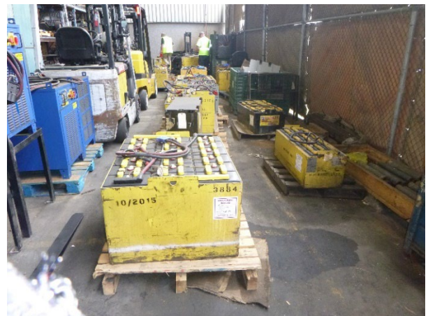
Photograph 50: Universal Waste Battery Storage.
