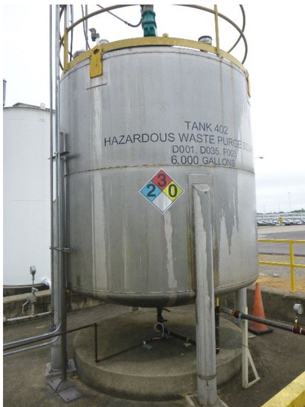
Photograph 32: Hazardous Waste Tank CAA.
