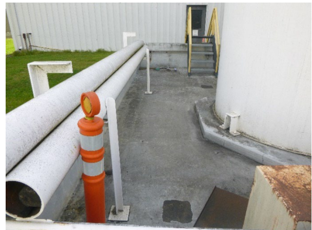
Photograph 59: Used Oil Tank.
