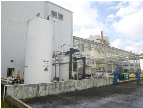
Photograph 56: Used Oil Tanks.
