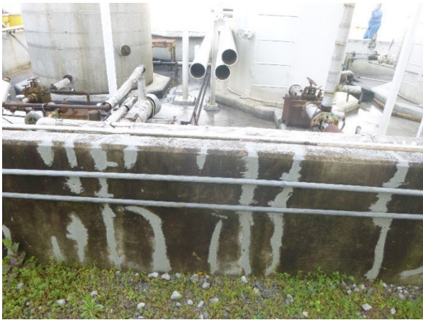
Photograph 60: Used Oil Tank.
