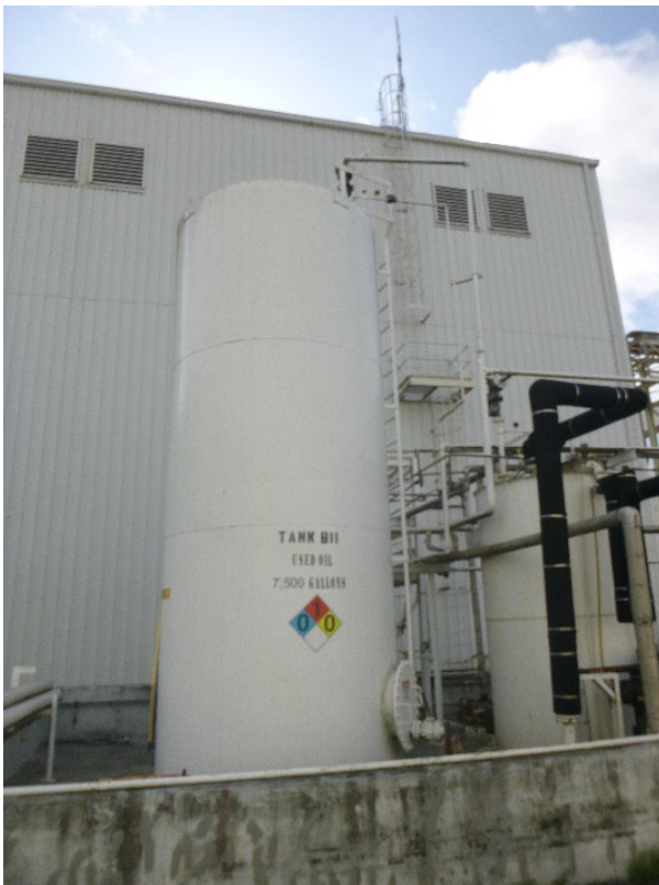
Photograph 57: Used Oil Tank.
