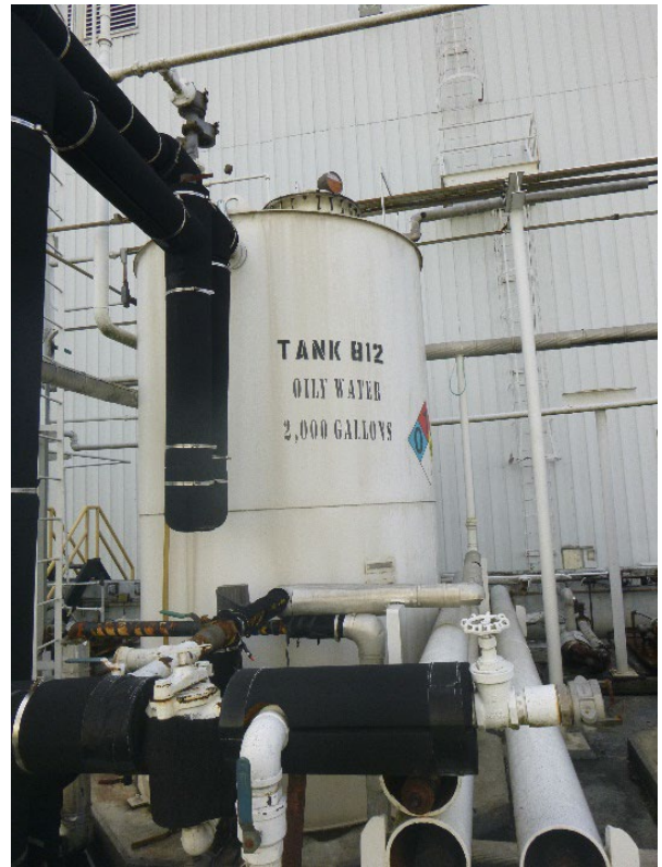
Photograph 58: Used Oil Tank.
