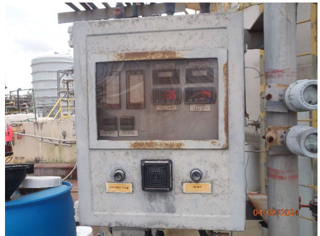
Picture 5 – Hazardous Waste Tank level
