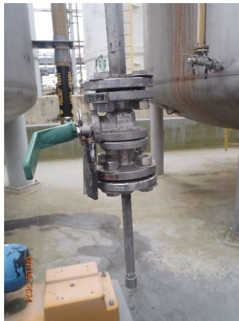
Picture 9 – Hazardous Waste Tank sample port missing BB tags
