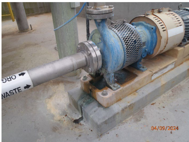
Picture 8 – Hazardous Waste Tank 647 recirc pump leaking
