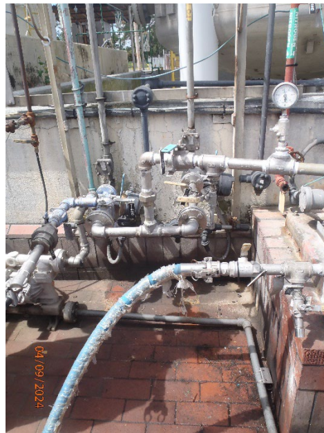
Picture 15 – HW tote unloading pump and piping
