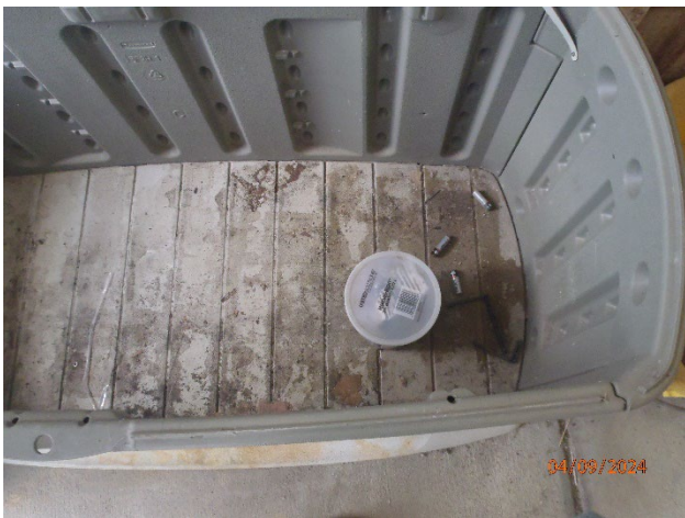
Picture 30 – Universal Waste Batteries - lead acid
