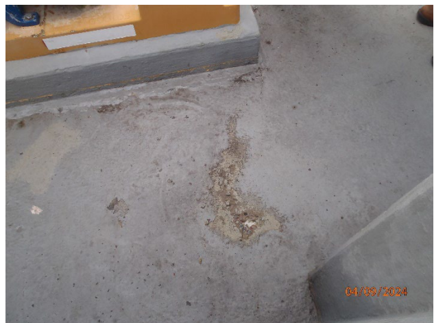
Picture 10 – Hazardous Waste Tank secondary containment corroded
