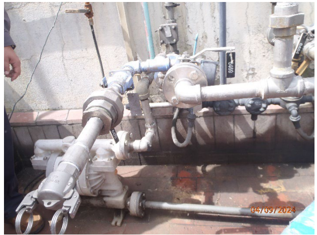
Picture 14 – HW tote unloading pump missing bolt
