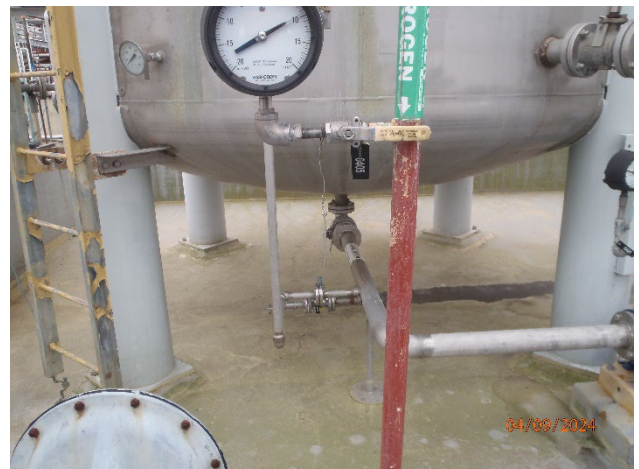
Picture 6 – Hazardous Waste Tank missing BB tags
