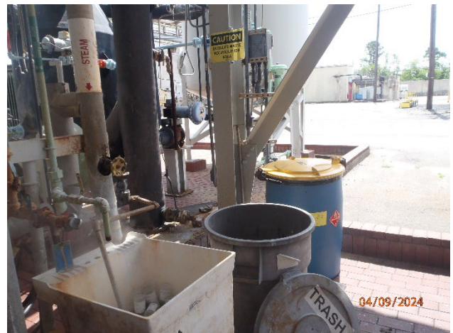
Picture 21 – BRIQUEST Unit SAA
