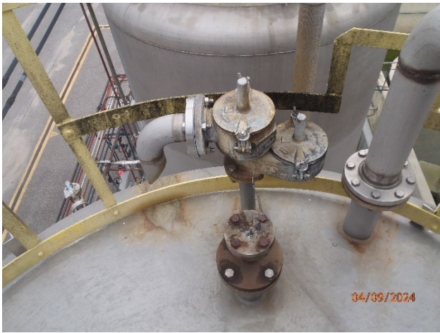
Picture 11 – Hazardous Waste Tank roof missing BB tags
