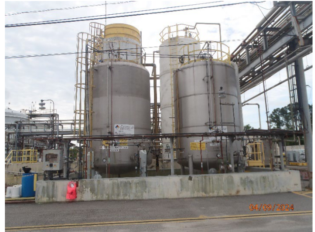
Picture 4 – Hazardous Waste Tanks 646 and 647
