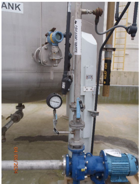
Picture 7 – Hazardous Waste Tank missing BB tags
