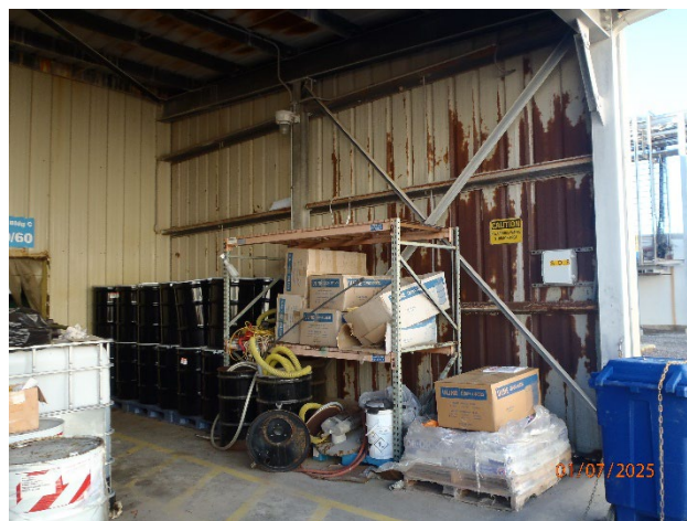
Picture 4 – Hazardous Waste Storage Area (HWSA)
