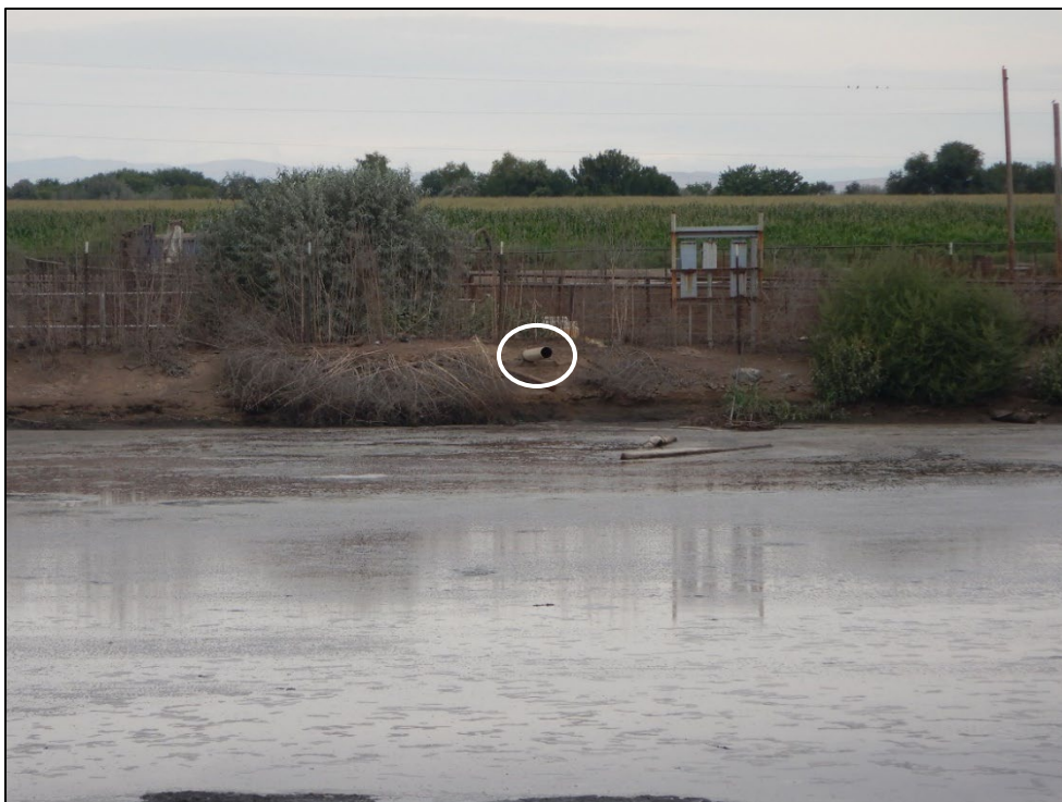
Photograph 18. View looking west towards the pipe (circled) that conveys wastewater from the Settling Pit to Lagoon 2.
