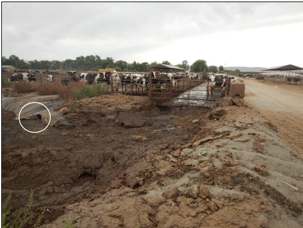
Photograph 22. View looking south along the western edge of the Pen 4 Pit and the Pen 4 feed alley. The inspection team observed a tear in the plastic liner (circled).
