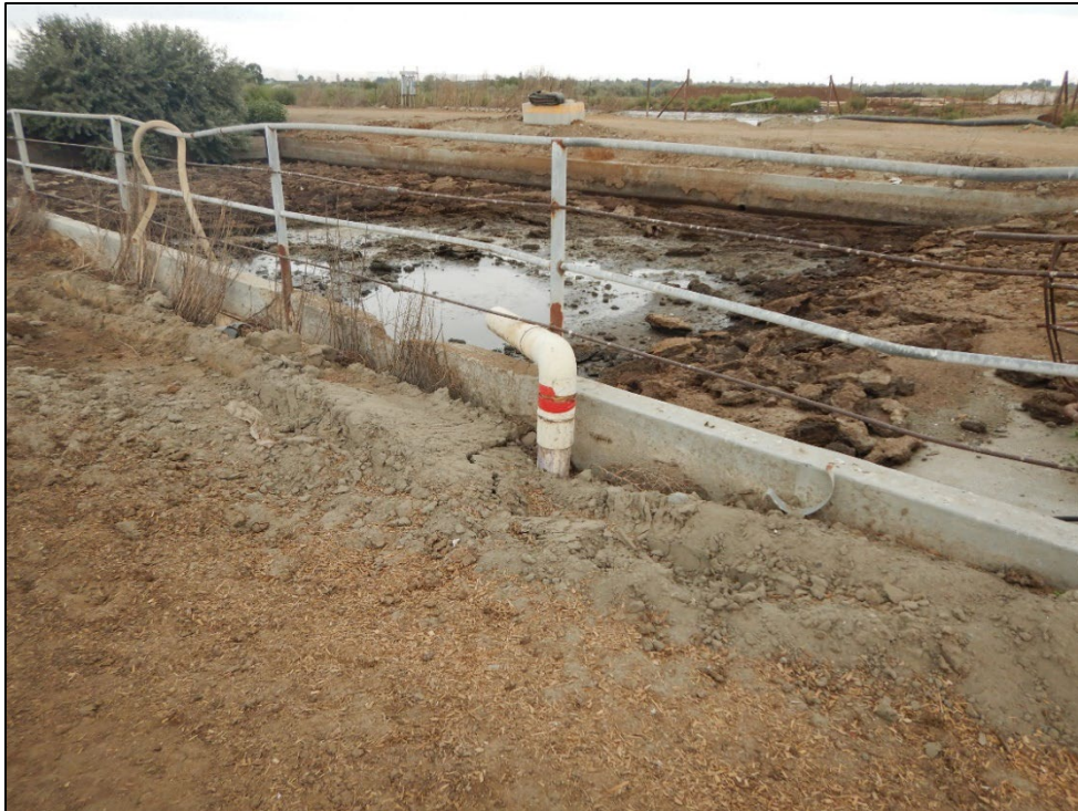
Photograph 27. View looking northeast across the Settling Pit. The PVC pipe shown in the photograph conveys wastewater from the Milk Parlor Pit to the Settling Pit.
