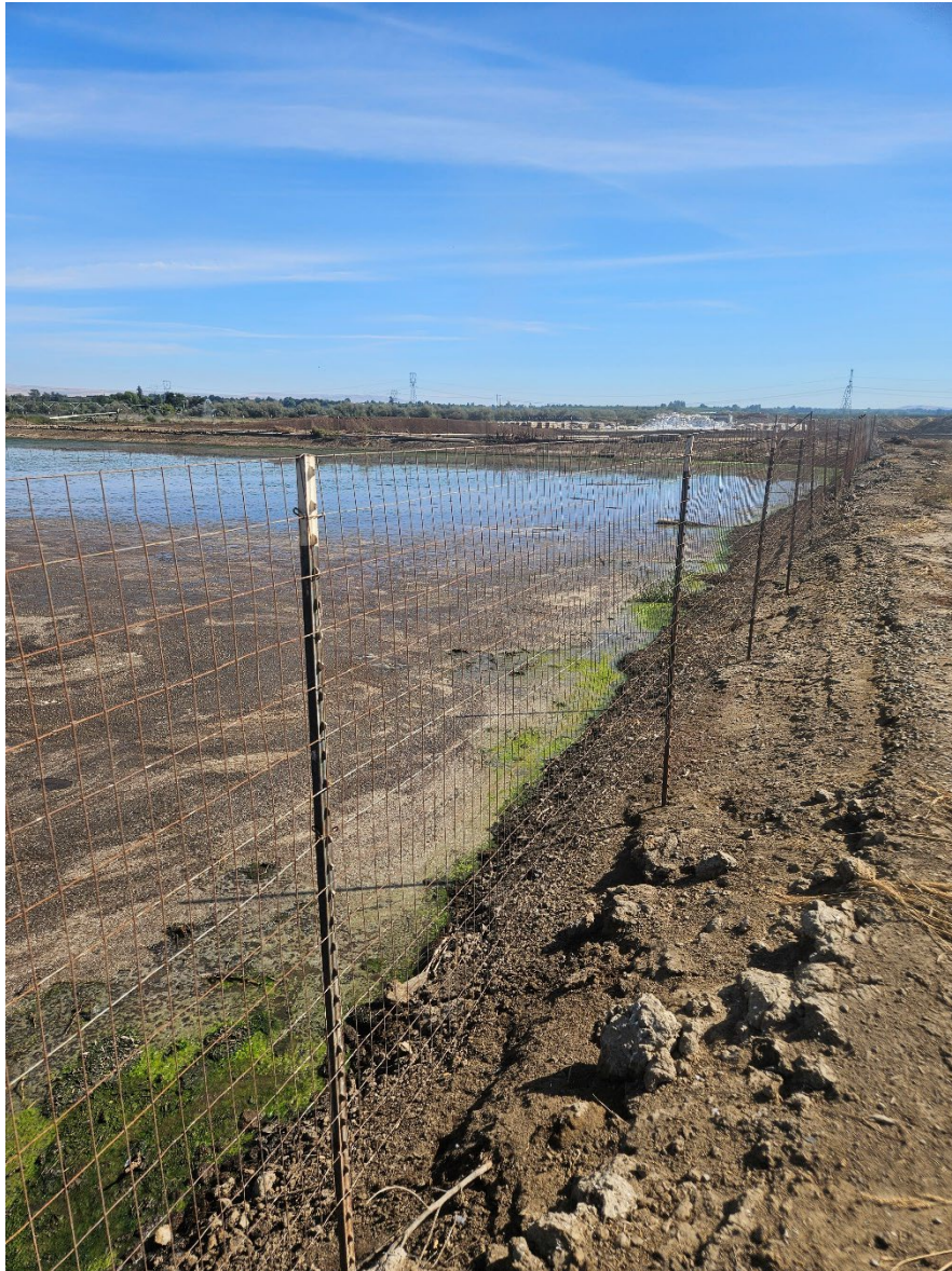
Photograph 2. View of Lagoon 2. Note the absence of vegetation compared to the photographs taken during the inspection site tour.
