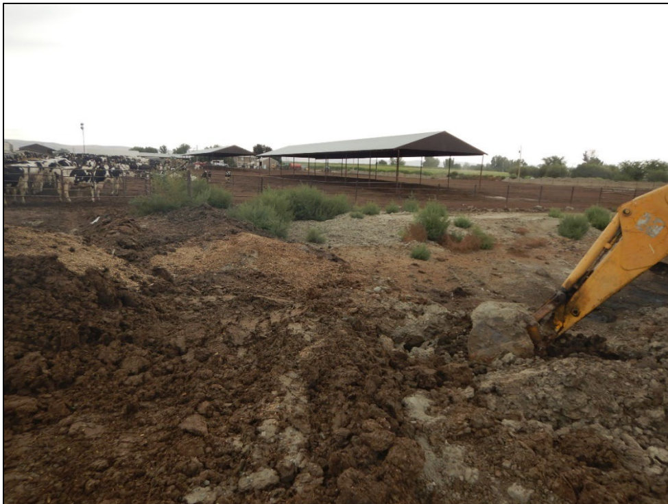
Photograph 29. Additional view looking southwest of the low spot shown in Photograph 27 .
