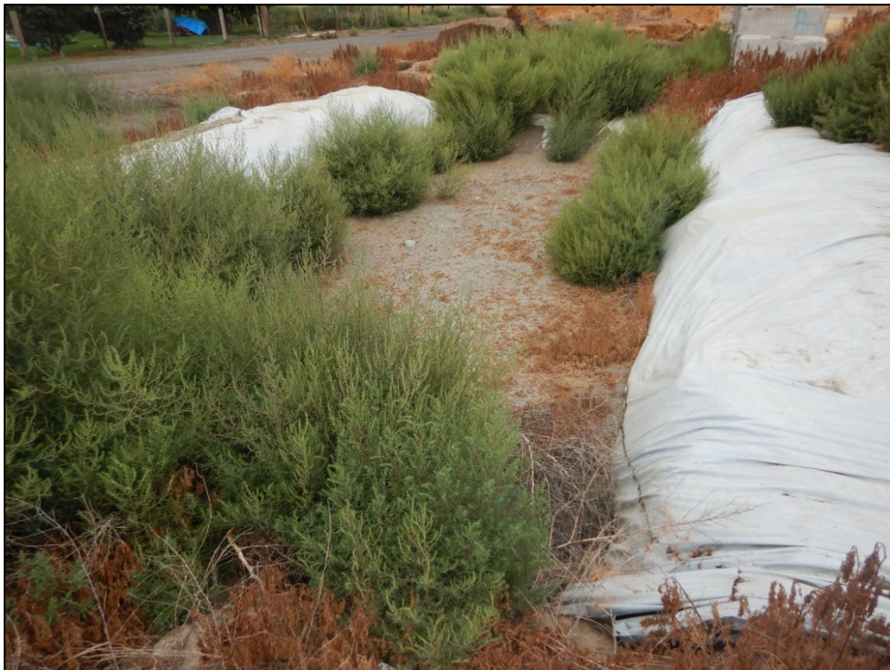
Photograph 8. Additional view looking west across the East Silage Pit shown in Photographs 6 & 7 . Note the heavy vegetation growing within the pit.
