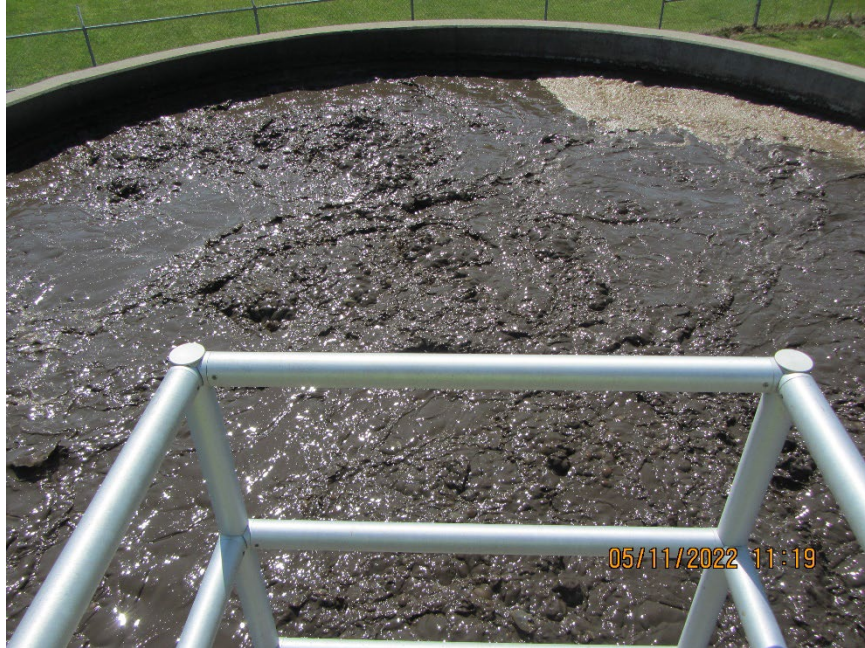
20: IMG_0268 Description: Sludge holding tank Location: East of aeration/digester/clarifier tank Camera Direction: East Date/Time: 5/11/22, 11:19 a.m.
