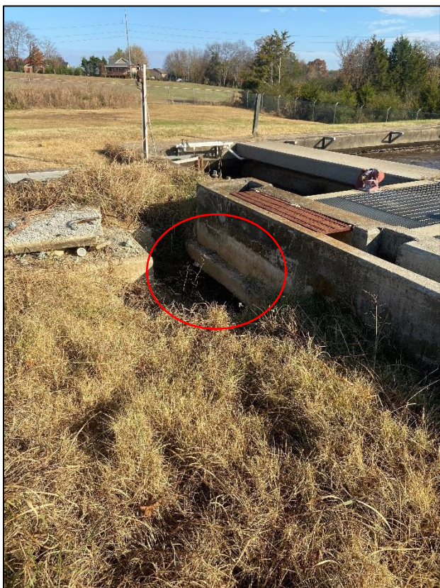
Photo 3: Hole under sludge digester from broken air line to aeration basin.
