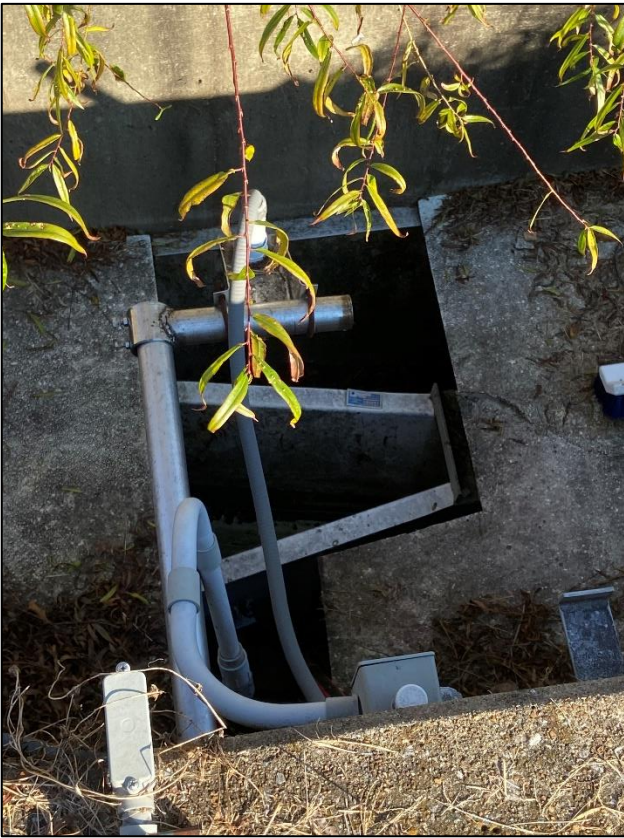
Photo 9: Effluent flow meter (read 0.035 MGD).
