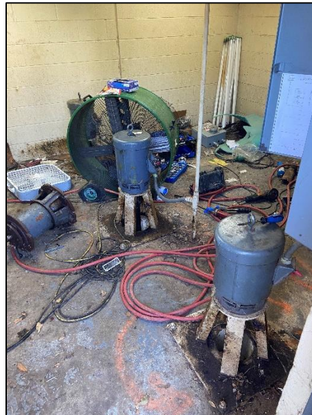
Photo 12. Final pump station upstream of STP (3 pumps).
