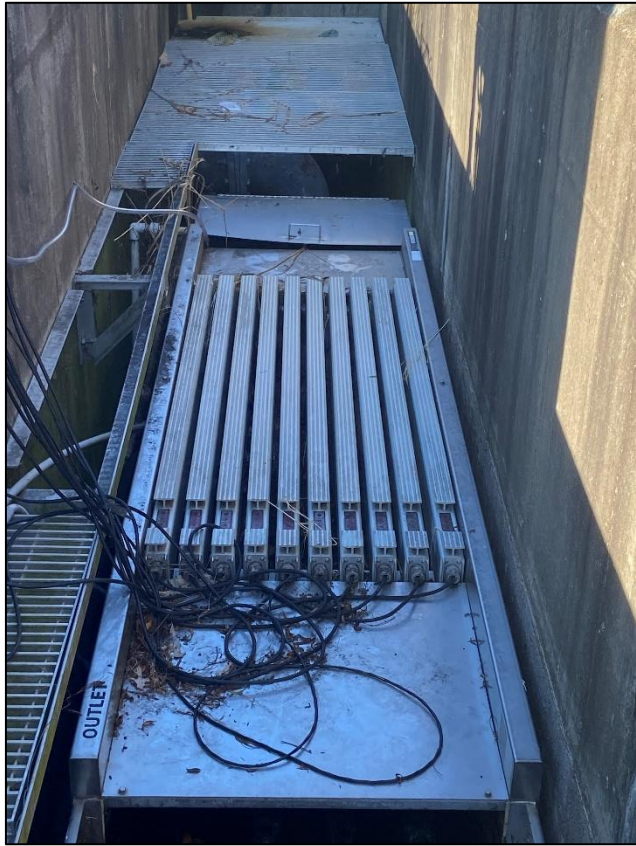
Photo 10: UV disinfection system.
