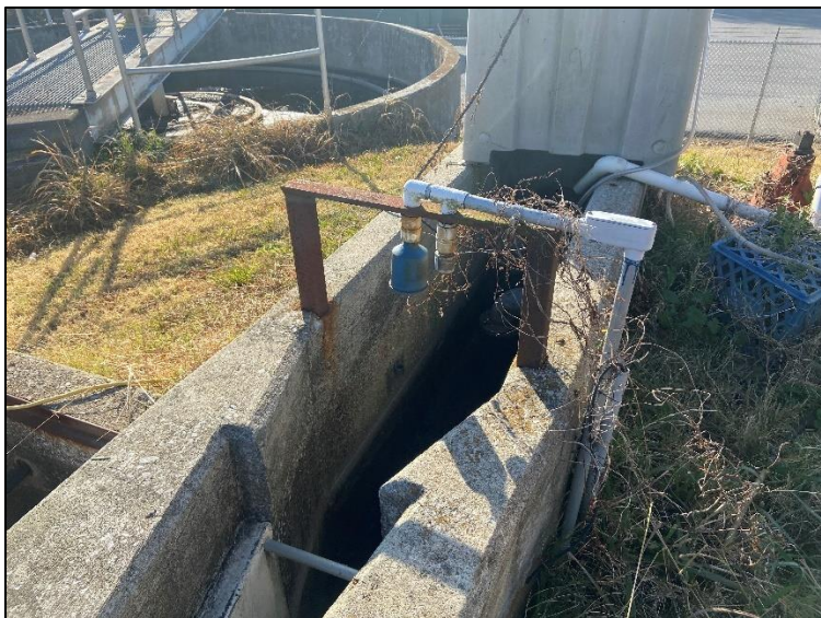
Photo 1: Influent flow meter/weir.
