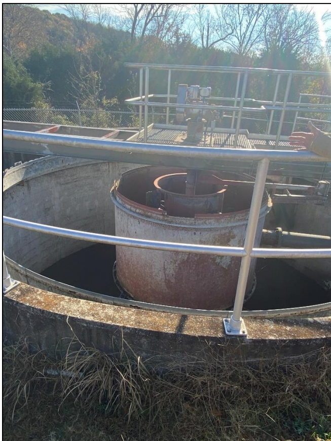
Photo 5: Secondary clarifier #2 (out of service).
