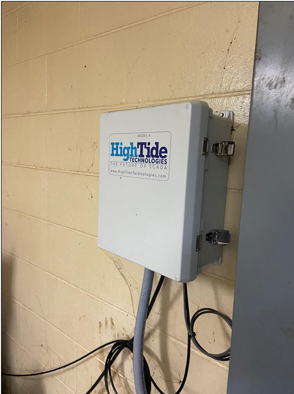
Photo 13. Pump Station SCADA system to cell phone (monitor only; no controls).
