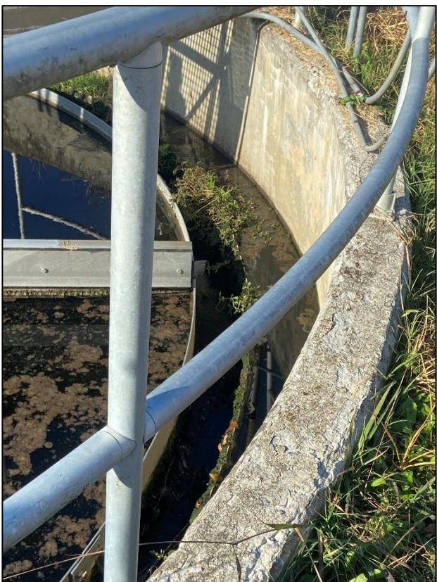
Photo 7: Clarifier #1 (grass growing on weir).
