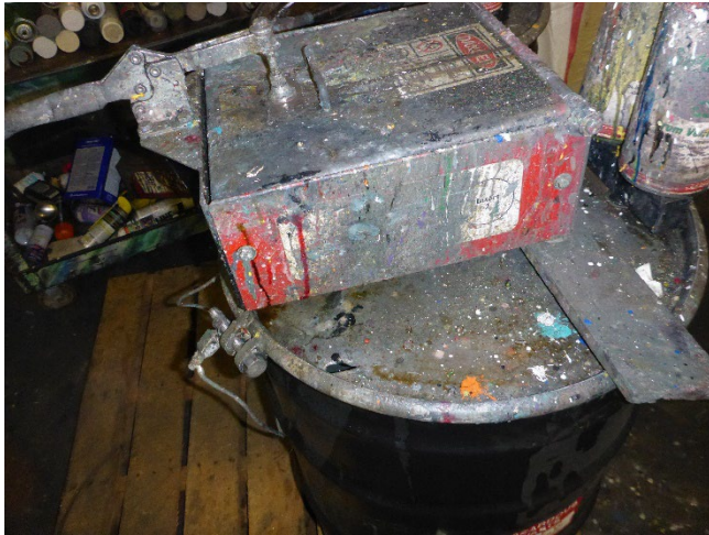
Photo 7 (P1010541.JPG): Hole in the top of a container used to accumulate liquids generated from aerosol can puncturing device in the Aerosol Processing Area.
