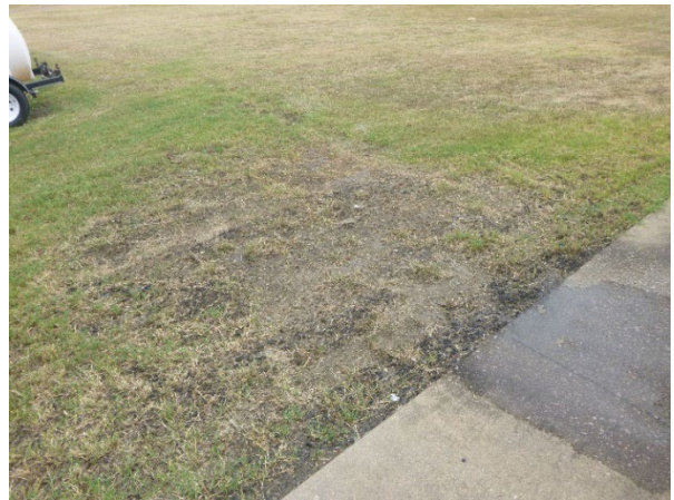
Photograph 57: Stressed vegetation area from roof drain downspout.
