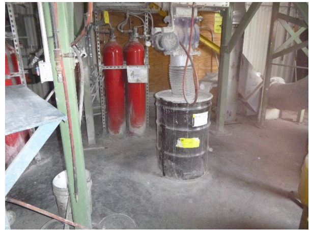
Photograph 33: Leadworks Baghouse SAA.
