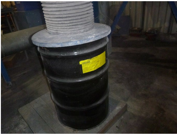
Photograph 36: Leadworks Baghouse SAA.
