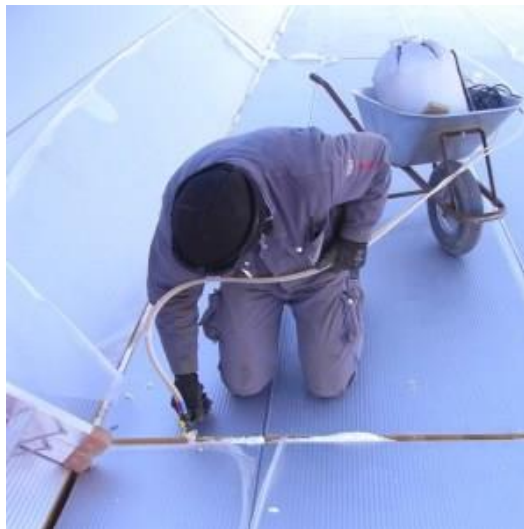
Picture 10: LP SPF cold storage application
