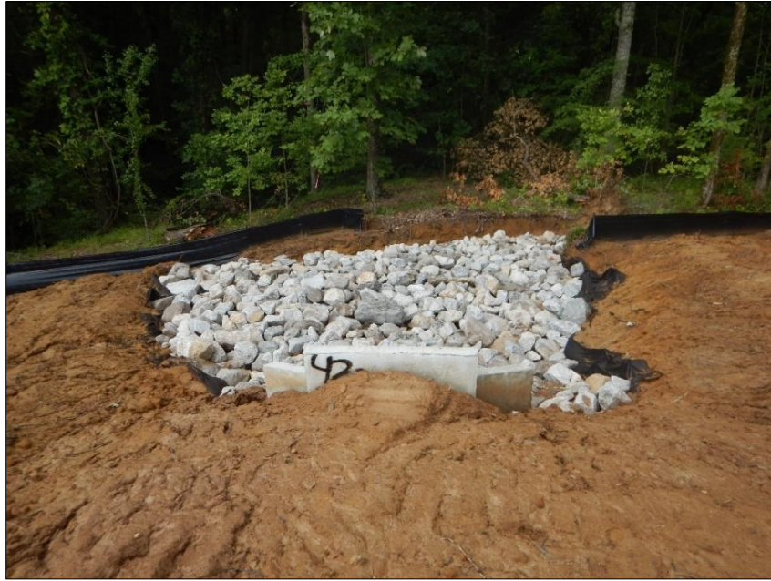
Photograph 23. View, facing west, of constructed Outfall #7 in the western portion of the Site. Slopes around the outfall were unstabilized and eroded.
