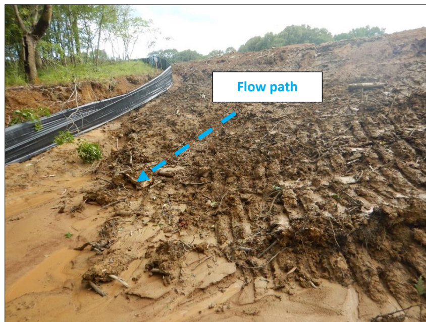
Photograph 26. Upgradient view of an unstabilized slope that leads to the unidentified discharge point shown in Photograph 25 . Silt fence was installed along the slope, not along the contour, at this location and no other slope stabilization measures were installed or implemented. The operator had performed earthwork outside the perimeter silt fence.
