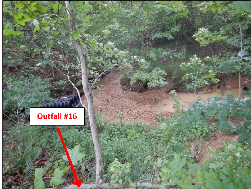
Photograph 41. View of an unnamed tributary to Oliver Creek. The water in the unnamed tributary to Oliver Creek downstream of the Site's Outfall #16 was turbid. The corrugated piping was not installed.
