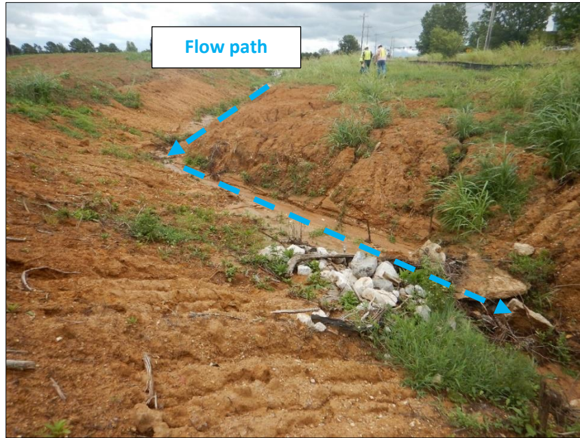
Photograph 57. View, facing northeast of the gully erosion in the center of the Site. The slopes on either side of the gully were unstabilized and eroded.
