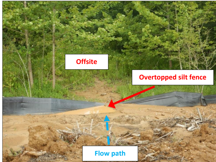
Photograph 67. View, facing west, of sediment overtopping the silt fence and discharging offsite in the center of the Site. The silt fence was installed across the discharge point, an area of concentrated flow.
