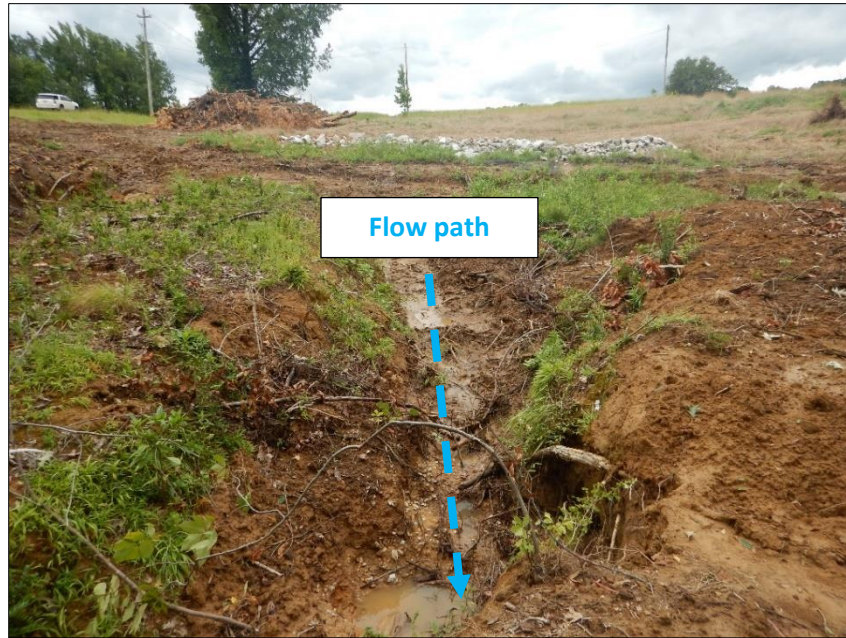
Photograph 53. Upgradient view of gully erosion on an unstabilized slope in the center of the Site. This flow path leads towards an unidentified discharge point shown in Photograph 55 .
