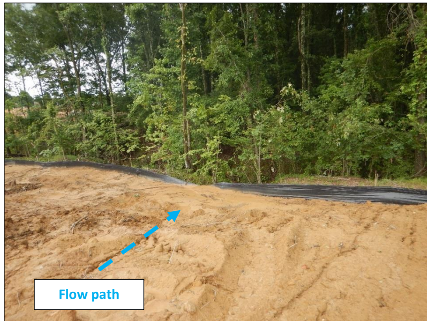
Photograph 28. Downgradient view of an unstabilized and eroded slope in the western portion of the Site. Sediment had overtopped the silt fence and discharged offsite.
