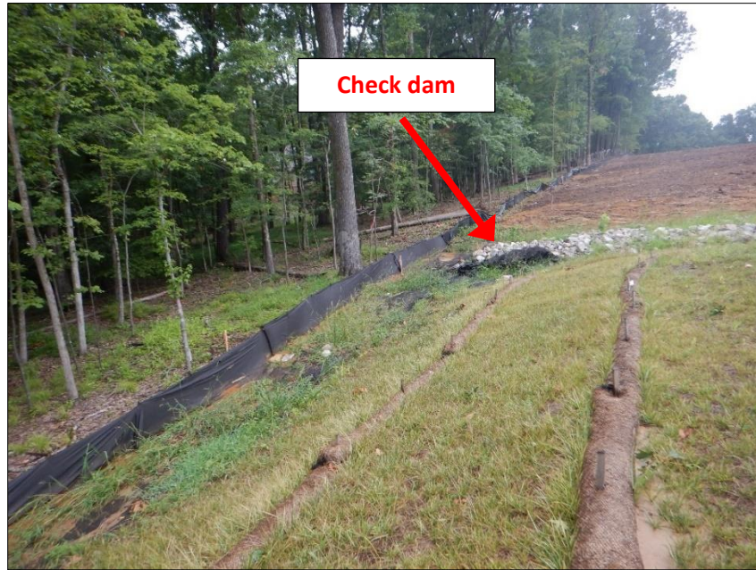
Photograph 29. Upgradient view, facing northeast, of a check dam and straw wattle erosion and sediment controls upgradient of Outfall #18.
