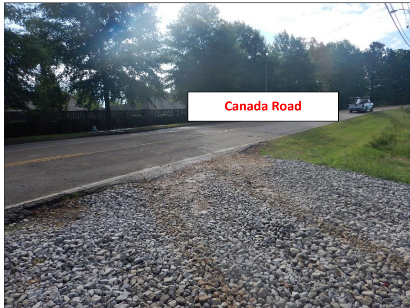
Photograph 2. View, facing southeast, of the stabilized construction entrance/exit off Canada Road. Minor sediment track out was observed. Bare spots were present between the stabilized entrance and Canada Road.
