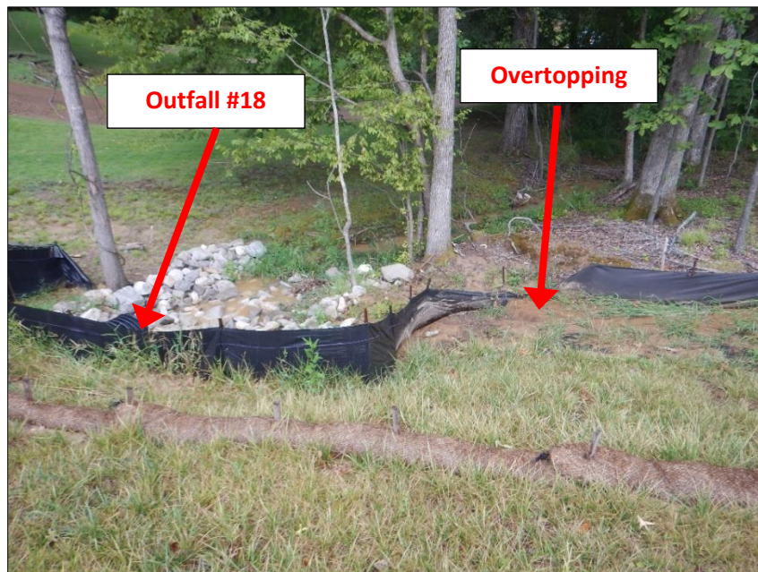
Photograph 30. Downgradient view of Outfall #18 in the southwestern portion of the Site. Vegetative stabilization was not sufficient to prevent sediment from overtopping the silt fence adjacent to the outfall. Sediment was visible downgradient from Outfall #18.
