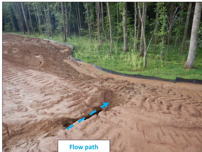
Photograph 20. Downgradient view, facing west, of rill erosion on an unstabilized slope in the northwestern portion of the Site. Sediment had accumulated to more than half the height of the silt fence, on the up gradient side.
