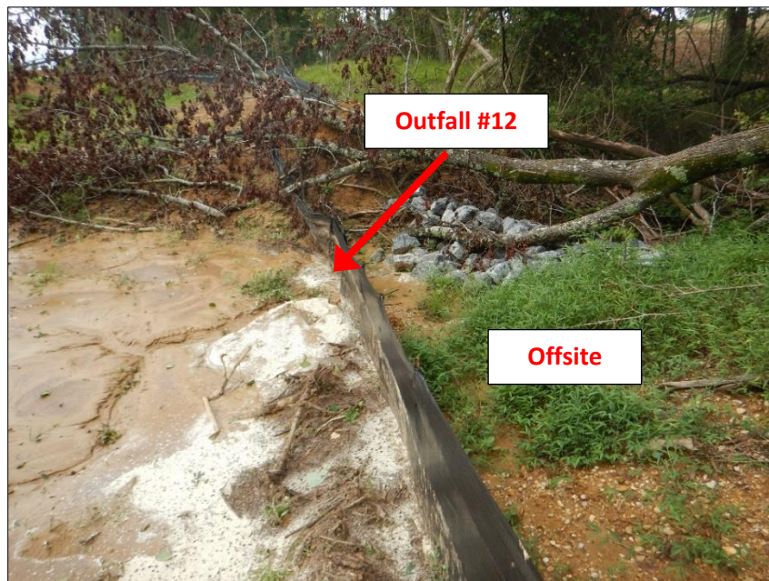
Photograph 66. View, facing southeast, of Outfall #12 in the center of the Site. It was unclear what the white substance on the ground was. The silt fence was installed across the outfall, an area of concentrated flow.
