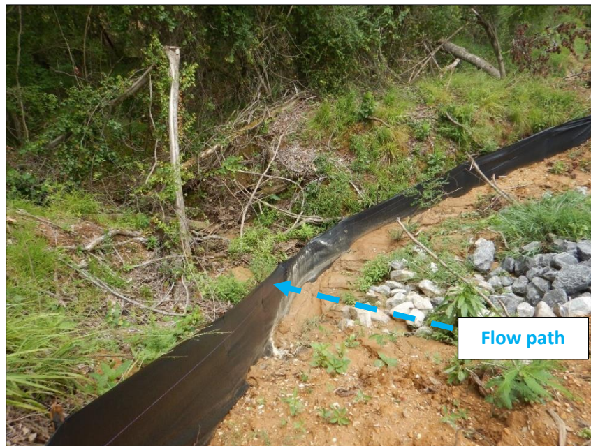
Photograph 64. Closer view of the unidentified discharge point shown in Photograph 63 . The silt fence was installed across the discharge point, an area of concentrated flow.
