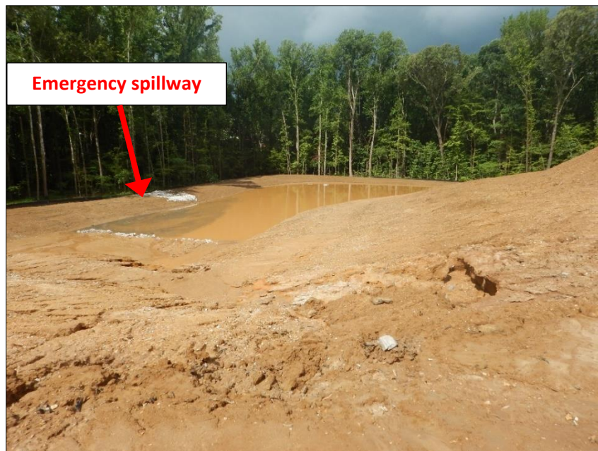
Photograph 6. Downgradient view, facing west, of a permanent sediment basin located in the northwestern portion of the Site. Rill erosion was visible on the unstabilized slopes leading to the basin.
