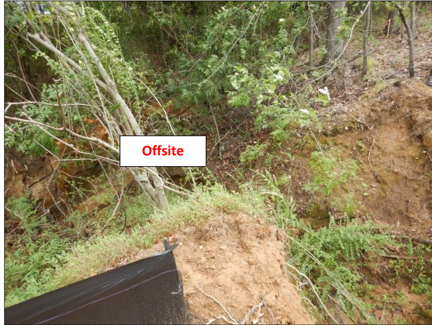
Photograph 55. View, facing northeast, of an unidentified discharge point and head cut in the center of the Site. There was a gap in the silt fence perimeter control in this location.
