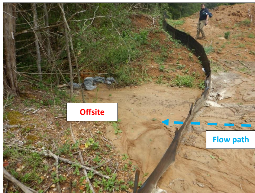
Photograph 62. Additional view of Outfall #14 shown in Photograph 61 . Sediment had discharged offsite. The silt fence was installed across the outfall, an area of concentrated flow.
