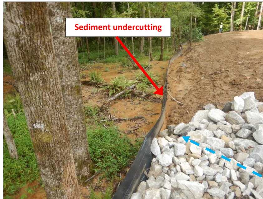
Photograph 13. View, facing north, of a location where the silt fence adjacent to the emergency spillway was incorrectly installed. Upgradient slopes were eroded and not stabilized. The base of the silt fence was not buried, therefore allowing sediment discharges to flow offsite. This area is approximately 75 feet east of an identified wetland area.
