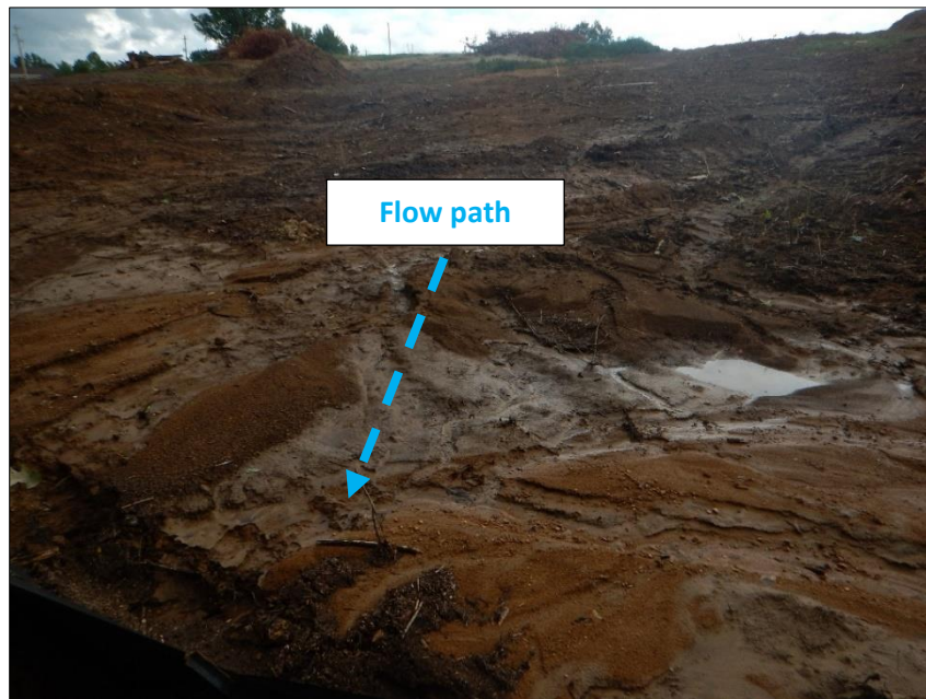
Photograph 42. Upgradient view of an unstabilized and eroded slope in the center of the Site.
