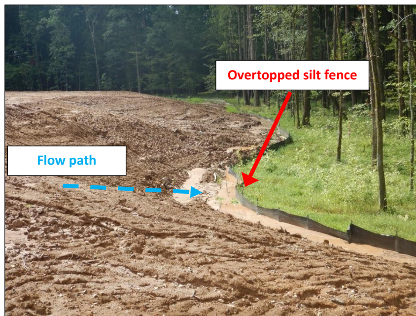
Photograph 8. View, facing south, of an unstabilized slope with rill erosion in the northern portion of the Site. The silt fence at the base of the slope had been overtopped by sediment and stormwater.
