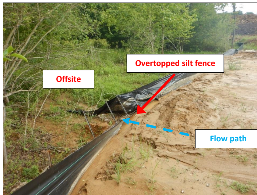
Photograph 68. Additional view of the sediment overtopping the silt fence and discharging offsite in the center of the Site shown in Photograph 67 . The silt fence was installed across the discharge point, an area of concentrated flow.
