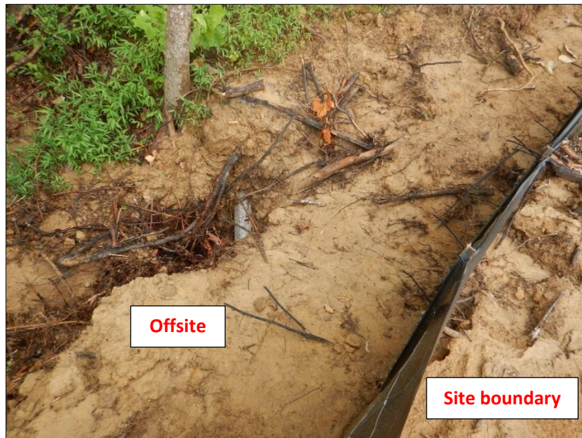
Photograph 40. View of offsite sediment discharge downgradient from Outfall #16. The base of the silt fence was not buried, therefore allowing sediment discharges to flow offsite
