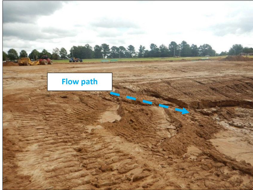
Photograph 21. Upgradient view, facing east, of unstabilized slopes shown in Photograph 20 with rill and gully erosion in the northwestern portion of the Site. Surface roughening was applied in the wrong direction and would increase flow velocity and channelization, not decrease velocity.
