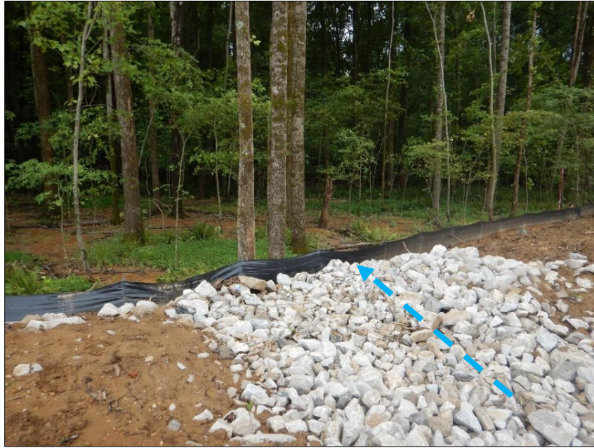
Photograph 11. View, facing west, of the emergency spillway from the sediment basin. Silt fence was installed across the emergency spillway, an area of concentrated flow.
