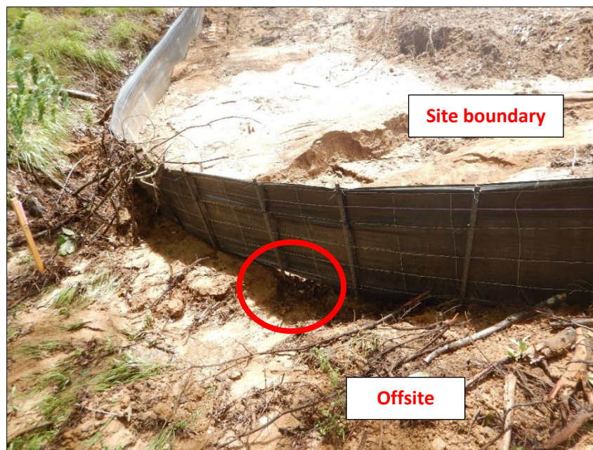
Photograph 48. View, facing east, of the discharge point shown in Photograph 47. The silt fence was not properly buried allowing sediment to undercut the silt fence and discharge offsite (circled in red). The silt fence was installed across the discharge point, an area of concentrated flow.
