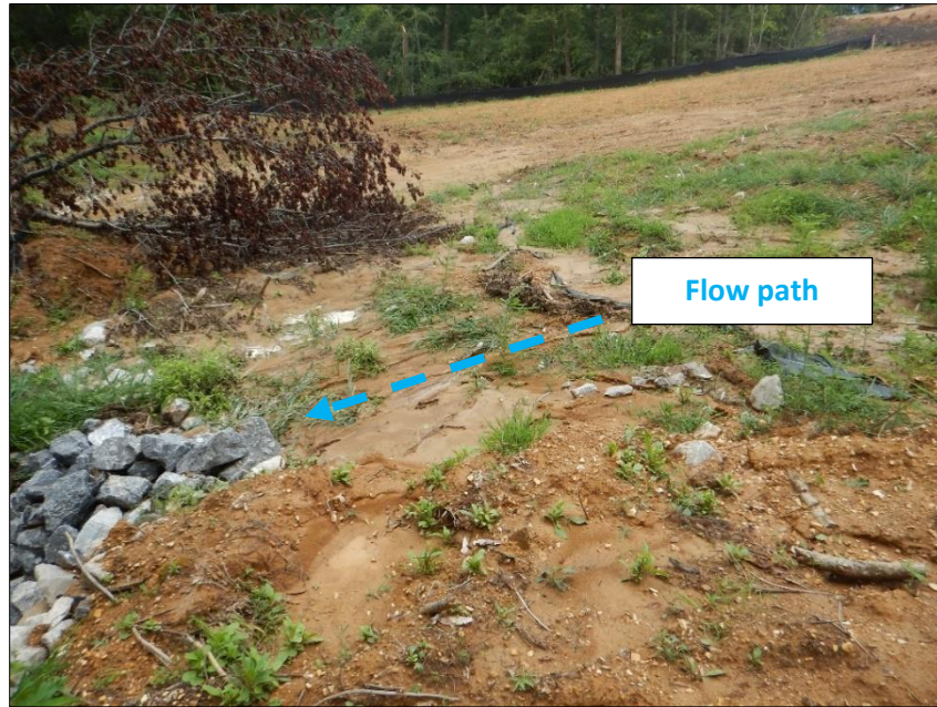
Photograph 63. View, facing northwest, of a stormwater and sediment flow path leading towards an unidentified discharge point in the center of the Site. The slope upgradient from the discharge point was unstabilized.
