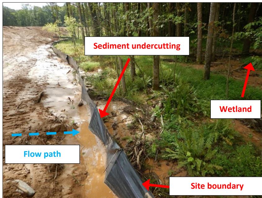
Photograph 12. View, facing south, of turbid water discharged from the Site at the base of a slope in the northwest portion of the Site. The base of the silt fence was not buried, therefore allowing sediment discharges to flow underneath the silt fence and offsite. An identified wetland is located approximately 75 feet west of the silt fence.
