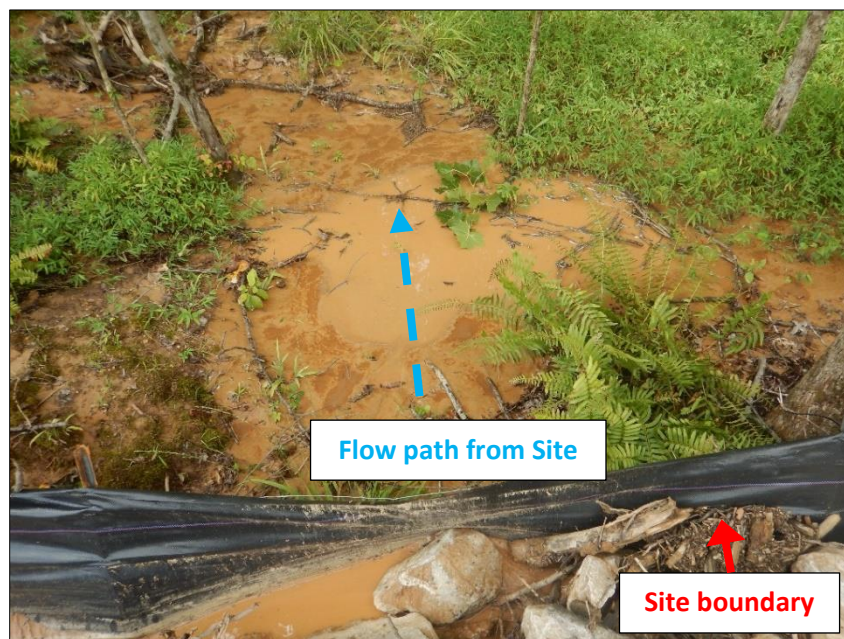
Photograph 14. Closer view of a location where concentrated stormwater flow conveyed sediment under the silt fence (refer also to Photograph 13 ) and offsite.
