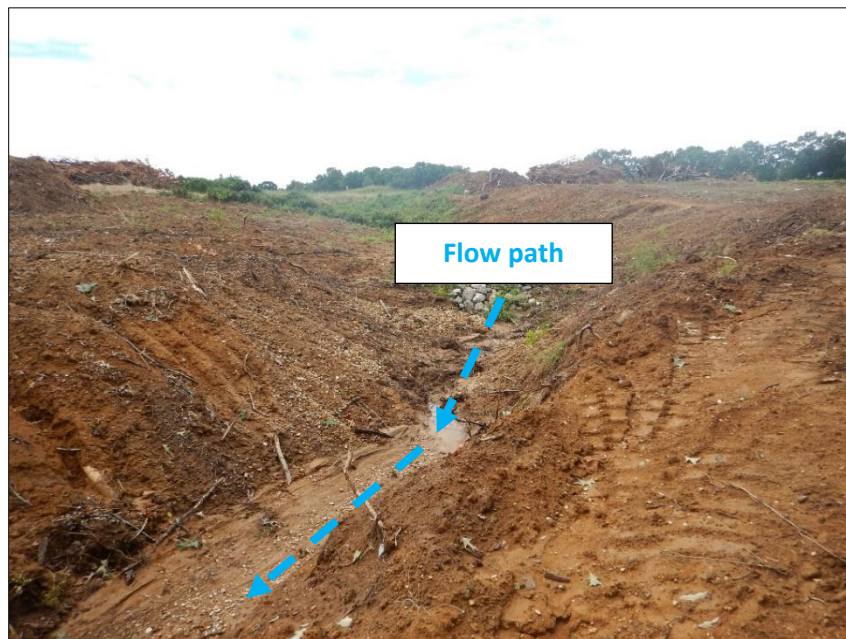
Photograph 46. Upgradient view of a concentrated flow path leading to an unidentified discharge point in the center of the Site. The slopes on either side of the concentrated flow path were unstabilized and eroded.
