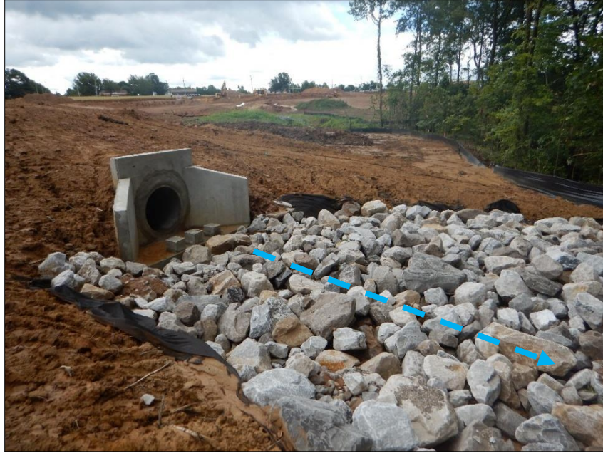
Photograph 27. View, facing south, of Outfall #7. Note the unstabilized slope upgradient of the outfall.
