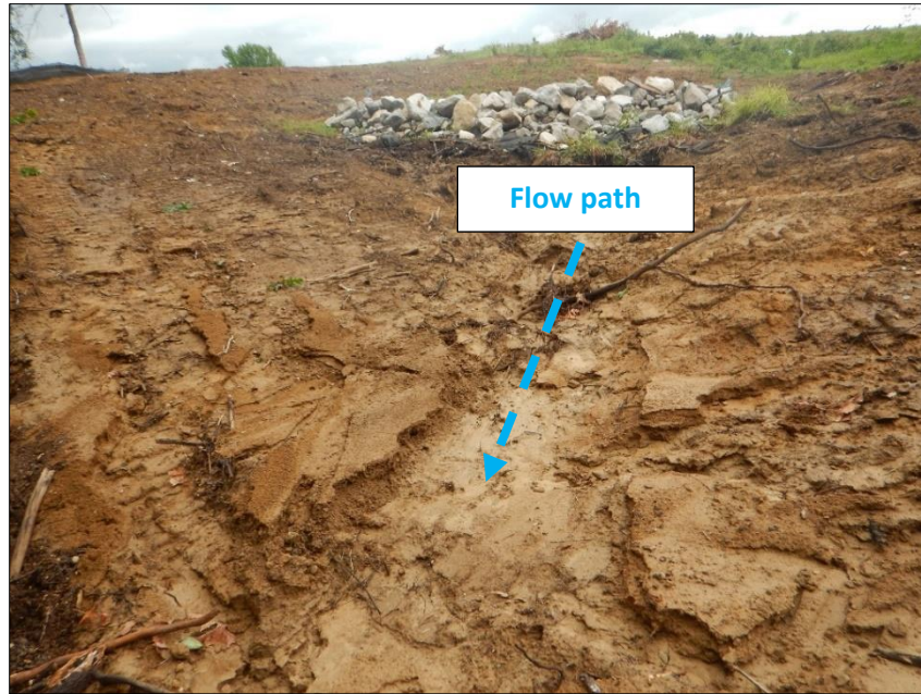
Photograph 39. Upgradient view of the flow path towards Outfall #16. The slopes were unstabilized and eroded. Stormwater and sediment had bypassed and undercut the check dam.
