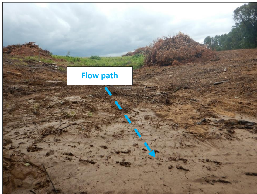
Photograph 34. Upgradient view of an unstabilized slope in the southern portion of the Site.
