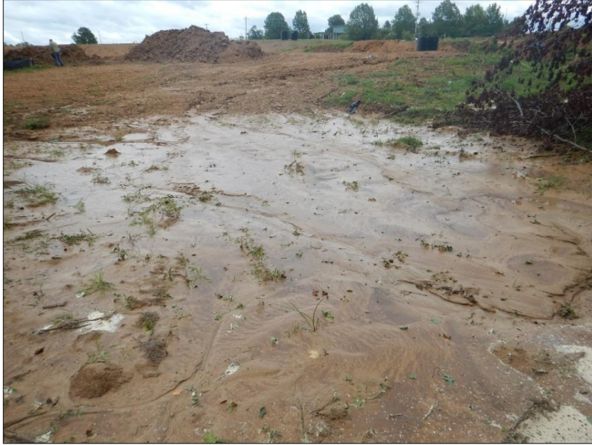
Photograph 65. View, facing northeast, of an unstabilized and eroded slope in the center of the Site.
