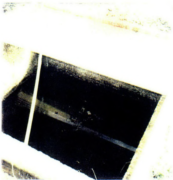
3 So Pit Dist Box 20 After Pumping 79
