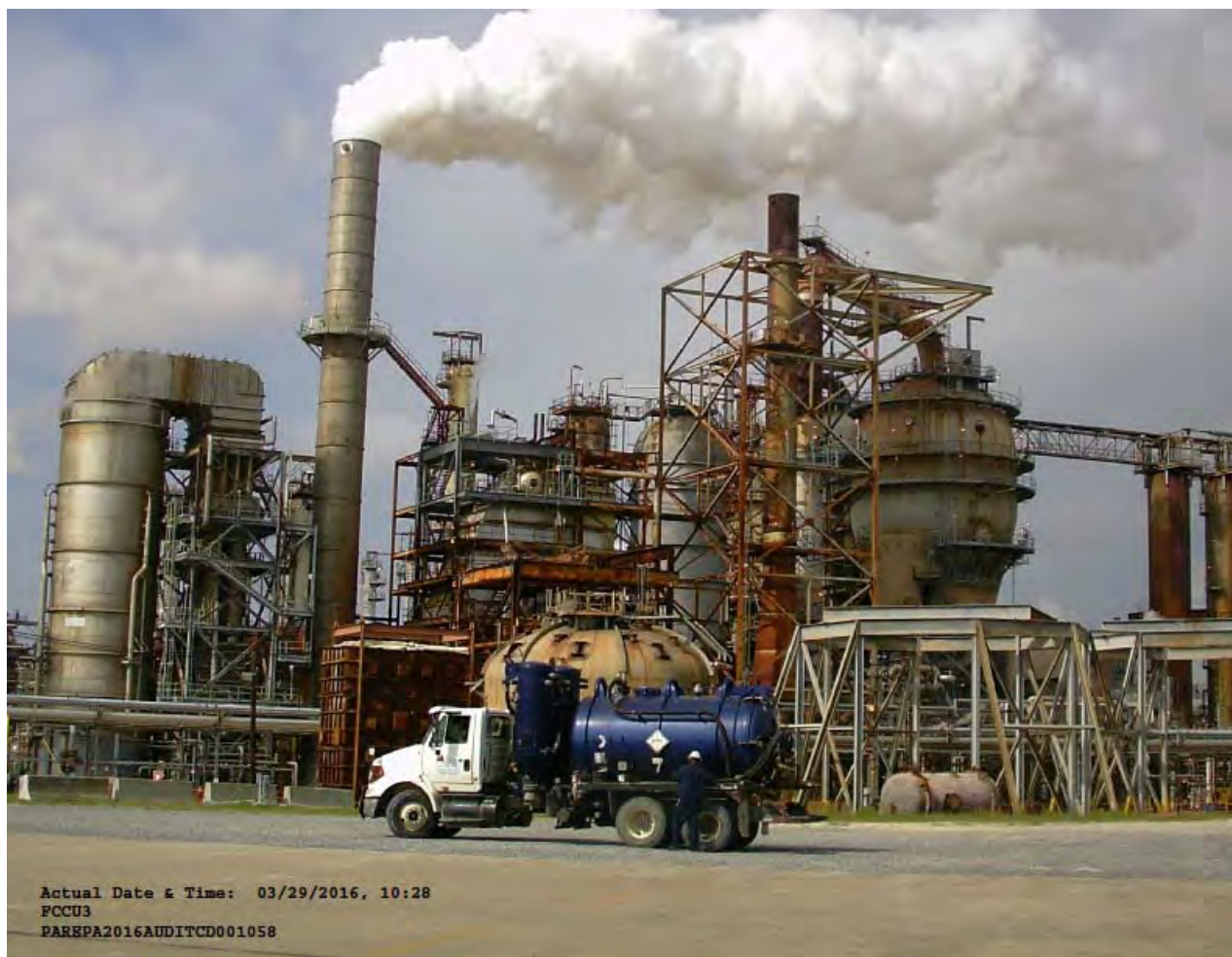
FCCU #3 Belco Wet Gas Scrubber
