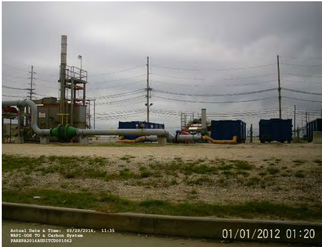
Waste Water Treatment Plant BWON Carbon Beds with shut down Thermal Oxidizer.
