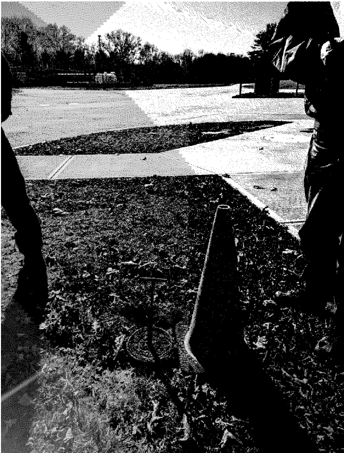
Photo 1 – Stormwater Cutoff Valve
