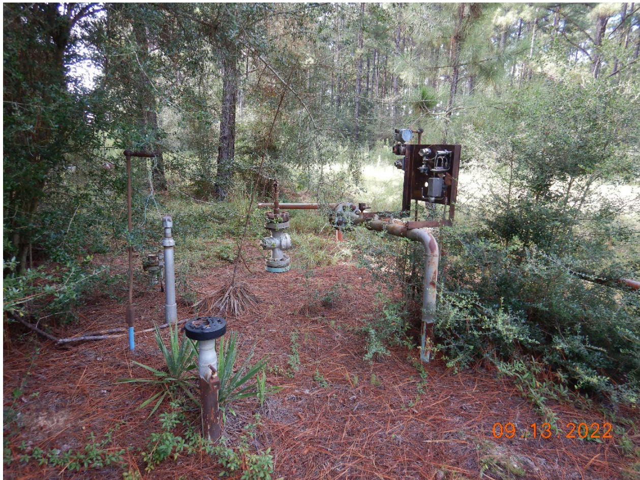
Photograph 6: Looking east, view of pressure relief system formerly attached to well, which used to convey unused nitrogen back to the Black Creek gas plant. It is disconnected and sealed off.
