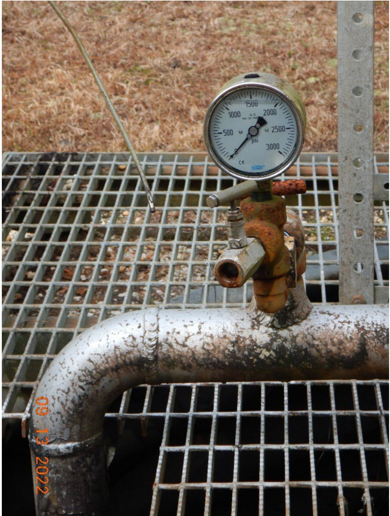
Photograph 3: Looking west, closeup view of production casing pressure gauge reading 0 psi.
