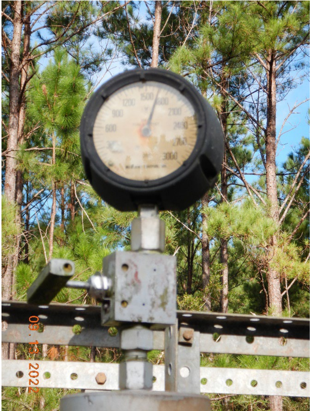
Photograph 4: Looking west, closeup view of internal pressure gauge reading 1,680 psi.
