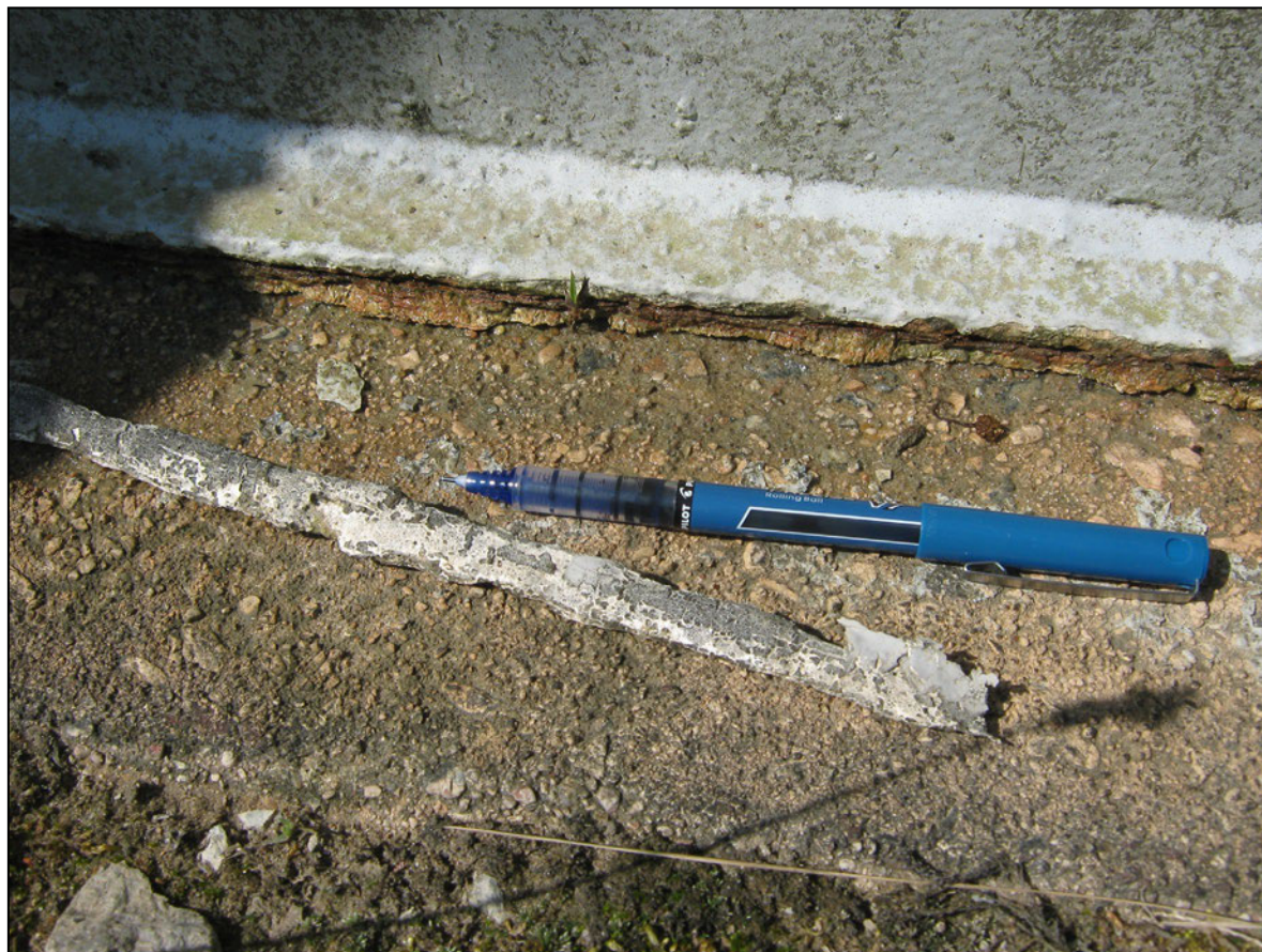
Photograph 6. Longhills Tank View of the grout and caulking seal at the base of the Longhills Tank that was weathered, peeling away, and cracked.
