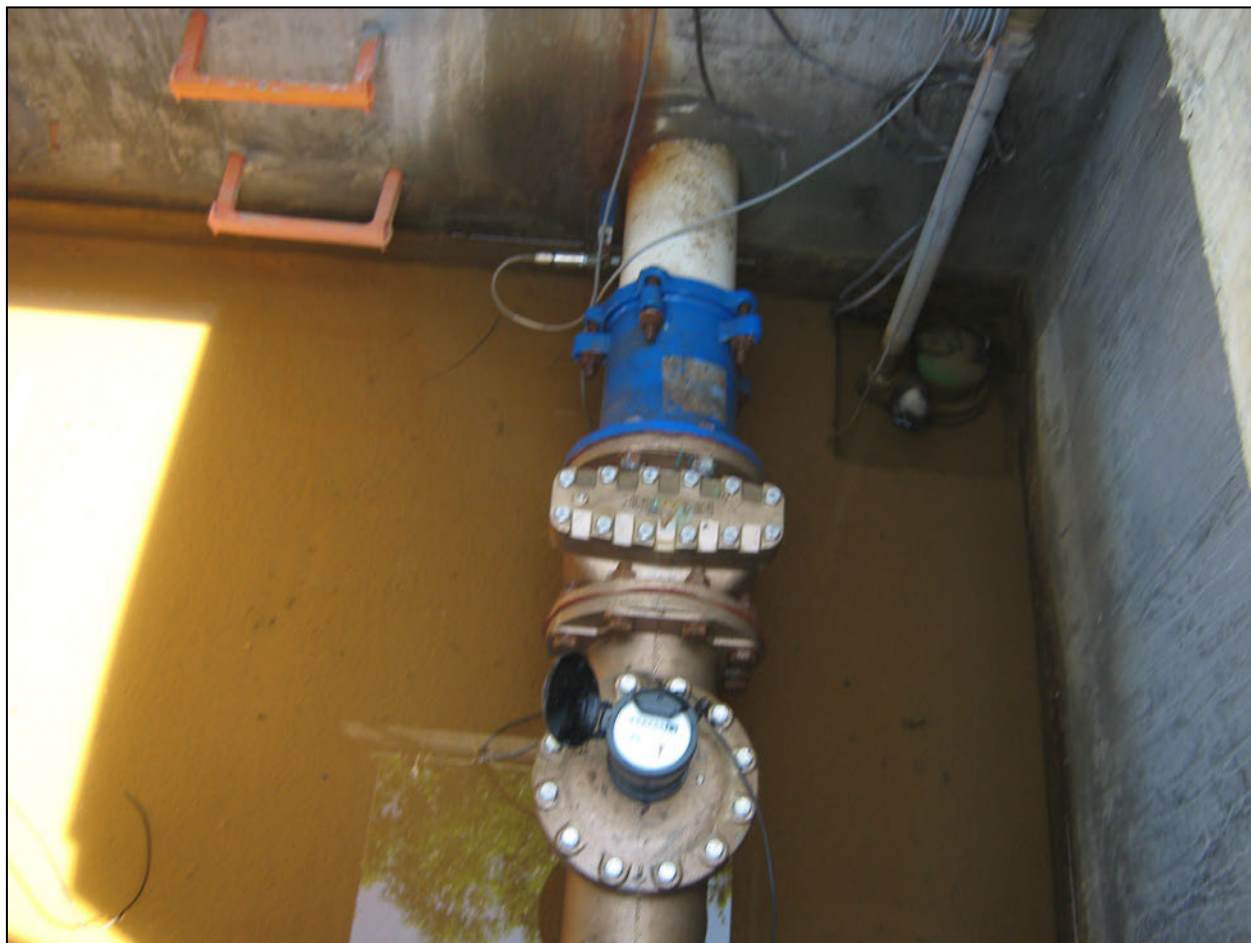
Photograph 12. Sparks CAW Master Meter View of light sediment on the pit floor and 1 foot of standing water which was near the submersible pump trigger point to operate.
