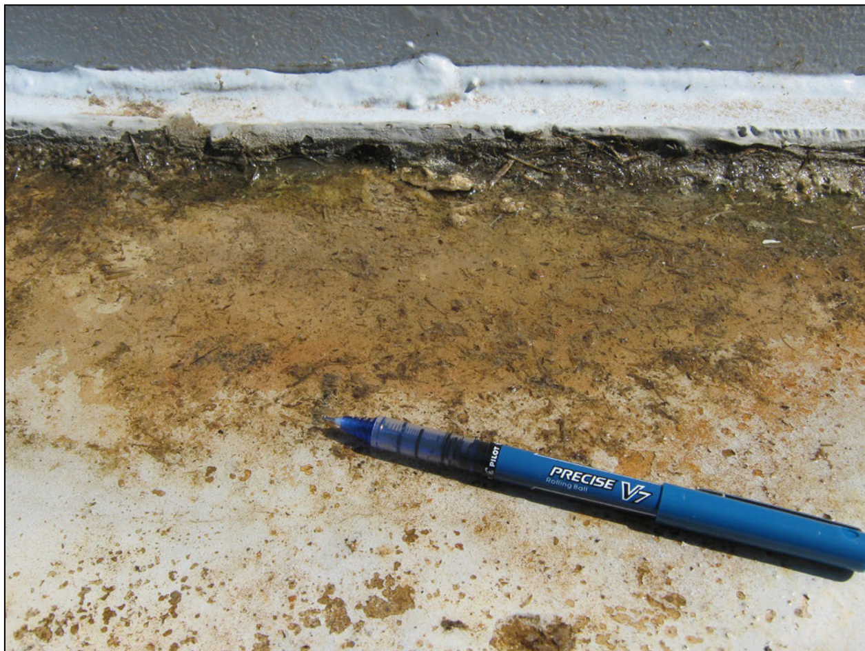
Photograph 15. Mulberry/Salem Tank View of apparent seepage from base of the tank, ponding onto the concrete base at the Mulberry/Salem Tank.
