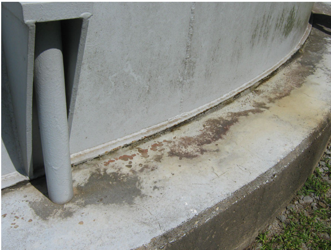
Photograph 16. Mulberry/Salem Tank Alternate view of apparent seepage from the base of the tank onto the concrete base at the Mulberry/Salem Tank.
