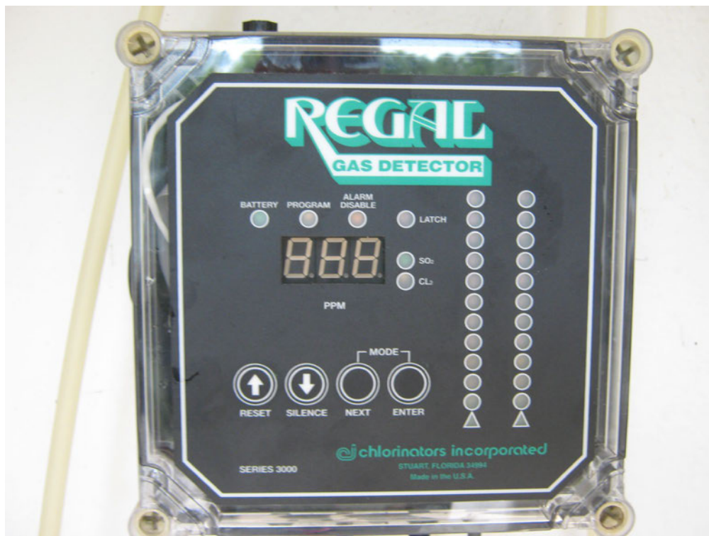
Photograph 17. Sparks Chlorine Booster Station View of the chlorine gas detector that was not functional at the Sparks Chlorine Booster Station.
