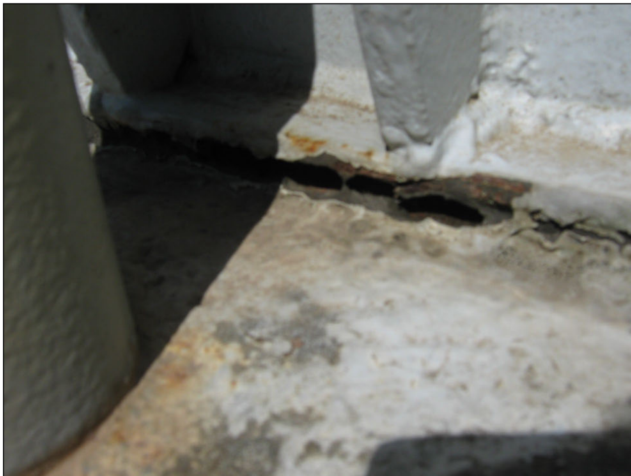
Photograph 11. Mulberry/Salem Tank View of a gap greater than \frac{1}{4} inch between the metal tank base and the concrete foundation of the Mulberry/Salem Tank.
