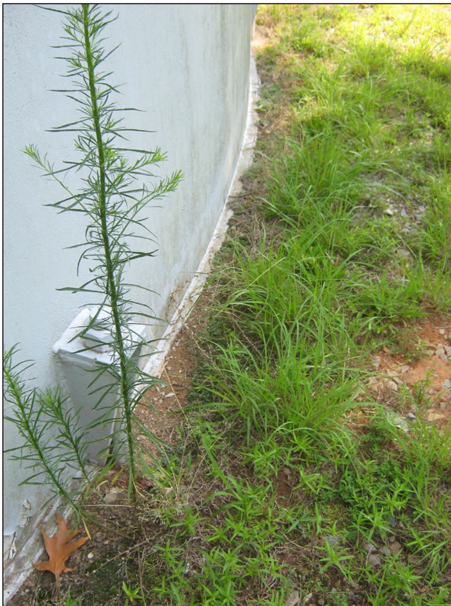
Photograph 5. Longhills Tank View of the concrete base of the Longhills Tank. The base was flush to ground level which allows water and sediment to come in contact with the metal tank base. The area was wet, indicating tank seepage from the base.
