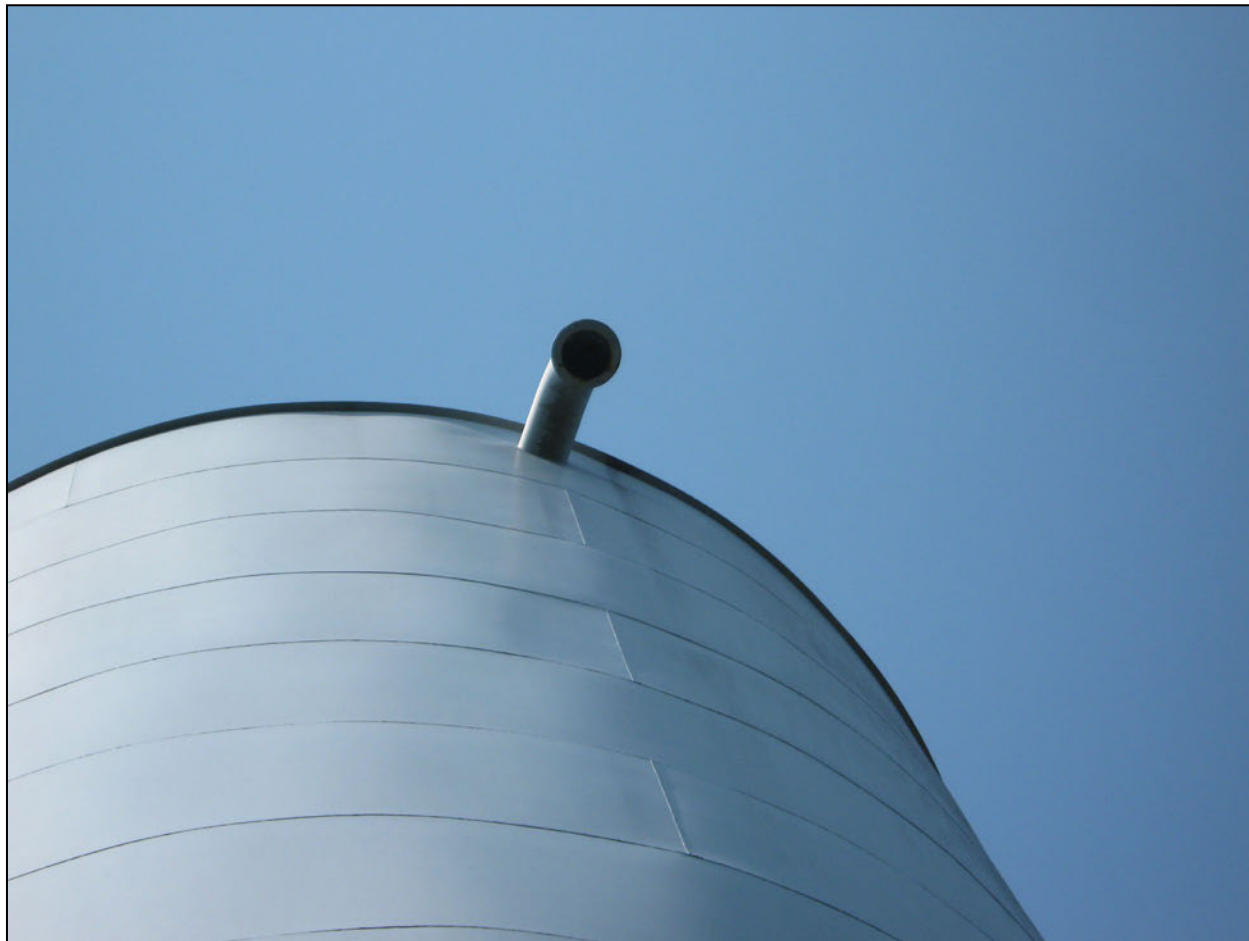
Photograph 10. Mulberry/Salem Tank View of the overflow of the Mulberry/Salem Tank that was downturned but did not extend to ground level. The overflow did not allow for evaluation for adequate screening.
