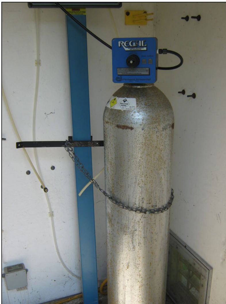
Photograph 14. Sparks Chlorine Booster Station View of one (1) 150 lb. chlorine gas cylinder that was in operation on a chlorine scale. The Regal chlorinator did not have a vent plumbed into the unit.
