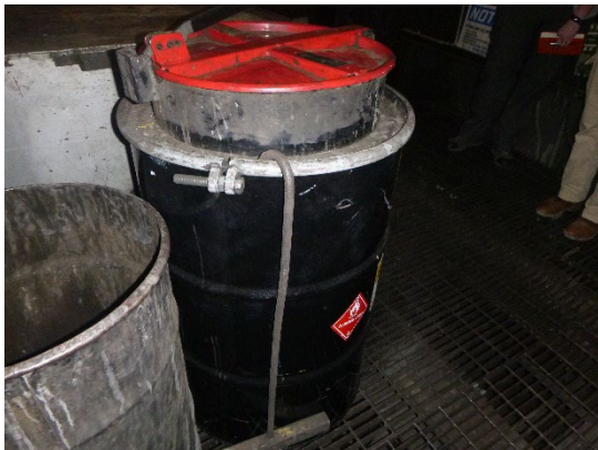
Photograph 3: Fill and Return Station SAA 55-gallon container.
