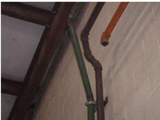
Photograph 5: Hazardous waste piping along Ceiling, which is untagged.
