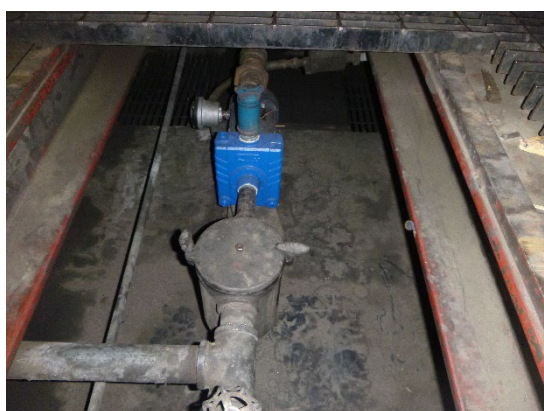
Photograph 9: Tagged filter and pump under Fill and Return Station.
