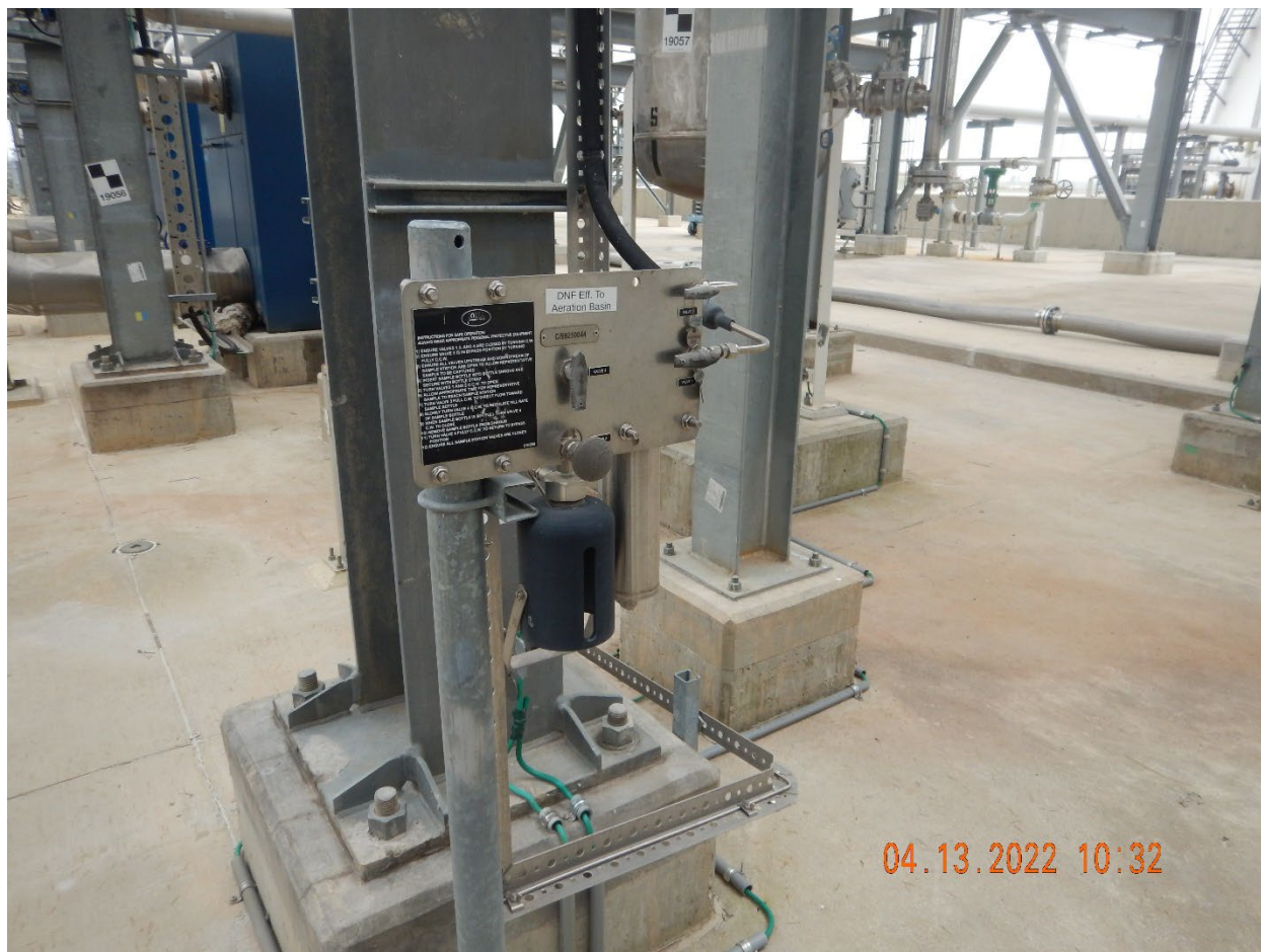
Inlet chemical oxygen demand sampling station for aeration basins.
