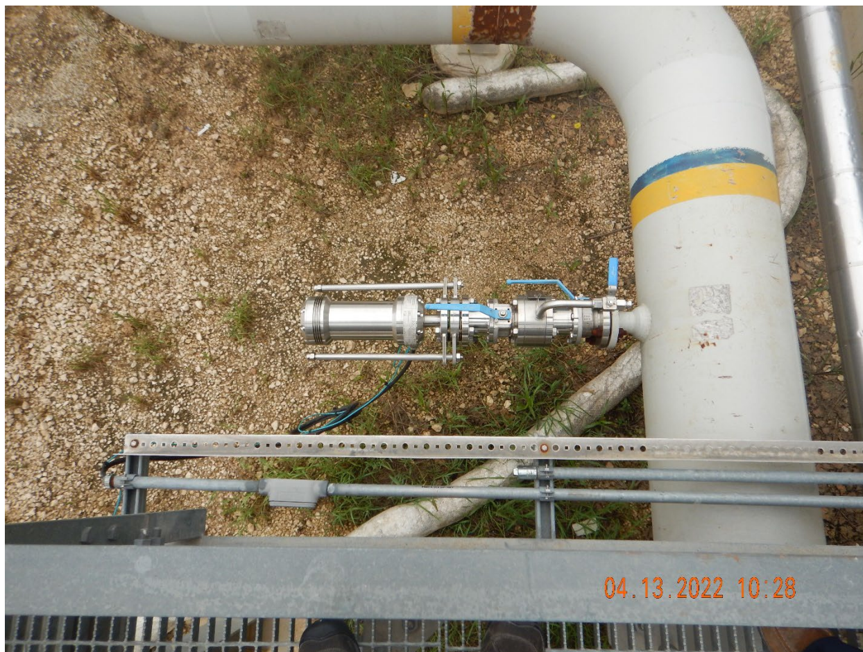
Oil analyzer for stormwater tank.
