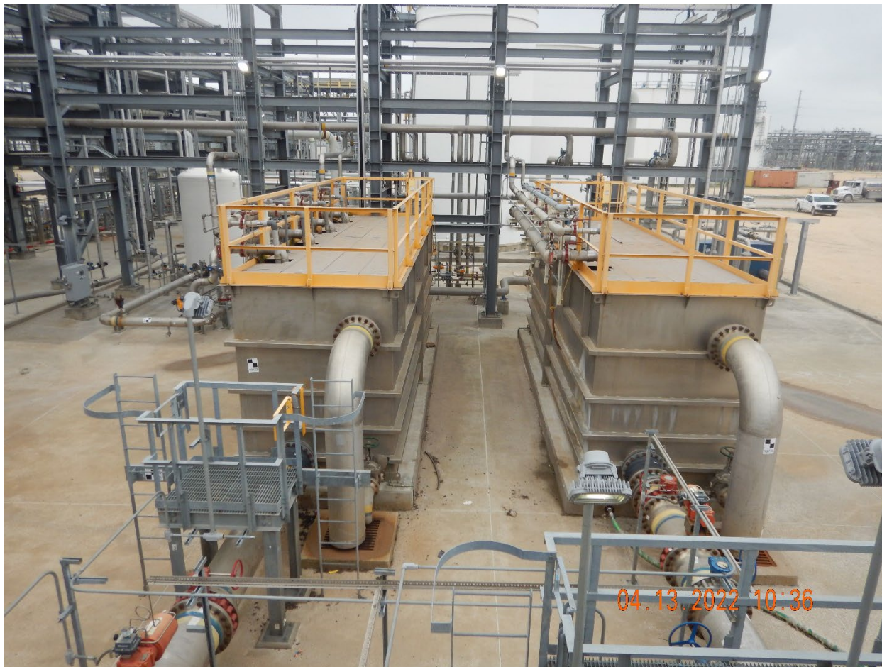
Membrane filter tanks.
