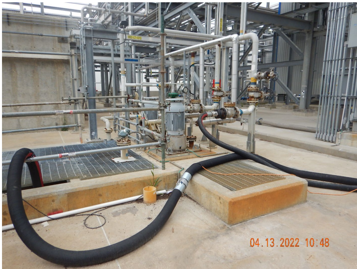
Biowater Sump Pump.
