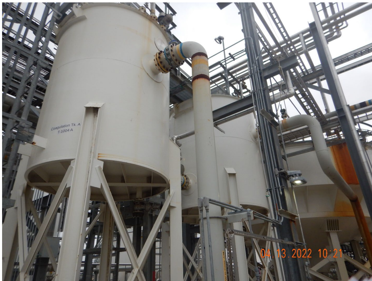
Coagulation, flocculation, and DNF 1 tanks for A train.
