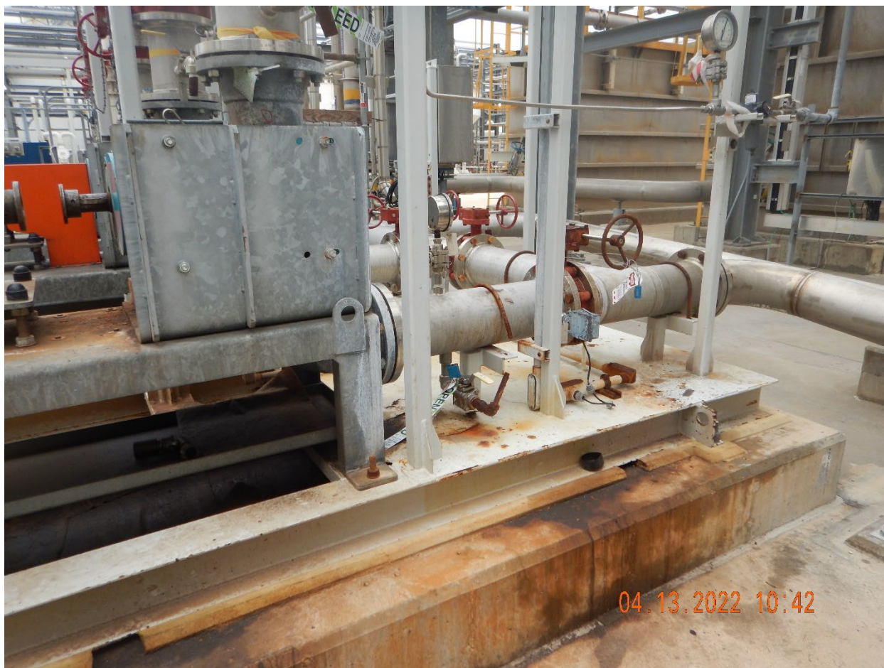
Chemical oxygen demand effluent sampling point post membrane tanks.
