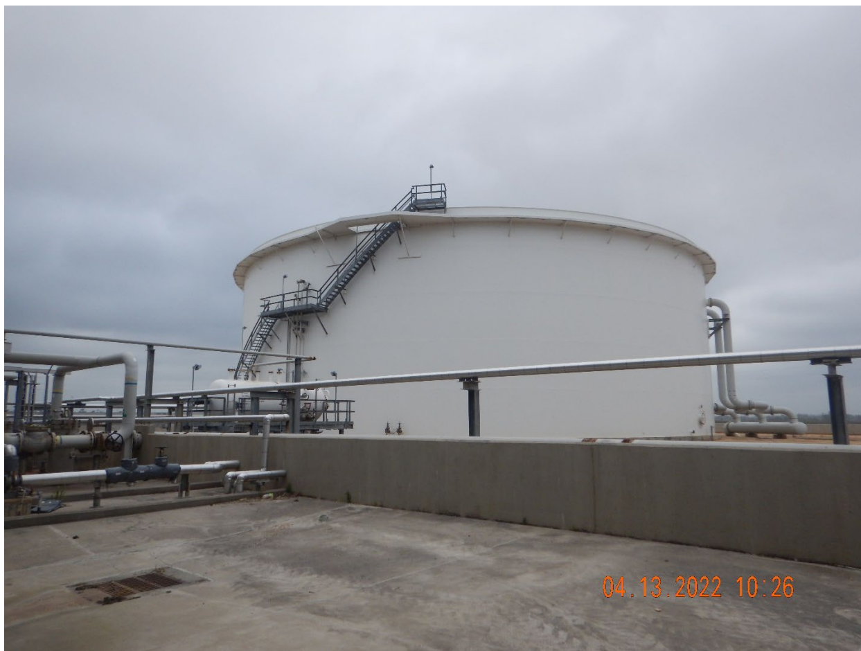
First Flush Tank.
