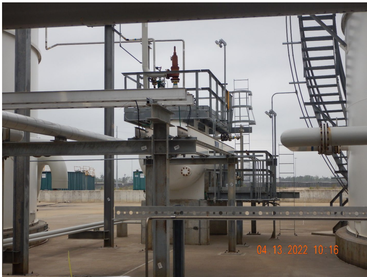
Oil skim drum next to EQ tanks.
