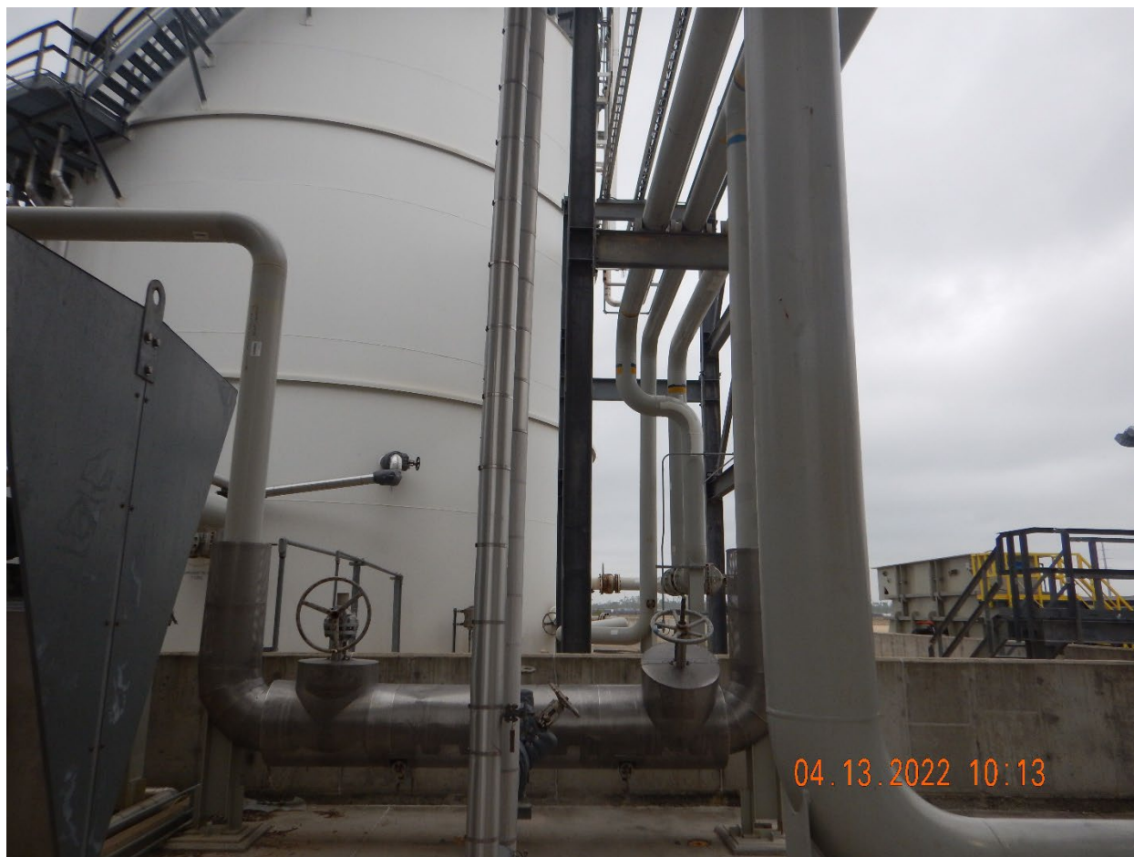
Pipe headers feeding to EQ 1 tank.
