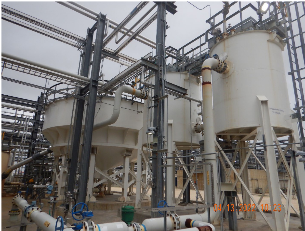
Coagulation, flocculation, and DNF 2 tanks for B train.
