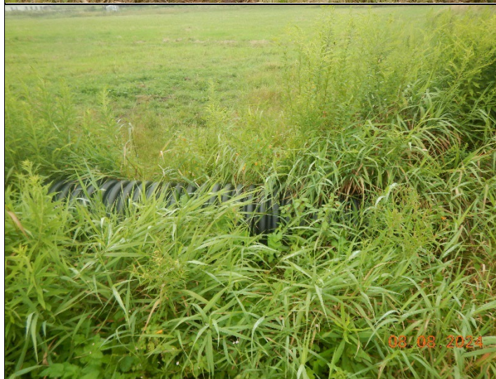
Hoopes Property Date: 8 August 2024 Photo ID: DSCN5563.JPG Photo taken by: Laura Mathew Notes: Unused drain observed in the vegetation during walkthrough.
